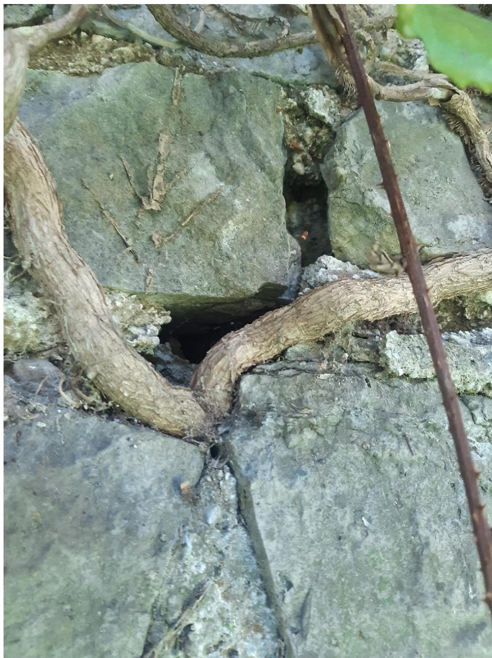
Plate 3: An example of how the ivy and vines are penetrating in between the stonework of the wall
