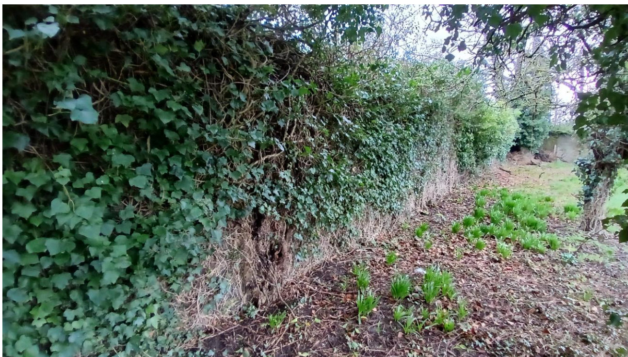
Figure 5: Extensive Internal Ivy and vines
