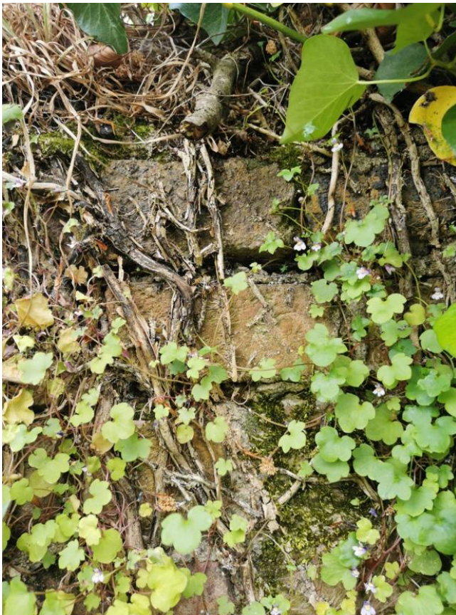
Plate 4 Examples of a cracks in the stonework and ivy penetrating into this crack.
