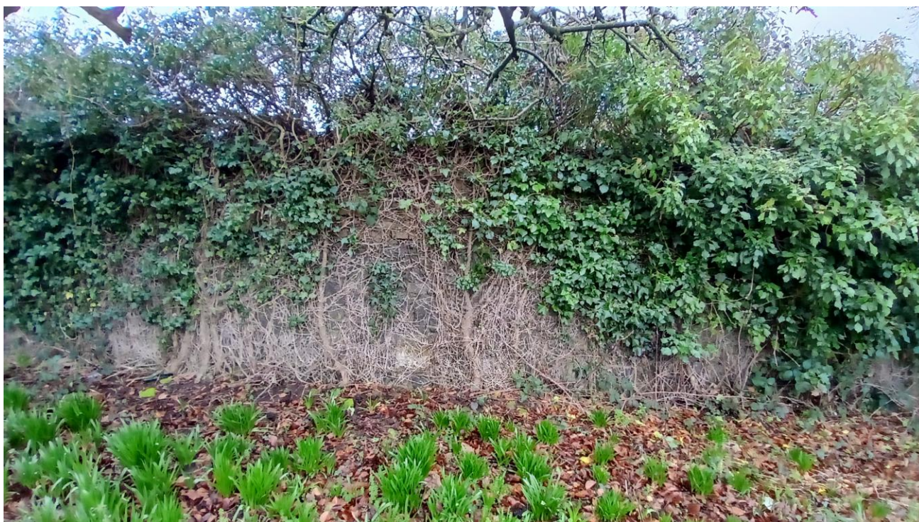
Figure 7: Extensive Internal Ivy and vines
