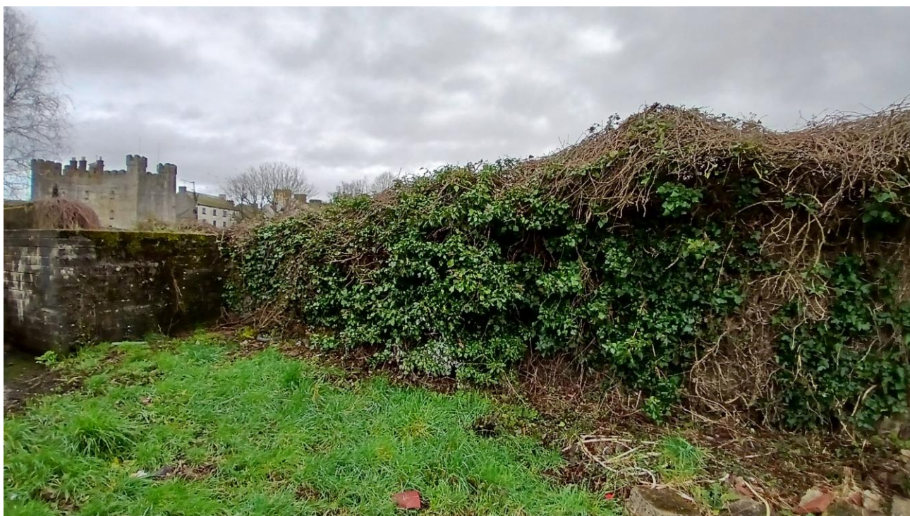
Figure 3: Extensive Internal Ivy and vines
