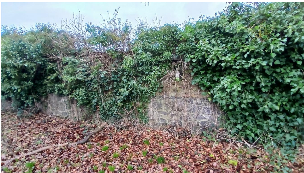
Figure 6: Extensive Internal Ivy and vines
