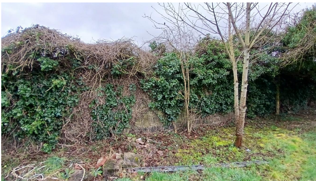
Figure 4: Extensive Internal Ivy and vines
