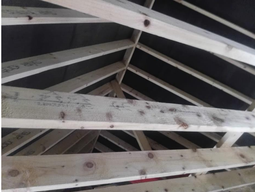
17 th Dec 2025 Bitumen felt on Stable B with loft to be closed up with access for inspection. Recommended additional horizontal lats across the apex to increase roosting options
