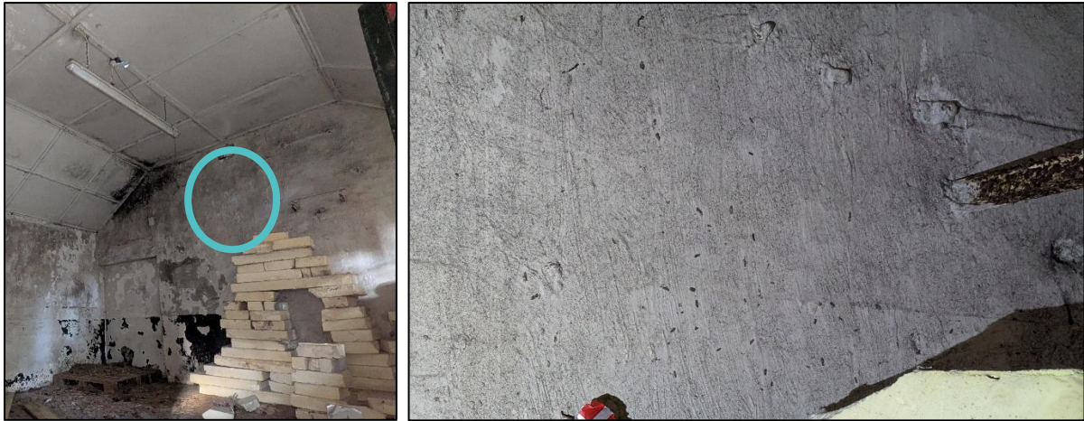
Plate 3-4. Bat droppings recorded within Building B1.
