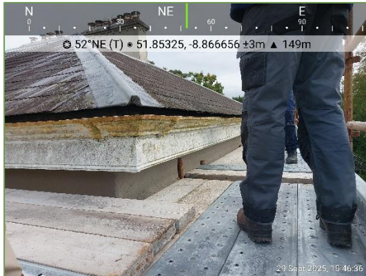
Plate 3.5 View of southwest corner of roof. Note gap between gutters and slate.
