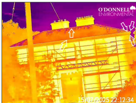
Plate 2.1 Thermal perspective overlooking the west aspect of Lissardagh Main House. Emergence points are highlighted with white arrows.
