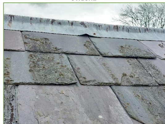
Plate 3.8 Example of buckled lead ridges, presenting suitable access/egress throughout.
