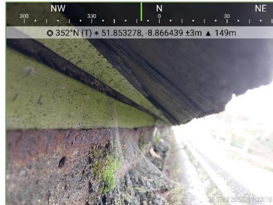
Plate 3.6 Detailed view of gap between gutters and slate on southwest corner, droppings evident.
