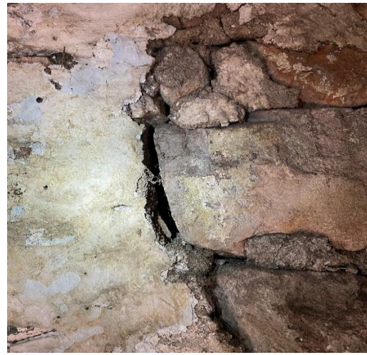
Plate 5-8 Large crack in interior stonework
