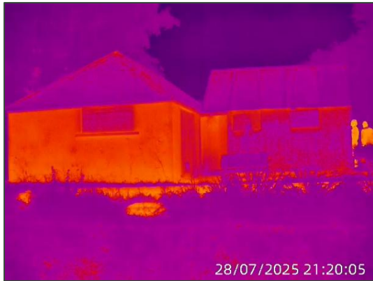
Plate 2.1 Thermal perspective overlooking the front/western aspect of the derelict cottage (S01) with surveyors in background.
