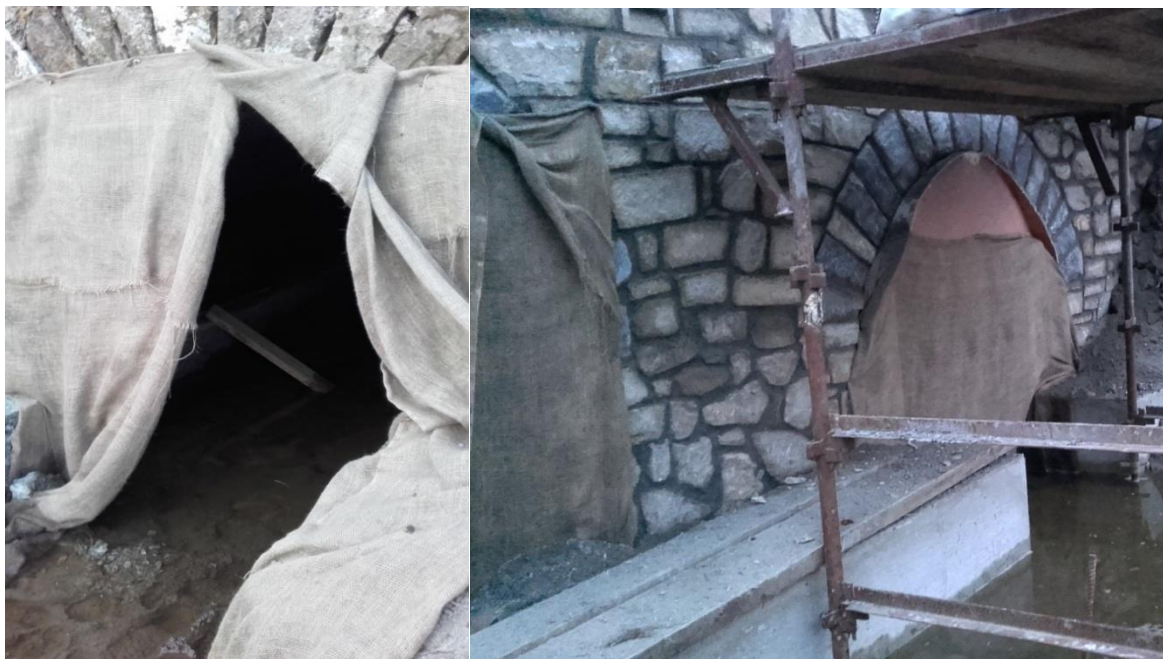
Plates 6a, b Example of hessian material curtains for sealing bridge arches
