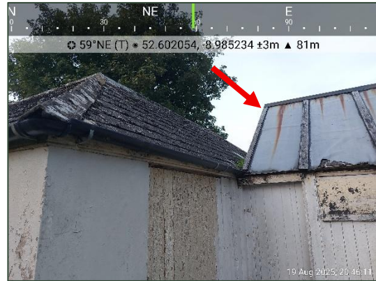
Plate 3.2 Close-up view of disused cottage, showing two distinct roofing styles. External view of access/egress near interior bat droppings shown in red arrow.
