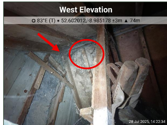
Plate 3.6 Location of bat droppings (red circle) and access/egress point (red arrow) in roof apex of southern section.
