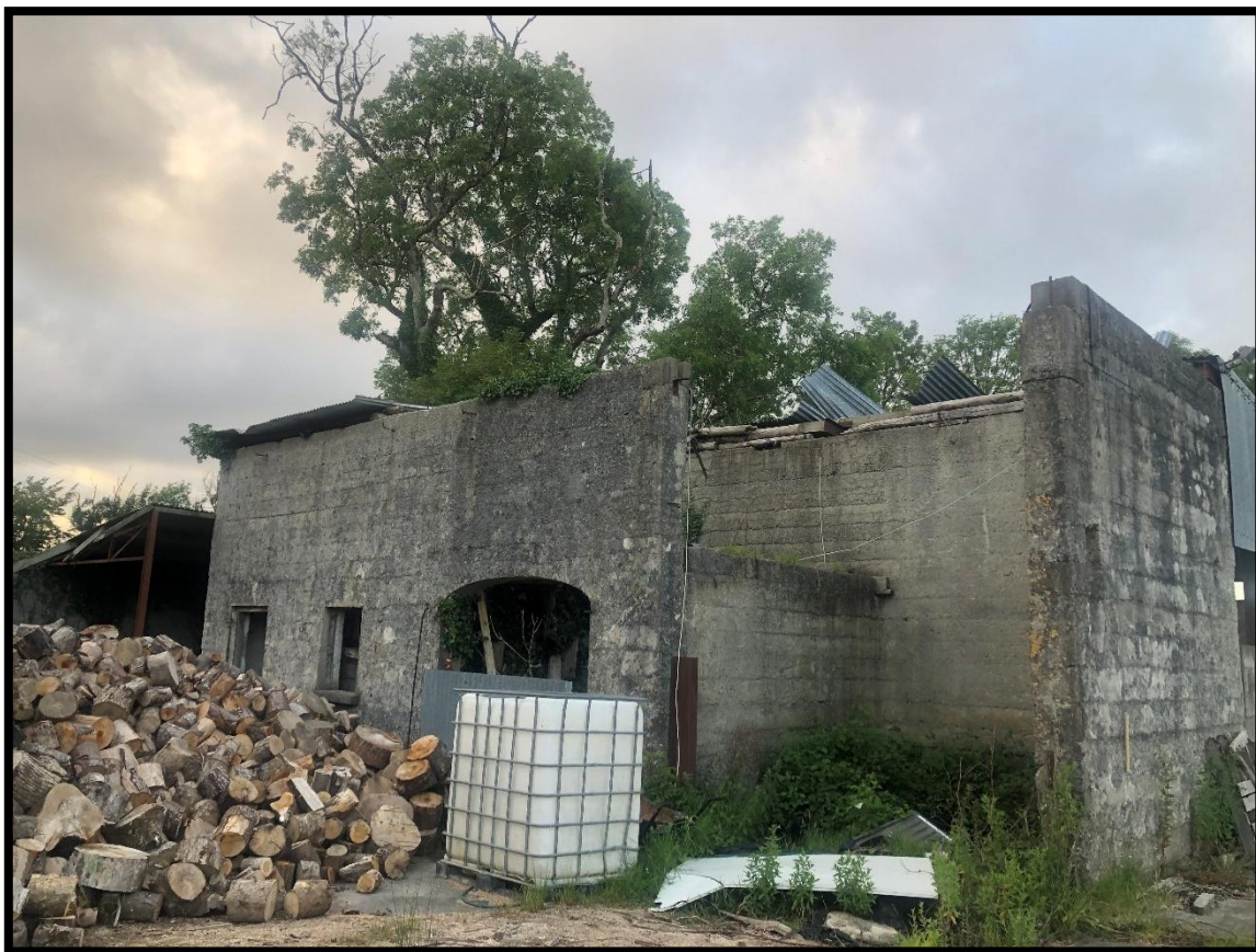
Plate 5.5 Shed to the north of the derelict house. Note unstable structure of roof unsuitable for roosting bats
