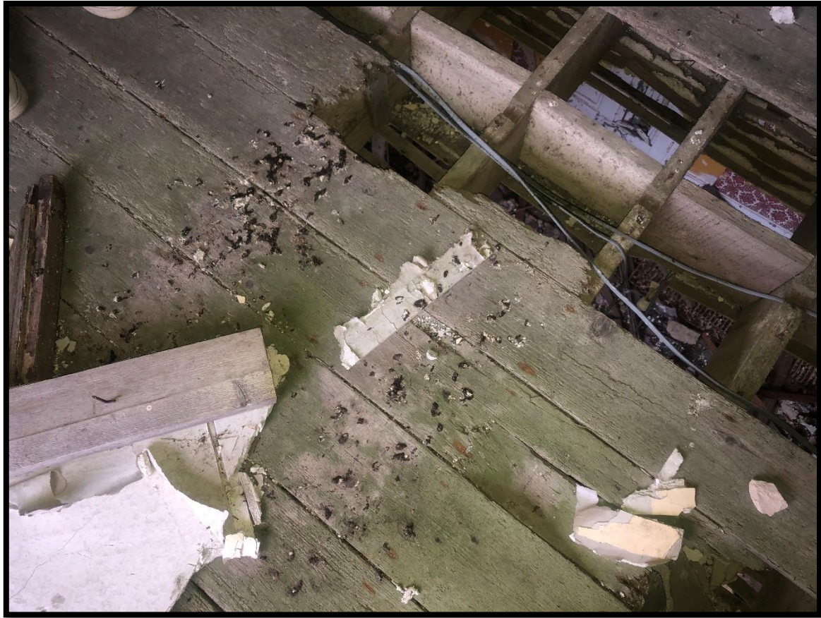
Plate 5.8 Image of bat dropping noted on the first-floor room to the east of the derelict house. Note the gaps in the floor to the ground floor
