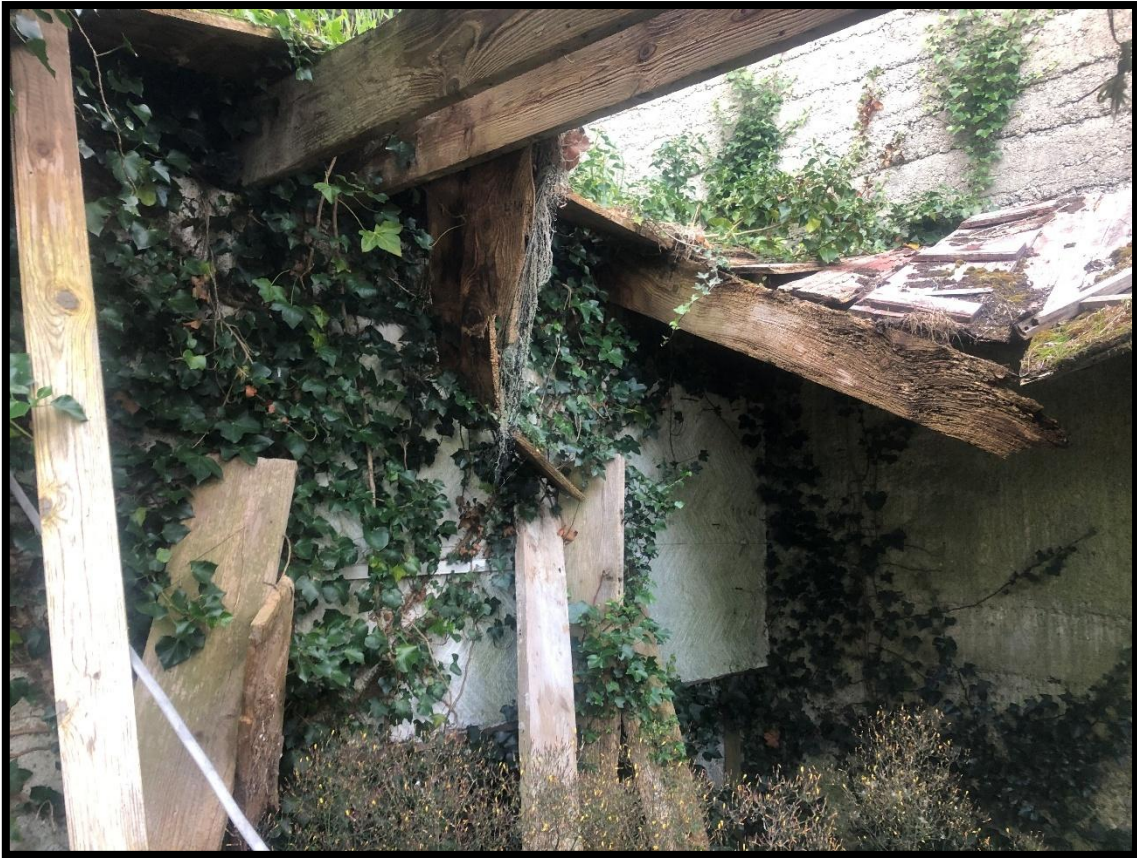
Plate 5.6 Interior of shed to the north of the site. Note dense ivy on walls and overgrown vegetation on the floor
