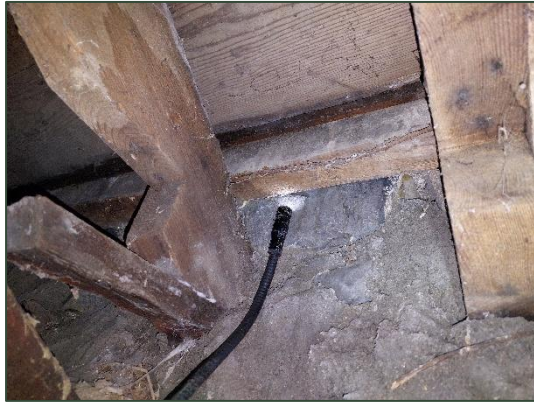
Plate 3.6 View of example crevice between roof structure sarking and wall plate.
