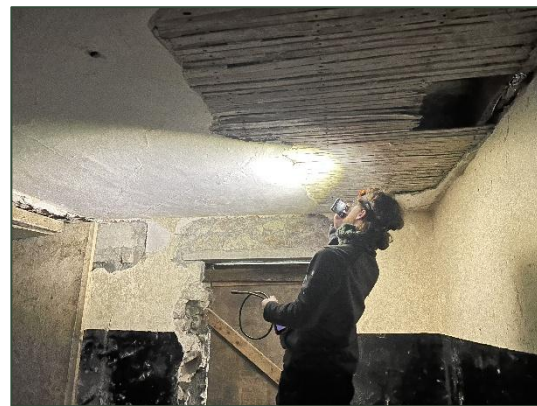
Plate 3.15 Surveyor inspecting void above small accumulation of droppings.
