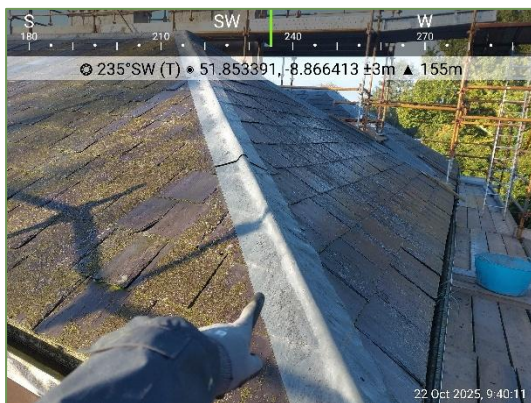
Plate 3.7 Example view of damaged lead. Presents voids underneath and above slates, with droppings and individual bats recorded underneath.
