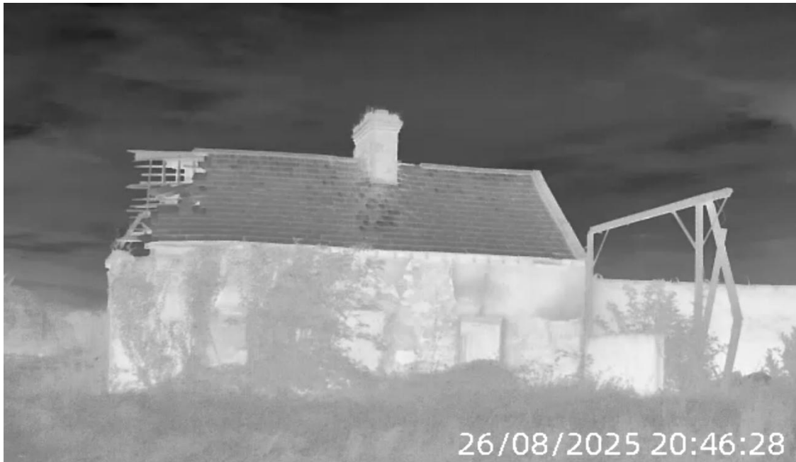
Plate 5-3: Canon Infrared view of derelict dwelling - Survey 1 (1b)
