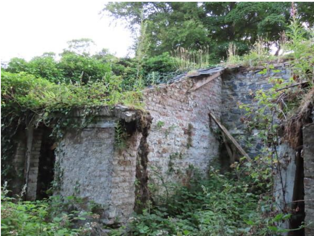
Figure 5. Ruined outbuilding with collapsed roof
