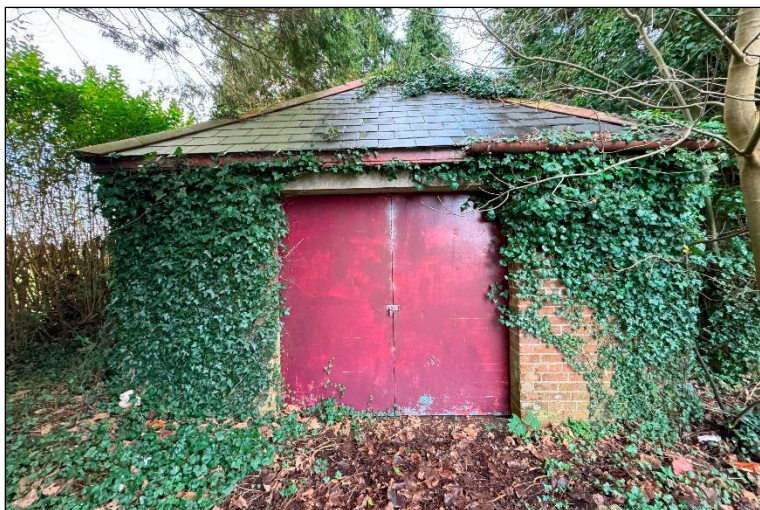
Plate 7 Small storage building covered in ivy which will be demolished (winter survey).
