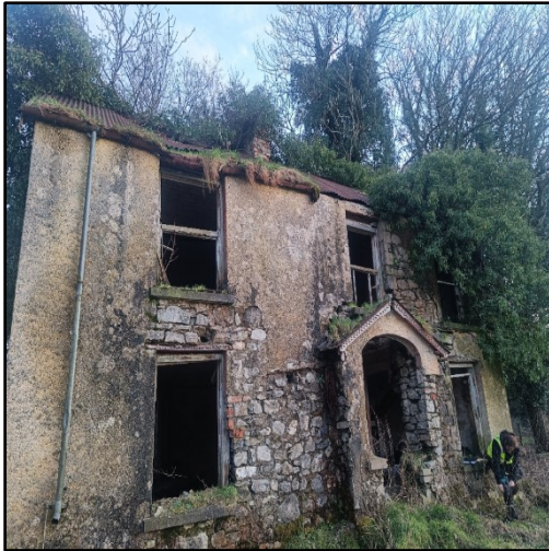
Plate 3-11. Derelict two-story house with collapsing damaged roof.
