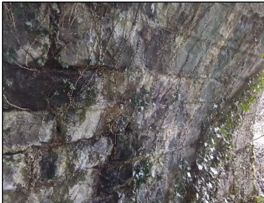
Plate 3-3 Stone blocks are sealed with cement with a small amount of ivy growth, some water leakage through the stonework.
