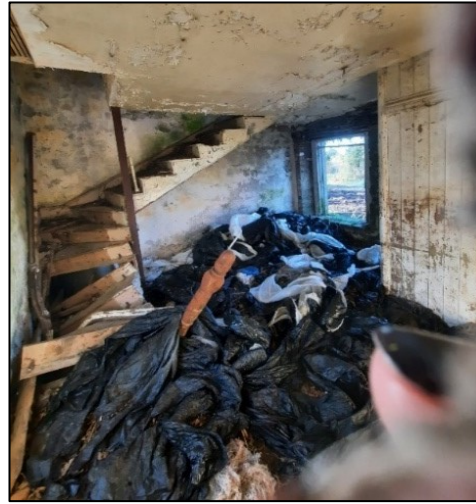
Plate 3-12. Interior view with partially collapsed staircase.
