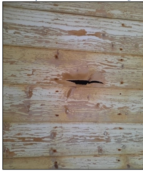
Plate 3-16 Gap in Wooden ceiling showing oil stains and missing paint showing a potential 'entry point'.
