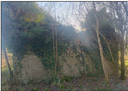
Plate 3-29 Northern Aspect showing brick wall, ivy growth and missing roof.
