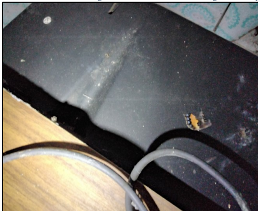
Plate 3-34 Butterfly feeding remains, likely from rats found within the building.
