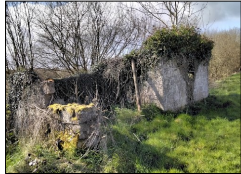
Plate 3-28 Derelict shed with missing roof.
