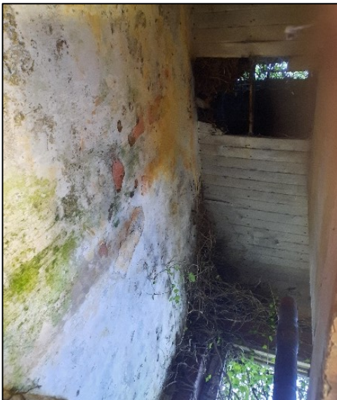
Plate 3-13 View of first floor ceiling with damage visible.
