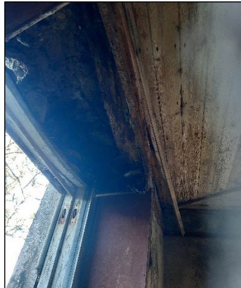
Plate 3-14 Gap between window frame and ceiling.
