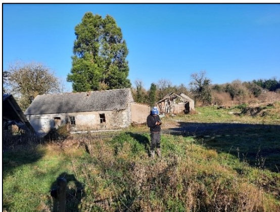
Plate 3-21 Northern Cottage B1 with missing windows, open doors and missing and damaged slates.
