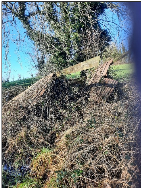
Plate 3-25 Collapsed shed roof with corrugated iron roof and briars covering the structure.
