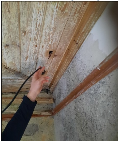
Plate 3-15 Endoscope use on the small gap in ceiling.
