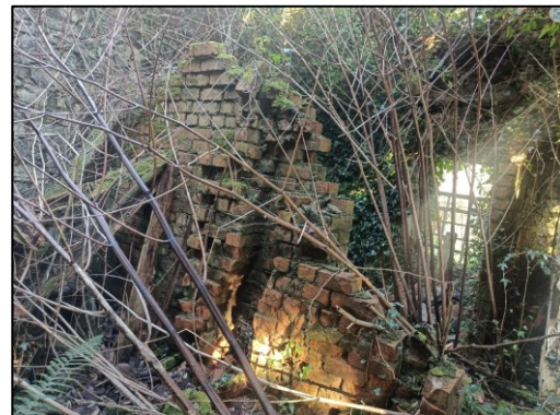
Plate 3-30 Internal view of the structure, with ivy growth and many gaps and cracks.
