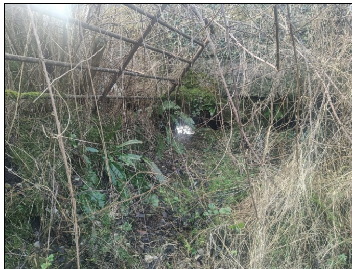
Plate 3-10 Bridge 3 Concrete pipe habitat, briar and scrub growth, the no water contained in the drain base.
