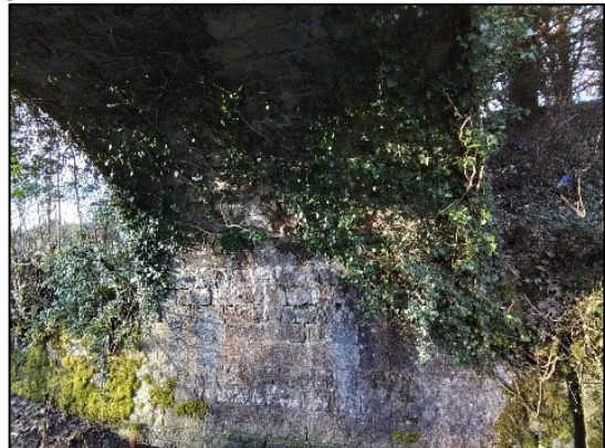
Plate 3-4 Ivy growth on the underside of the bridge.
