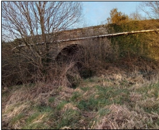
Plate 3-7. Bridge 2 Stone masonry bridge with ivy cover and a pipe along one side.
