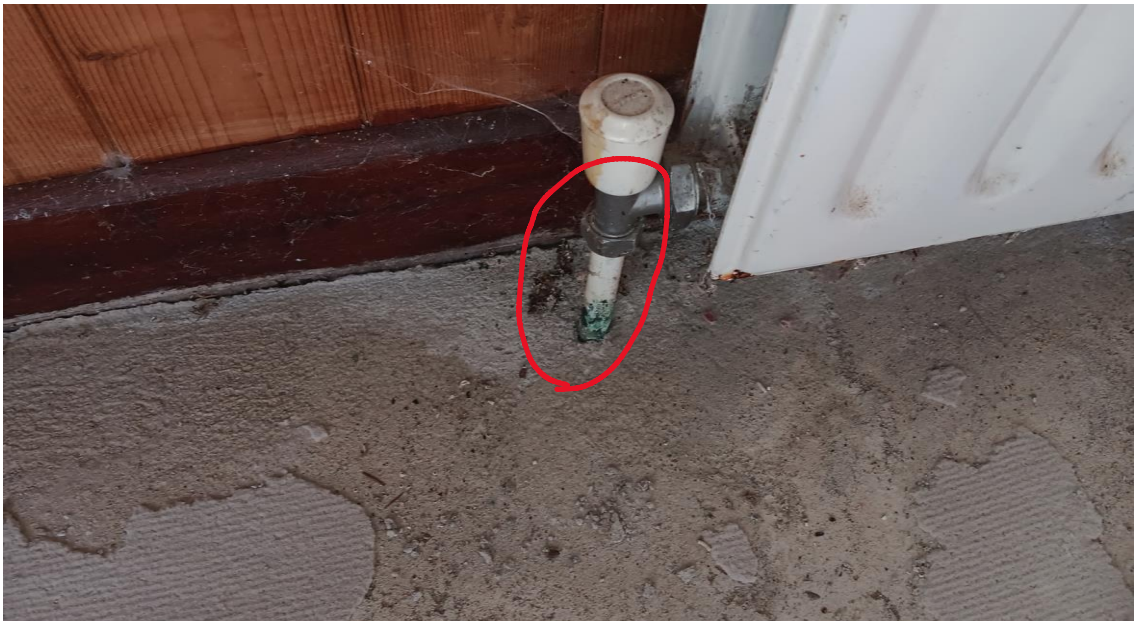
Photo 41 – signs of corrosion at copper pipe. House approx 50 years old – typical age for copper radiator pipes to leak (pitting corrosion)
