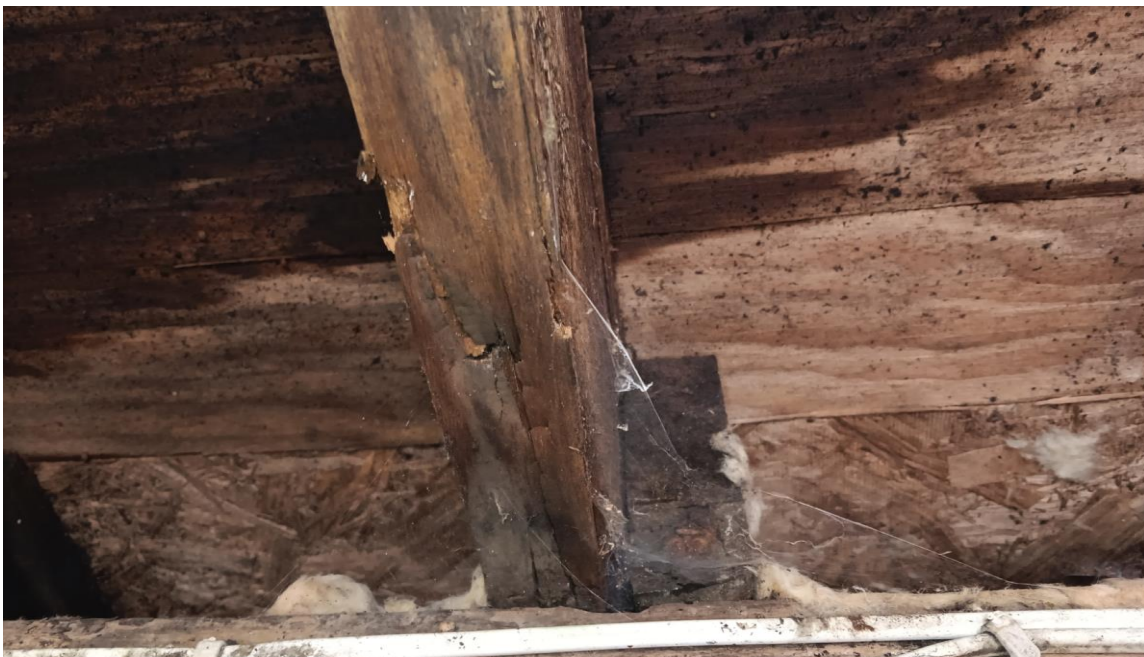
Photo 4 – Rotten and failed flat roof joist. Timber ‘split’ and degraded throughout. Wet rot visible
