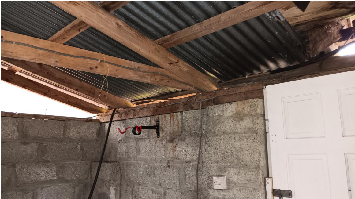
Photo 49 Structural inadequacy of garage roof; Purlins undersized, insufficient rafters, rot presenting at wall plate, no ‘holding down’ straps present – Entire garage roof to be replaced. (note: all electrical wiring, sockets etc are not IP rated, for semi- exposed /damp area, and should be replaced – all wiring to current IEE standards).
