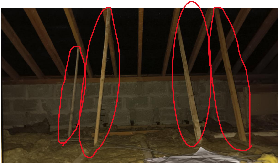
Photo 26– Struts provided to support roof (struts measure 50mm x 50mm and 100mm x 50) totally structurally inadequate to support roof. Bowing observed on rafters. Overall sagging noted externally on this roof (see photo no 30 ) due to inadequate structural support. No ‘holding down’ straps present. Overall roof is structurally weak.
