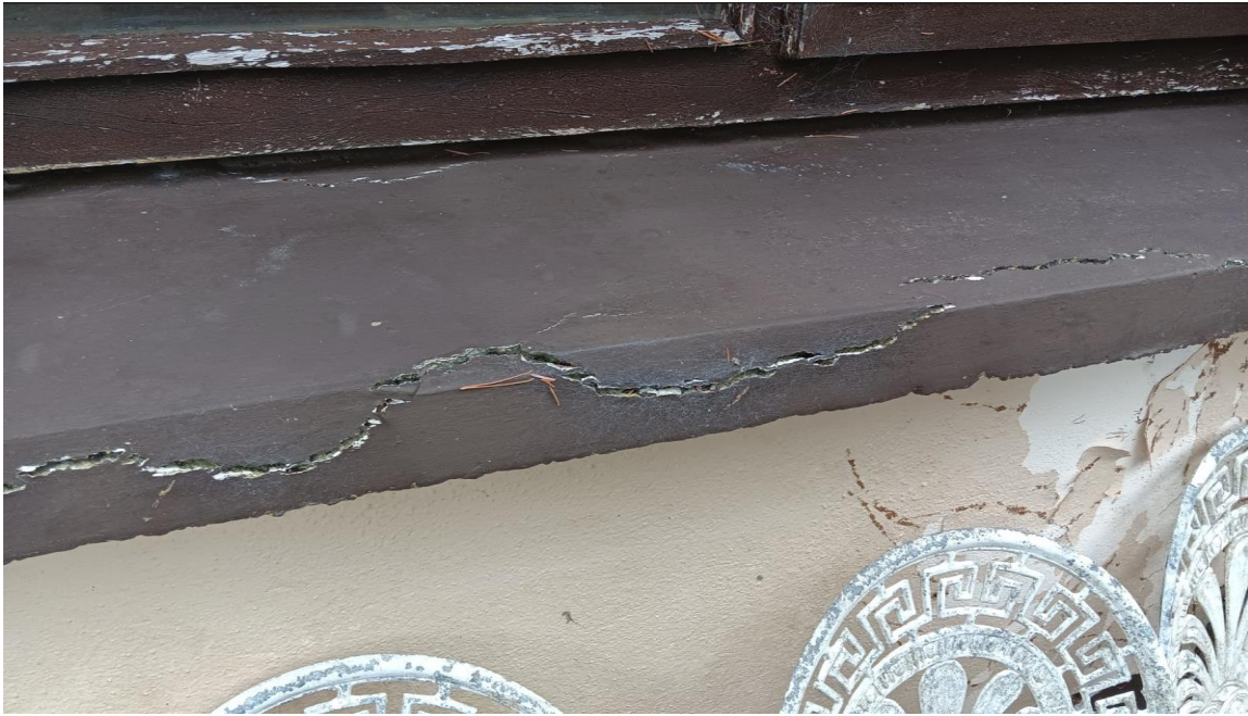
Photo 34 damage to window cill spalling / cracking – to be rectified.
