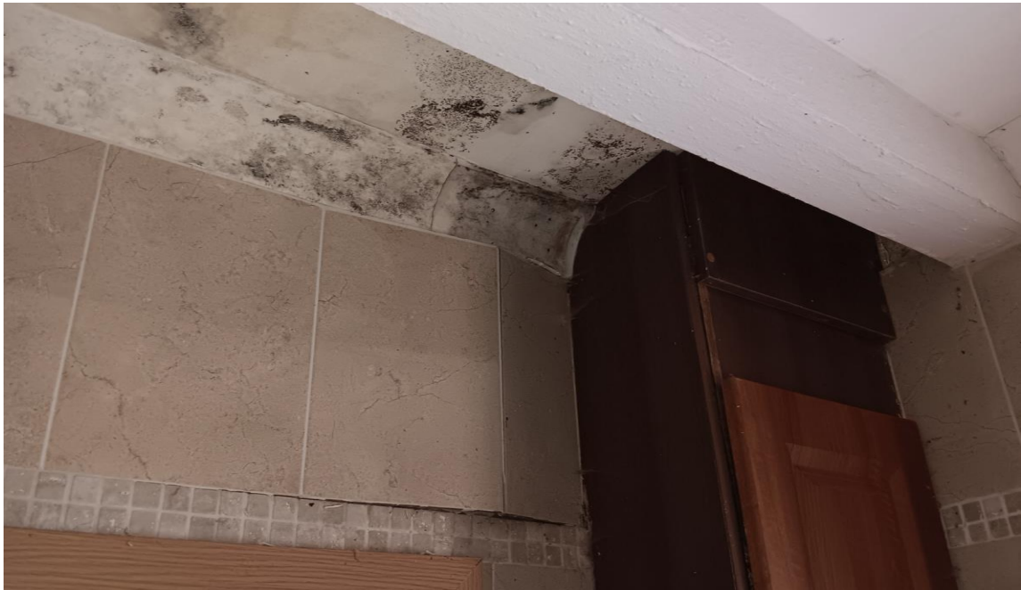
Photo 24 -severe mould growth on ceiling , due to defective roof. Severly damp walls present
