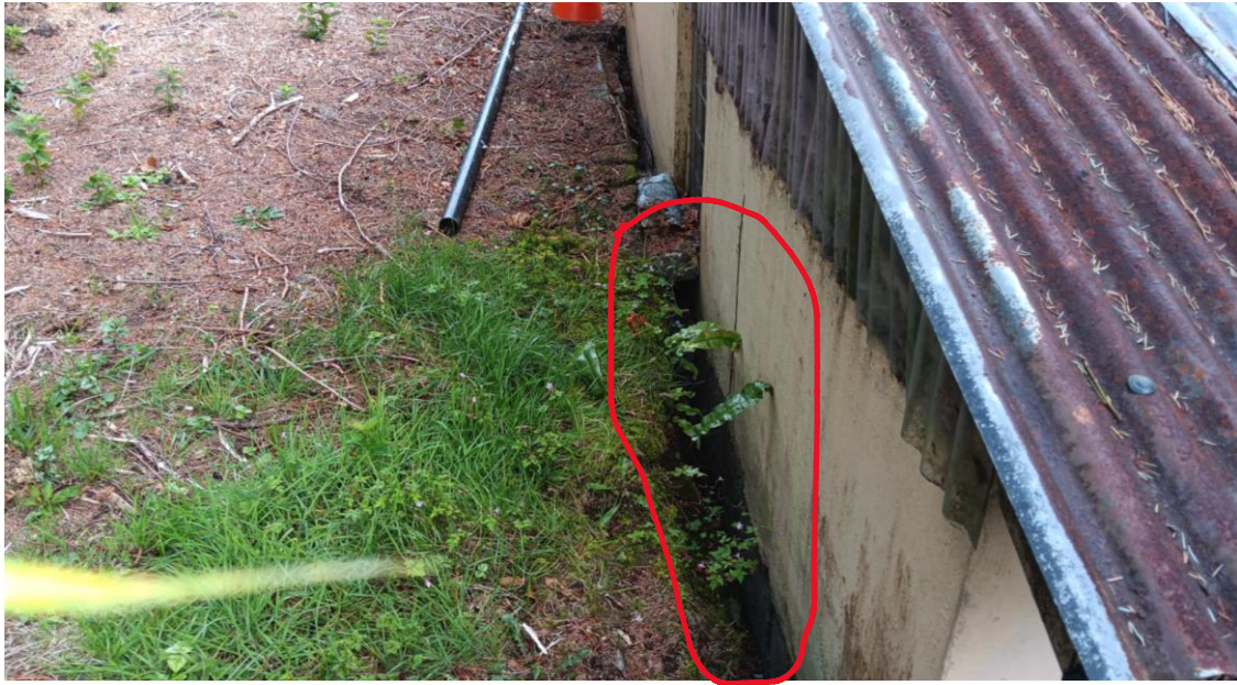
Photo 52 – Garage wall is not designed as a retaining wall - possibility of potential collapse of ground – which would compromise the wall structure.
