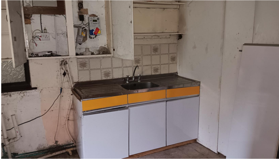
Photo 22– Faulty electrical wiring
