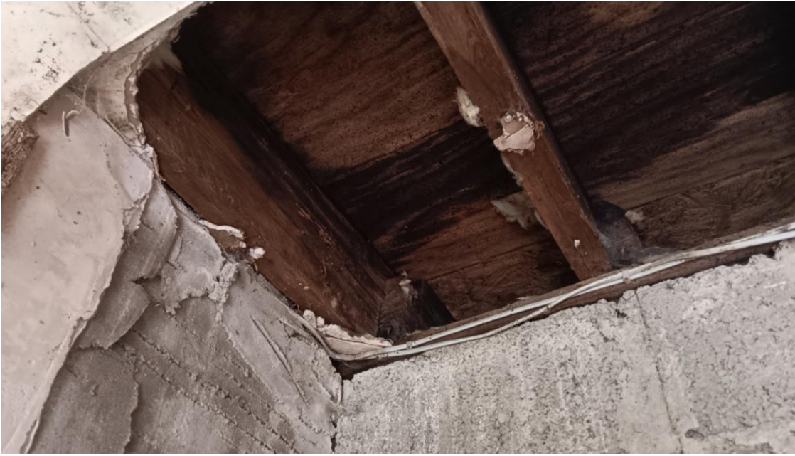
Photo 5 – Visible damp on underside of roof deck – general overall fail of flat roof.
