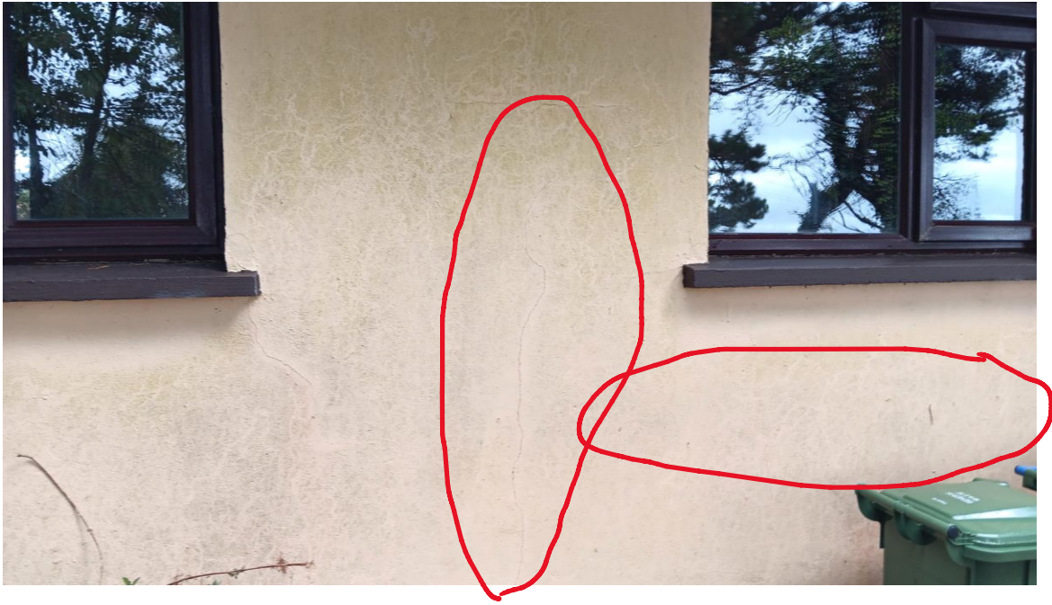
Photo 32 Slight cracking in wall (vertical and horizontal)
