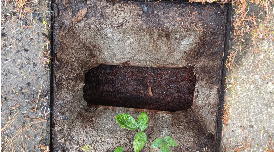
Photo 44 Drainage manhole inadequate - Very poor Construction detail. Cover and frame structurally failed.
