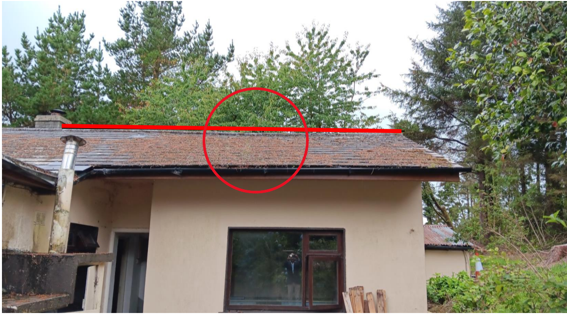
Photo 30 'bow' in roof, due to inadequate structural roof support (see photo no 26).
