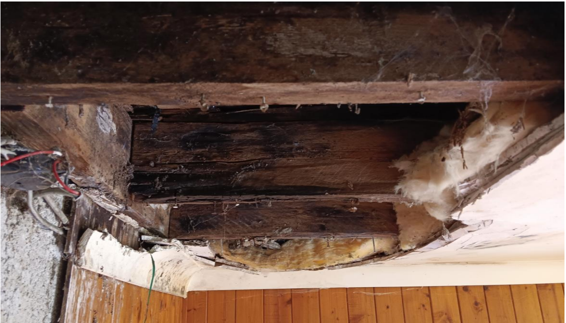
Photo 2 – flat roof over hall. Rotten / wet timber joists – inadequate fixing of joists to trimmer joist.
