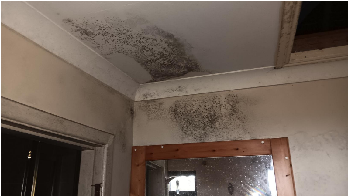
Photo 29 Black mould growth on ceiling due to structurally defective and leaking roof.
