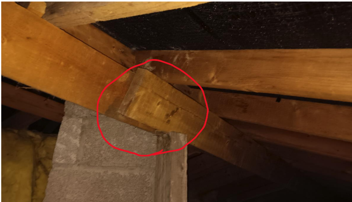
Photo 27– 2no purlins (measuring 75x255 and 63x225 respectively) spanning over entire length of pitched roof with 1No central support (total purlin span = c12m ie approx 6m span per purlin) this is wholly structurally inadequate. Purlin supports to be max 2.4m spacing. Central strut support is inadequate, no fixing of purlins to each other exists (ie splice joint not present). White rot noted on rafters due to damp / lack of attic ventilation. Structural design of roof is required – roof to be replaced
