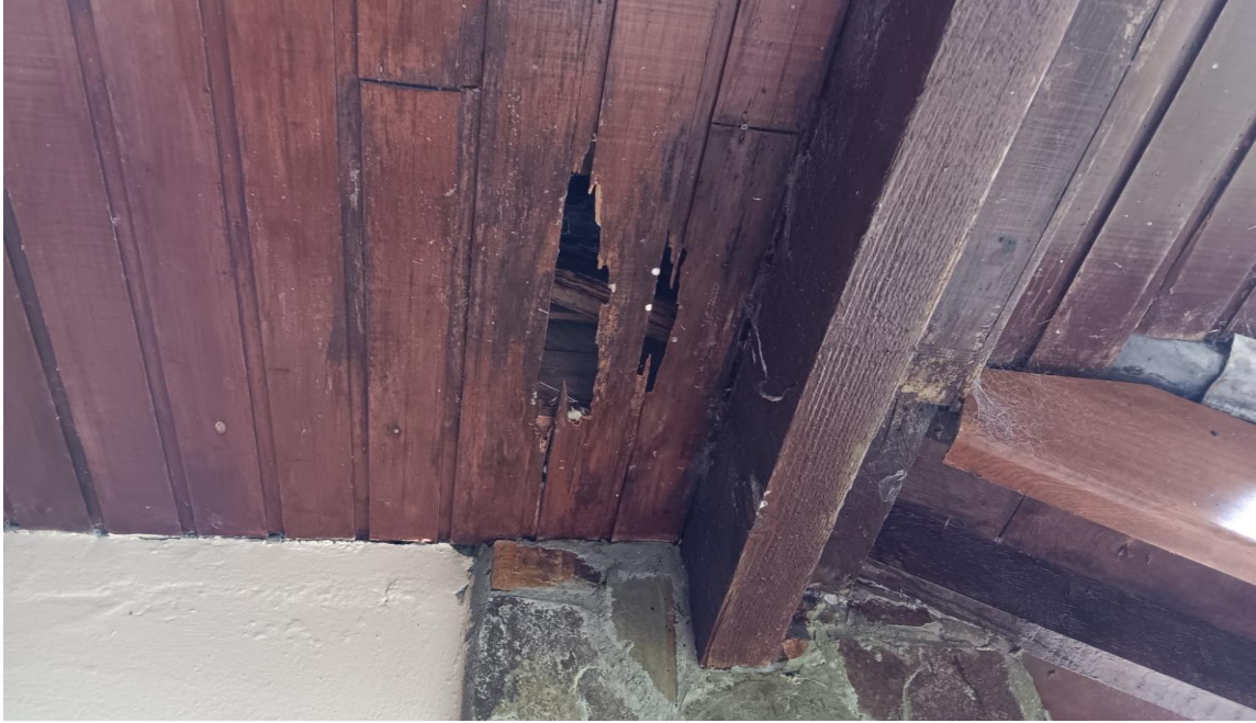
Photo 36 – timber cladding rotten – rafters visible through hole in cladding – rafters also rotten and structurally defective.
