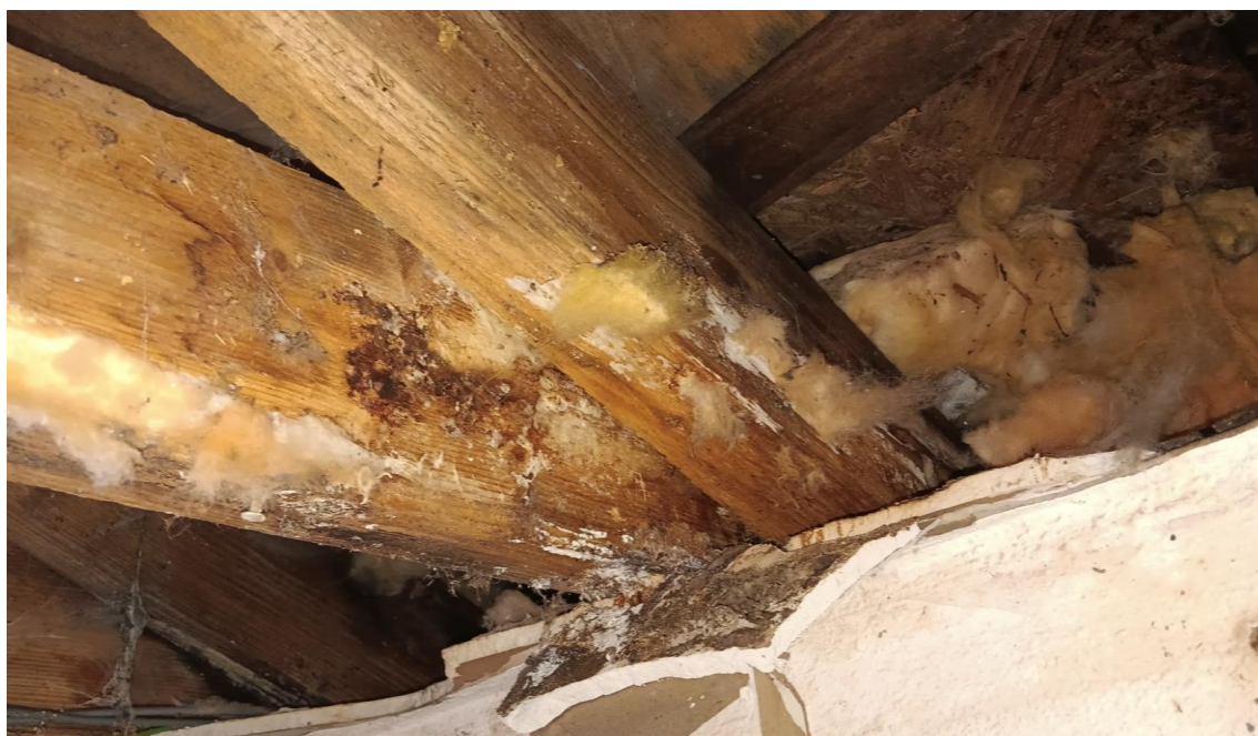
Photo 12 – Ceiling Joists (in pitched roof) lounge 2 , presents fungal growth. Ends of timber (joist and rafter) are rotten / severely damp.
