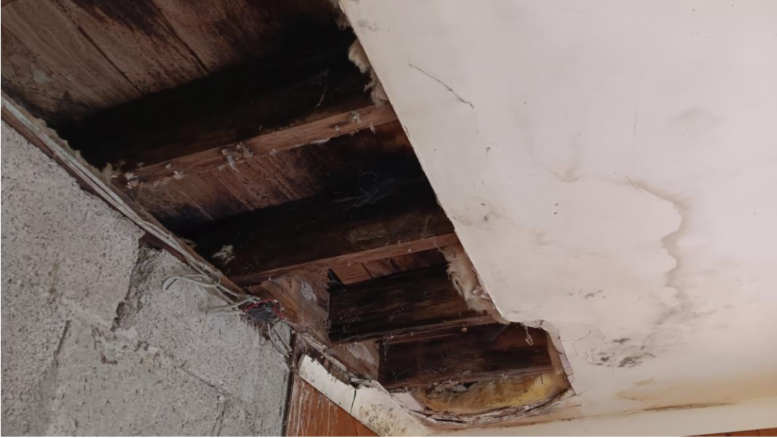
Photo 1 – Rotten timber joists (within flat roof) - incorrect and inadequate bearing – signs of wet rot (cuboidal cracking) and fungal growth – joists visibly wet. Irreparable Structural damage to joists.
