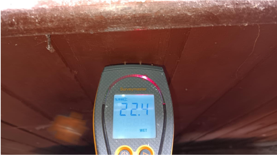
Photo 18– Moisture Content (MC) of timber cladding adjacent wall = 22.4% - damp. Indicates damp wall structure behind cladding.
