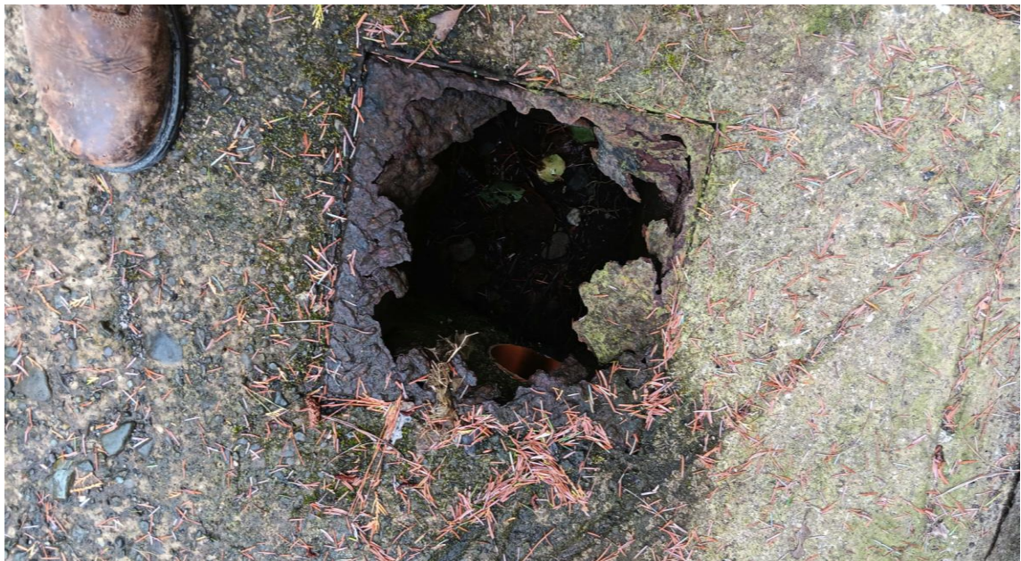
Photo 39 – severe structural damage to drainage cover and frame. Cover completely disintegrated. Substantial health hazard presents.
