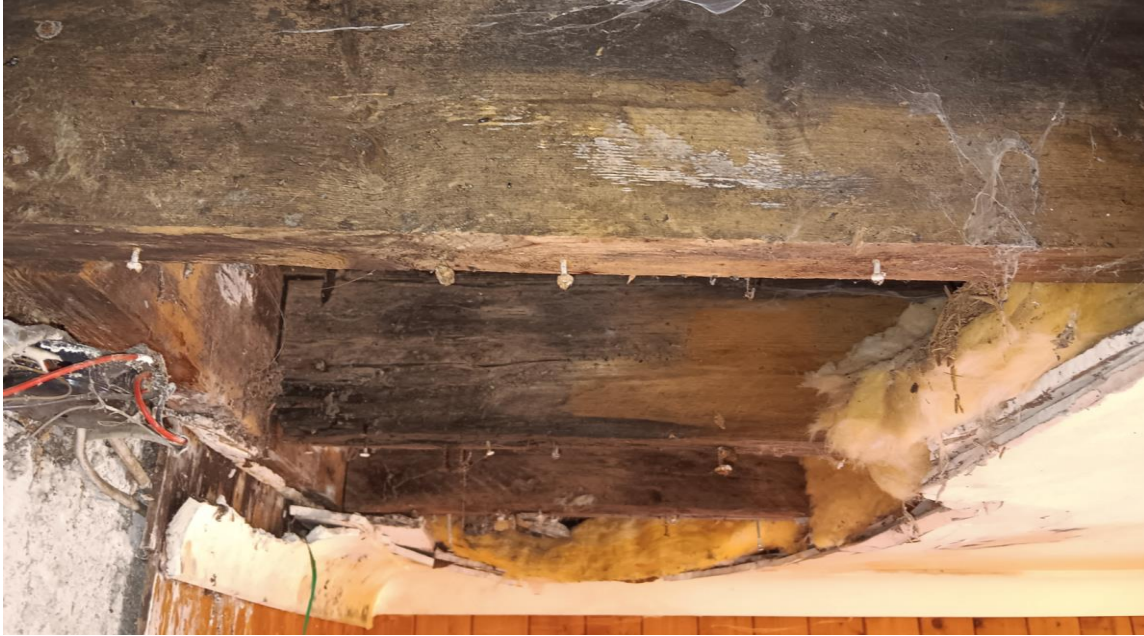
Photo 3 – ‘White rot’ visible on joists. Incorrect fixing to trimmer joist – Structural cracking noted and joists now structurally defective.
