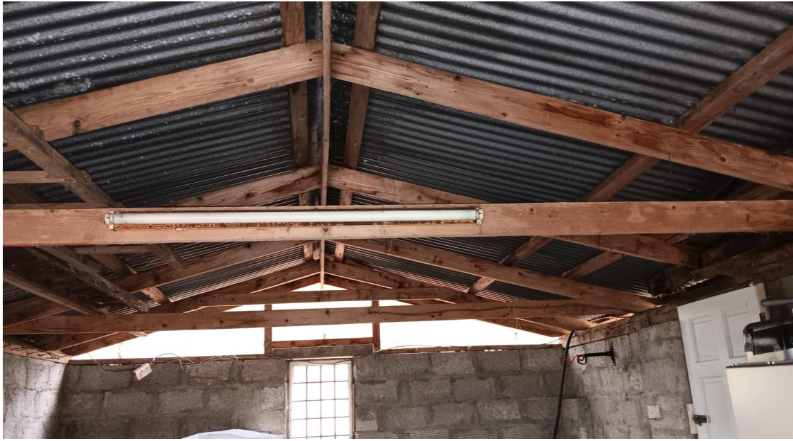
Photo 50 Structural inadequacy of garage roof; Purlins undersized, insufficient rafters, rot presenting at wall plate, no 'holding down' straps present – Entire garage roof to be replaced.
