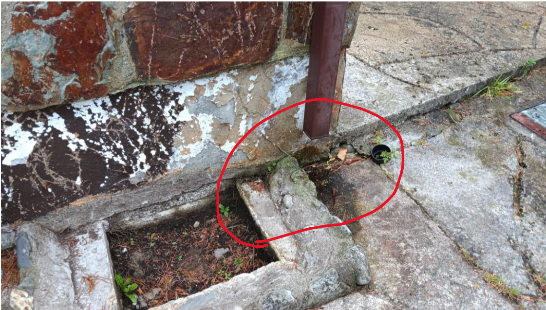
Photo 37 – off-set rainwater outlet pipe from gully – may cause foundation subsidence over time – to be rectified.
