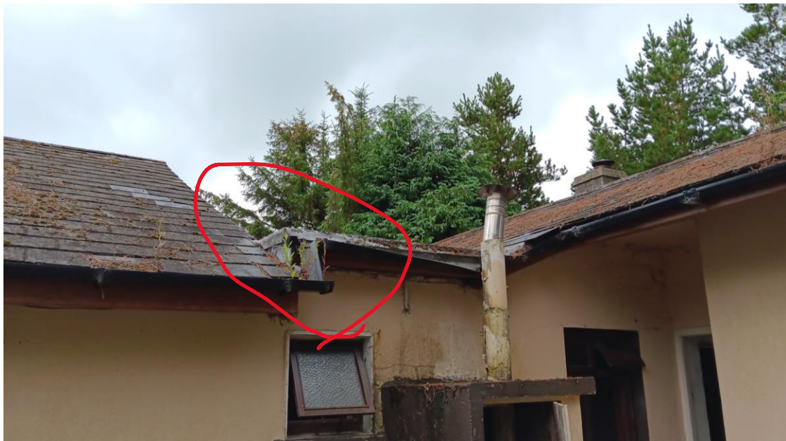
Photo 31 – roof tiles at 'end of life' Note: the probability of asbestos containing material, within the tile is high. Loose /missing tiles exist, and overall defective roof covering. Structurally damaged vertical flue pipe (probably storm damage), water ingress at flat roof within ensuite, due to failed flashing construction. Damp wall behind boiler enclosure penetrating to internal rooms. Note: asbestos flue sleeve around stainless steel flue.
