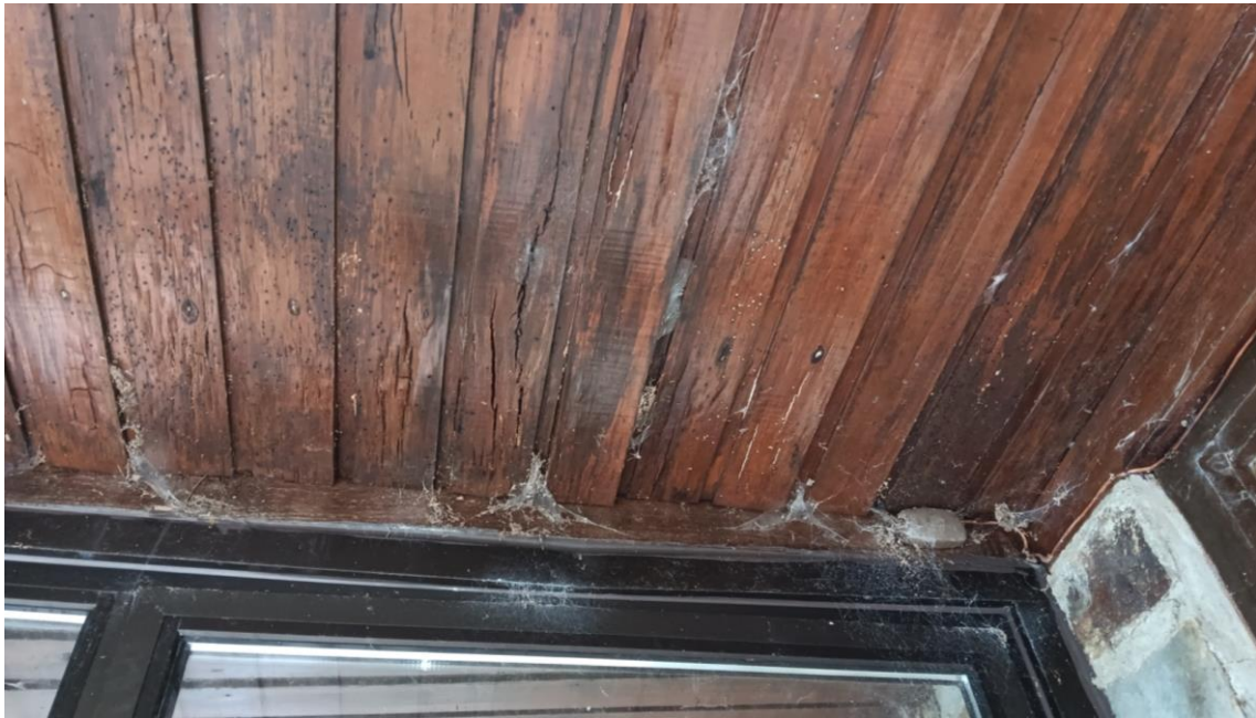
Photo 35 – rotten timber cladding over porch, due to defective roof, at front door.
