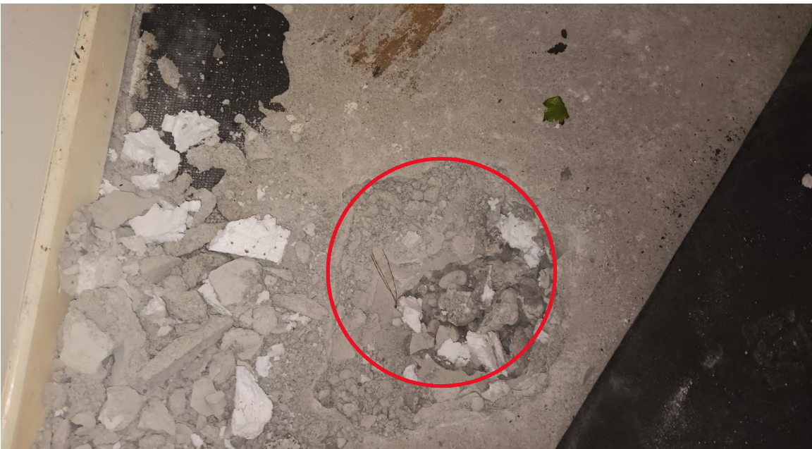
Photo 21– No damp proof membrane within floor (lounge 2) . Weak concrete presents
