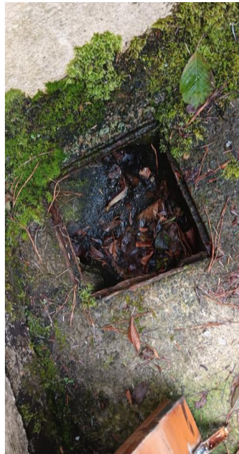
Photo 45 Drainage manhole inadequate - Stuctural fail of sides of manhole, cover and fame. Very poor Construction detail – requires replacement.
