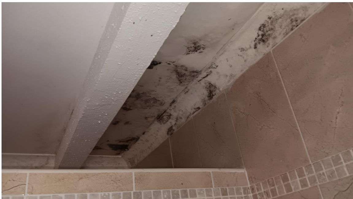
Photo 25 -severe mould growth on ceiling – due to defective roof. Severly damp walls present - black mould on ceiling due to damp.
