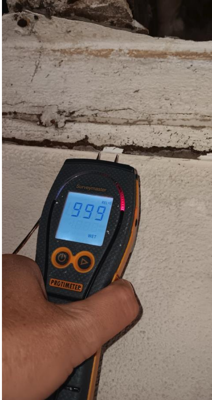
Photo 15– Wall under wall plate – ‘saturated’ (MC index = 999)
