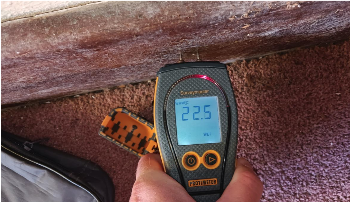
Photo 9 – Skirting board reading as 'damp' (MC – 22.5%) due to damp wall / floor
