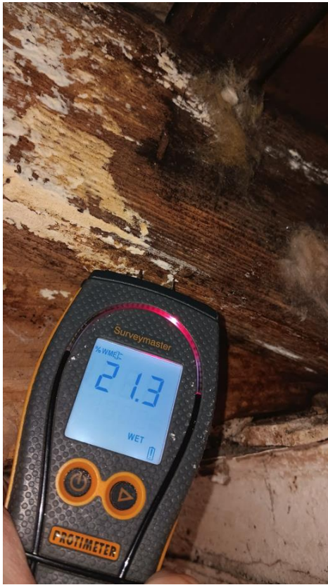
Photo 14 – Timber rafters rotten – MC = 21.3% (damp) white rot present. Timbers irreparable.
