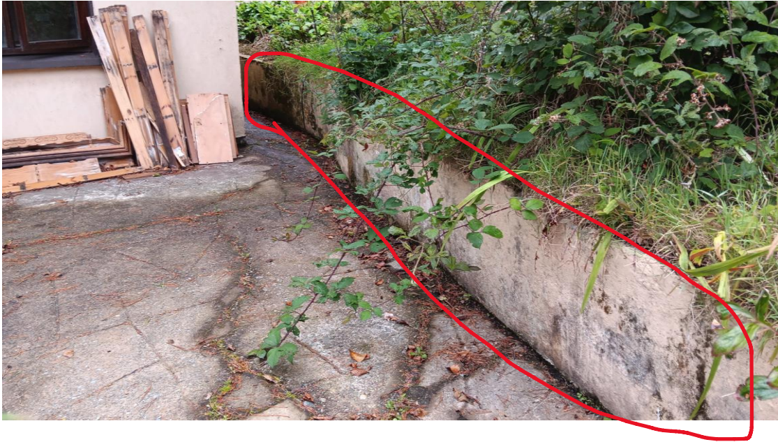
Photo 48 Structural failure of retaining wall – wall severely ‘leaning’ (approx 100mm displacement from vertical)
