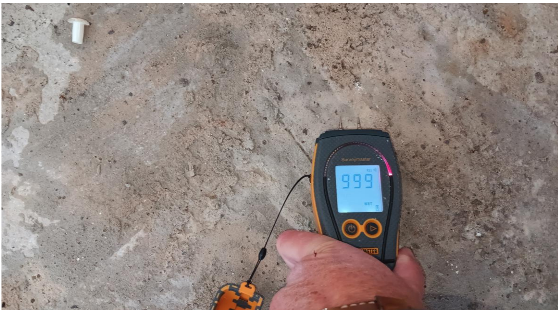
Photo 19– Moisture Content index (MC) of floor (lounge 2) = 999 (ie 'saturated').
