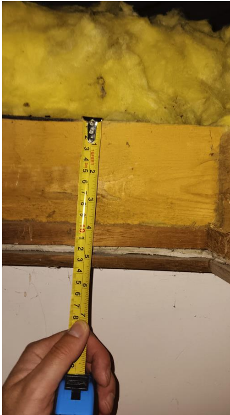
Photo 28 Thickness of ceiling joist = 100mm. inadequate for any pulin loading.
