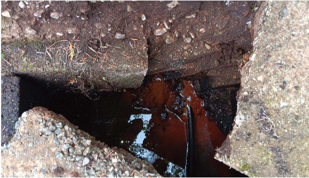
Photo 40 – Severe structural damage to concrete inspection drainage manhole
