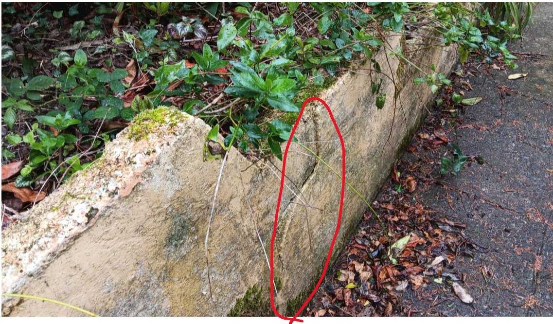
Photo 47 Structural failure of retaining wall – Structural crack presents (c.20mm wide ) wall not vertical and is 'leaning', no 'weep' holes in wall. Land drainage absent.
