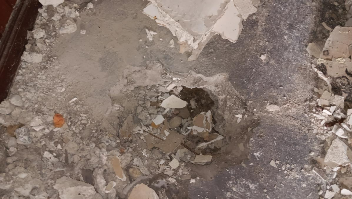
Photo 20– No damp proof membrane within floor (lounge 2) . Floor easily ‘broken out’ - Weak concrete, not suitable as structural slab.
