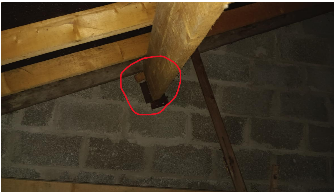
Photo 23– Structurally inadequate purlin fixing to gable wall. No 'birdsmouth' joint in raft-purlin connection.
