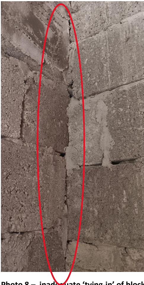
Photo 8 – inadequate 'tying-in' of blockwork – no 'keying in' of blocks, and no ties at wall junction. Poor bed and perpend mortar joints.
