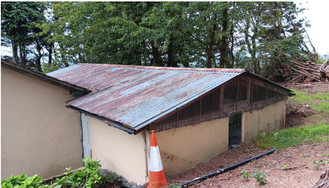
Photo 51 Overview of rear of garage – roof structurally inadequate. rear gable wall potentially acting as a retaining wall – current wall not adequate as a retaining wall. (see photo 52)
