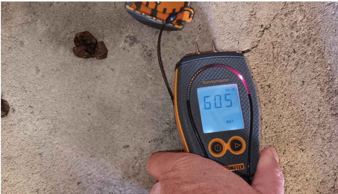
Photo 10 – Hall floor reading as 'wet' (MC index = 605) – lack of correct damp proofing.
