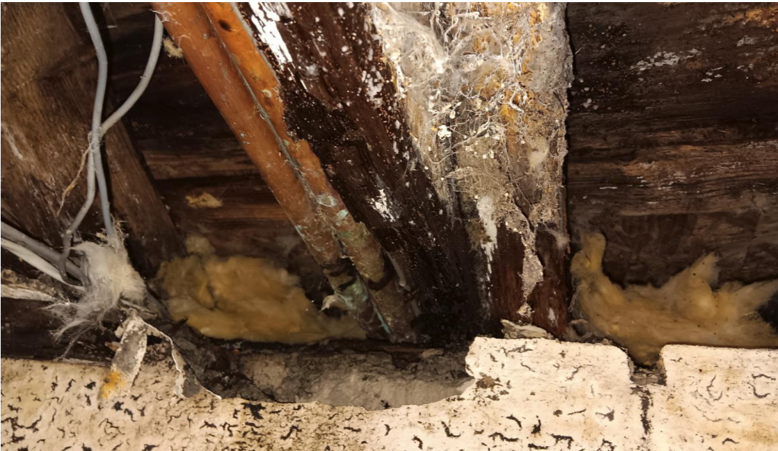
Photo 16– Severe degradation of timber joists and rafter – easily ‘crumbled’ by hand on timber surface– fungal growth clearly present.
