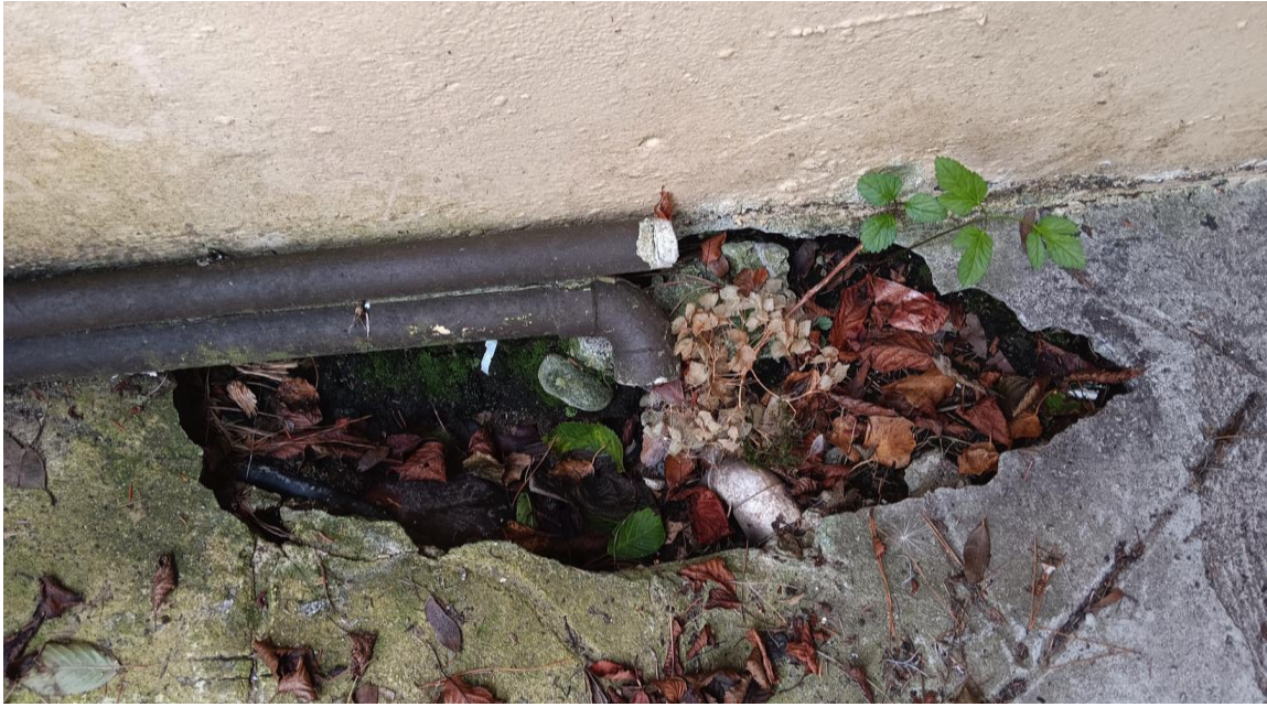
Photo 46 Drainage gully inadequate - Very poor construction detail, and arrangement contrary to Building Regulations
