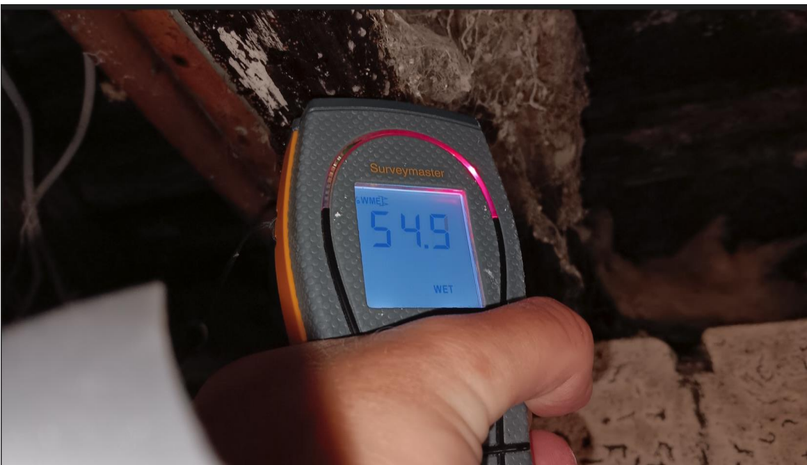
Photo 17– Moisture Content (MC) of timber joist = 54.5% - severely wet.
