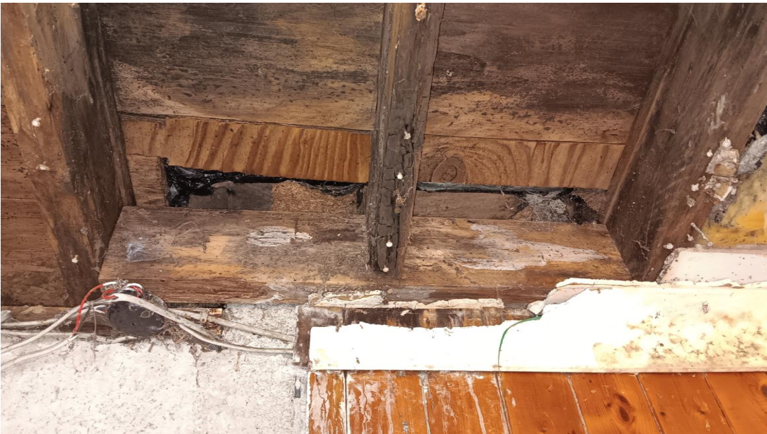
Photo 6 – Rotten flat roof joists – cuboidal fractures present – visible 'white rot' and severe timber degradation noted. Severe damp penetrating through structural roof deck.
