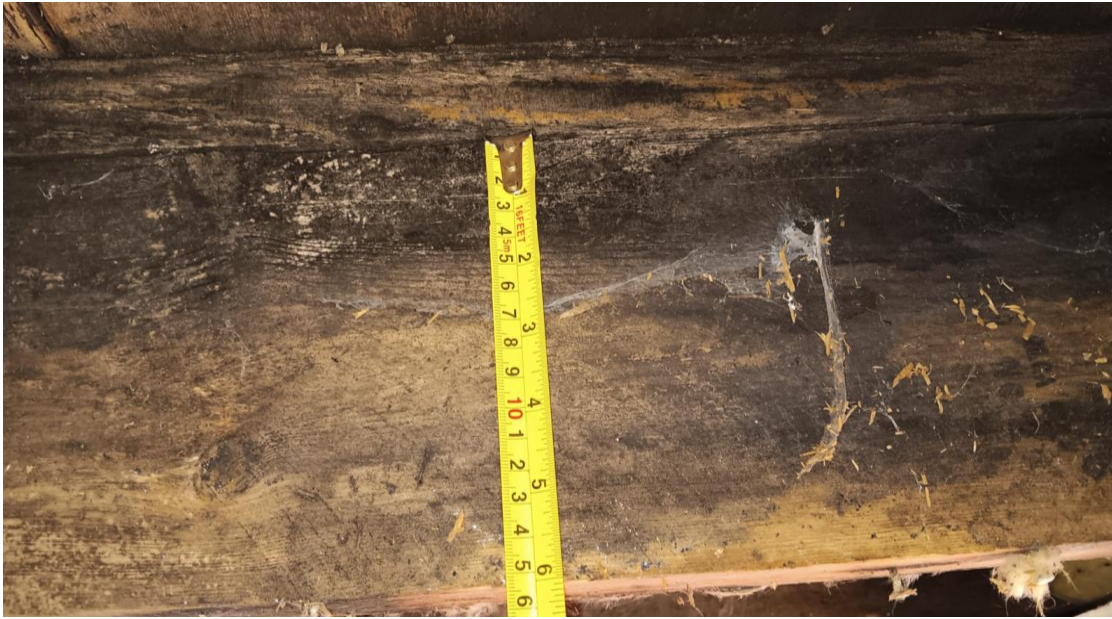
Photo 7 – Depth of flat roof joists measures 150mm – undersized for flat roof loads given required span. Structural inadequate.
