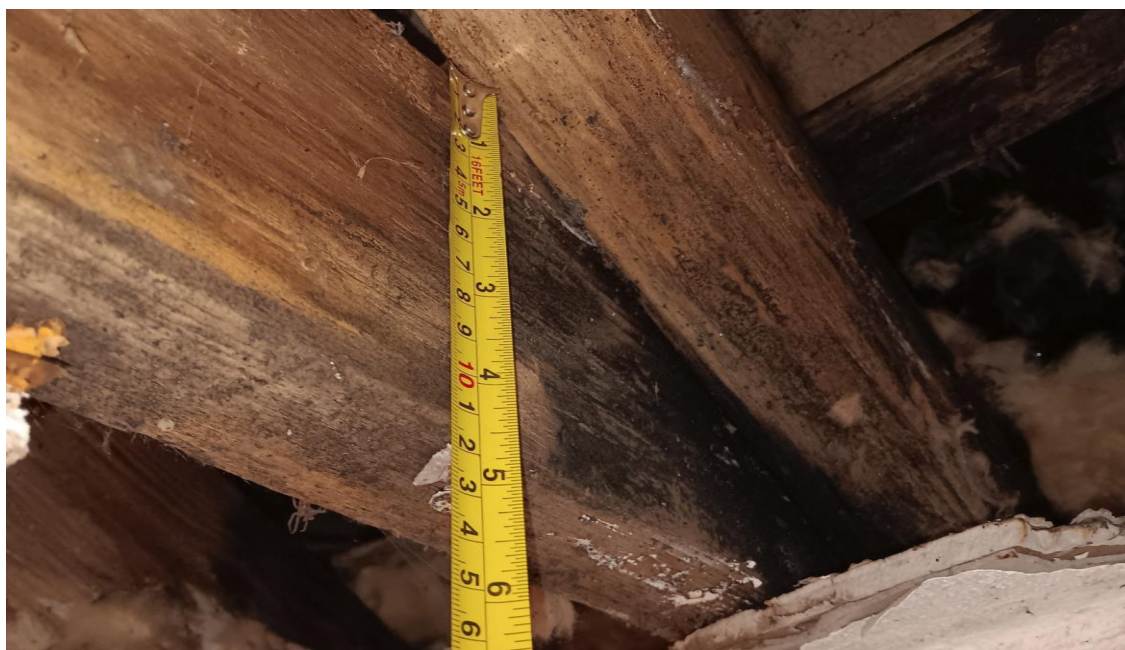
Photo 11 – Ceiling Joist (in pitched roof) lounge 2 , measures 110mm. Undersized given span. Substantial damp and timber damage at wall junction, on wall plate. Wet rot / timber damage visible
