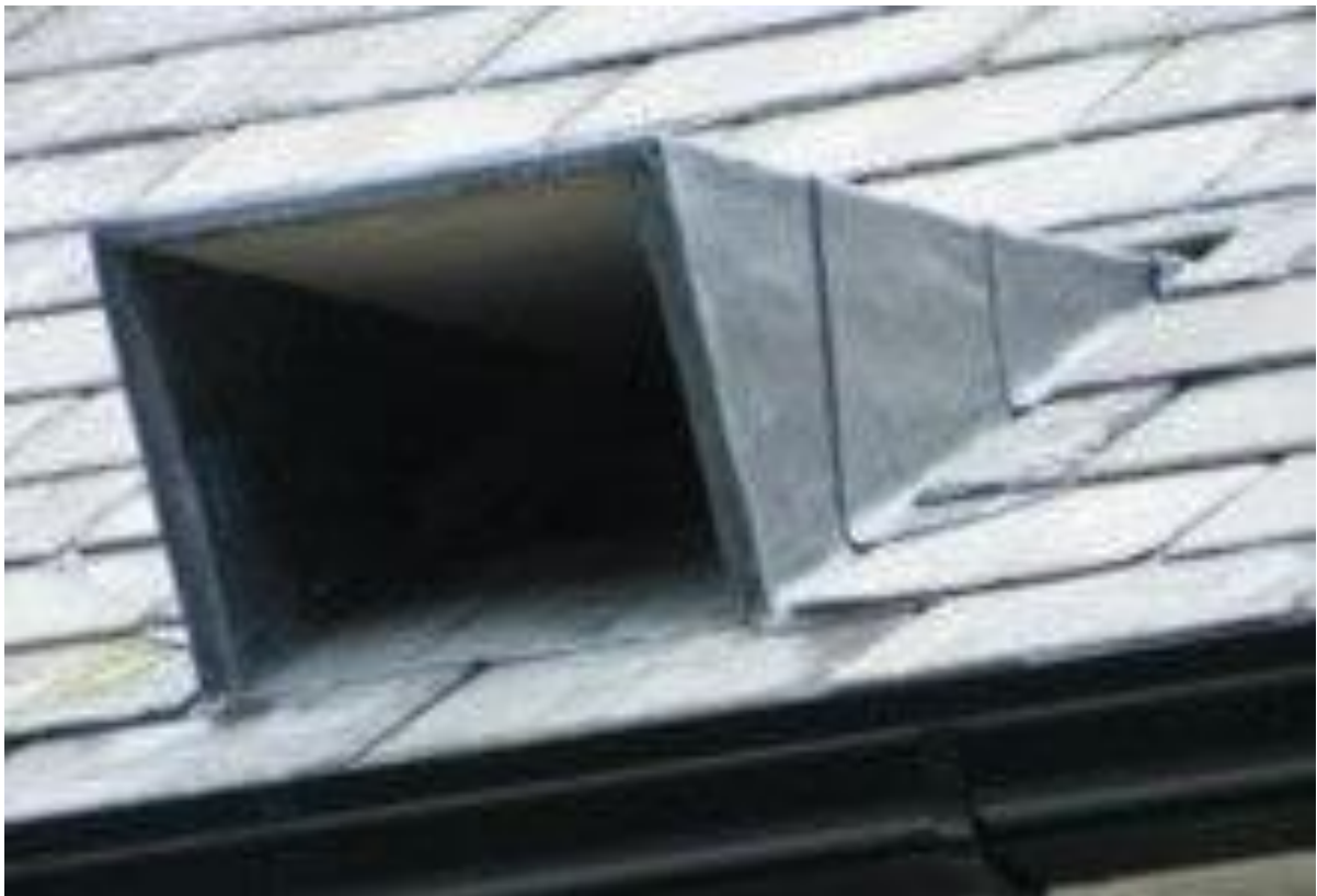
Photo 4: Dormer access point to be installed in roof to provide access for lesser horseshoe bats.
