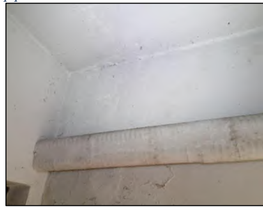
Plate 3-3 Heating pipe wrapped in insulation
