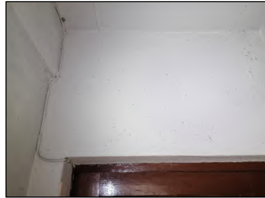
Plate 3-2 Droppings above door by heating pipe
