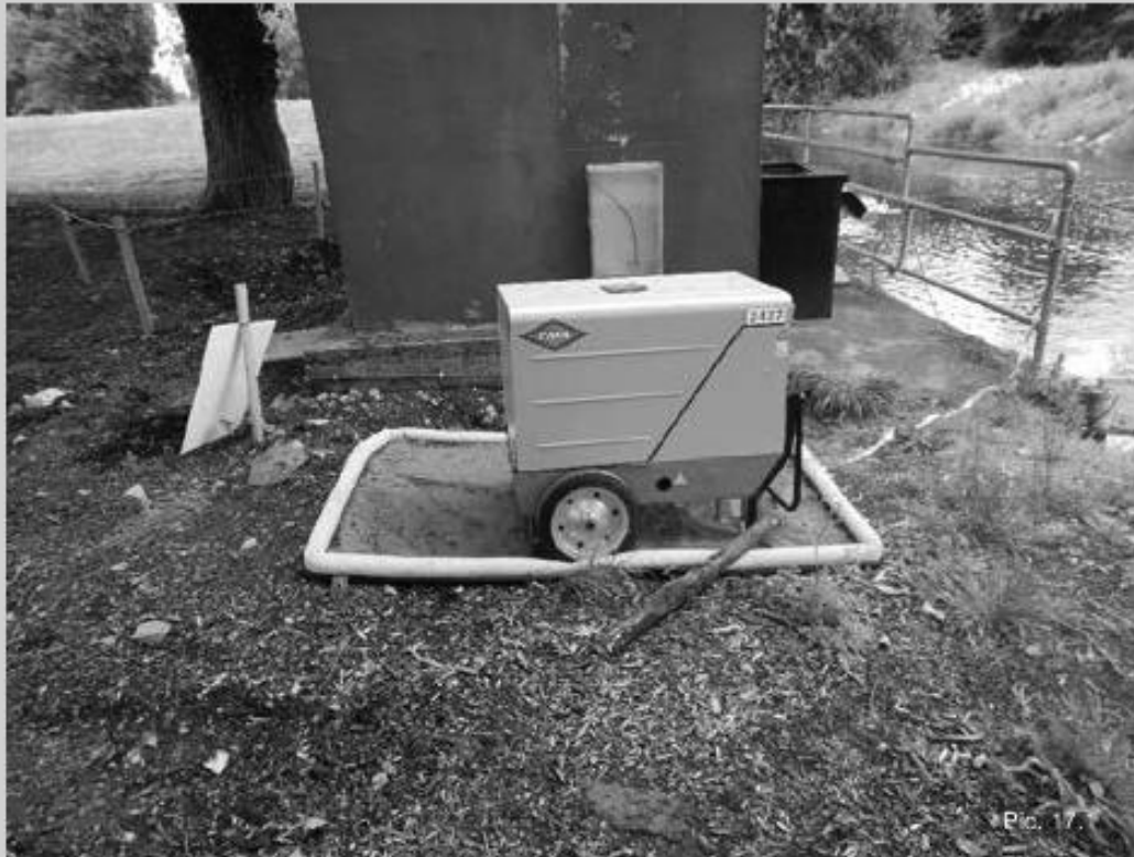
Pic 17.1 Plant nappy under a compressor.
