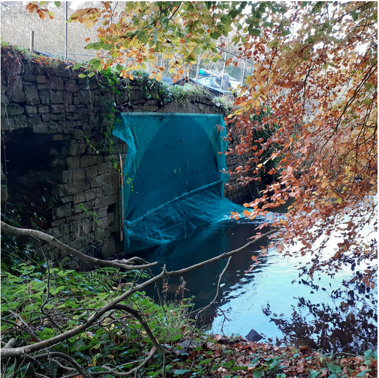
Plate 5: Closed netting on Claddy Bridge, Bective, Co. Meath.
