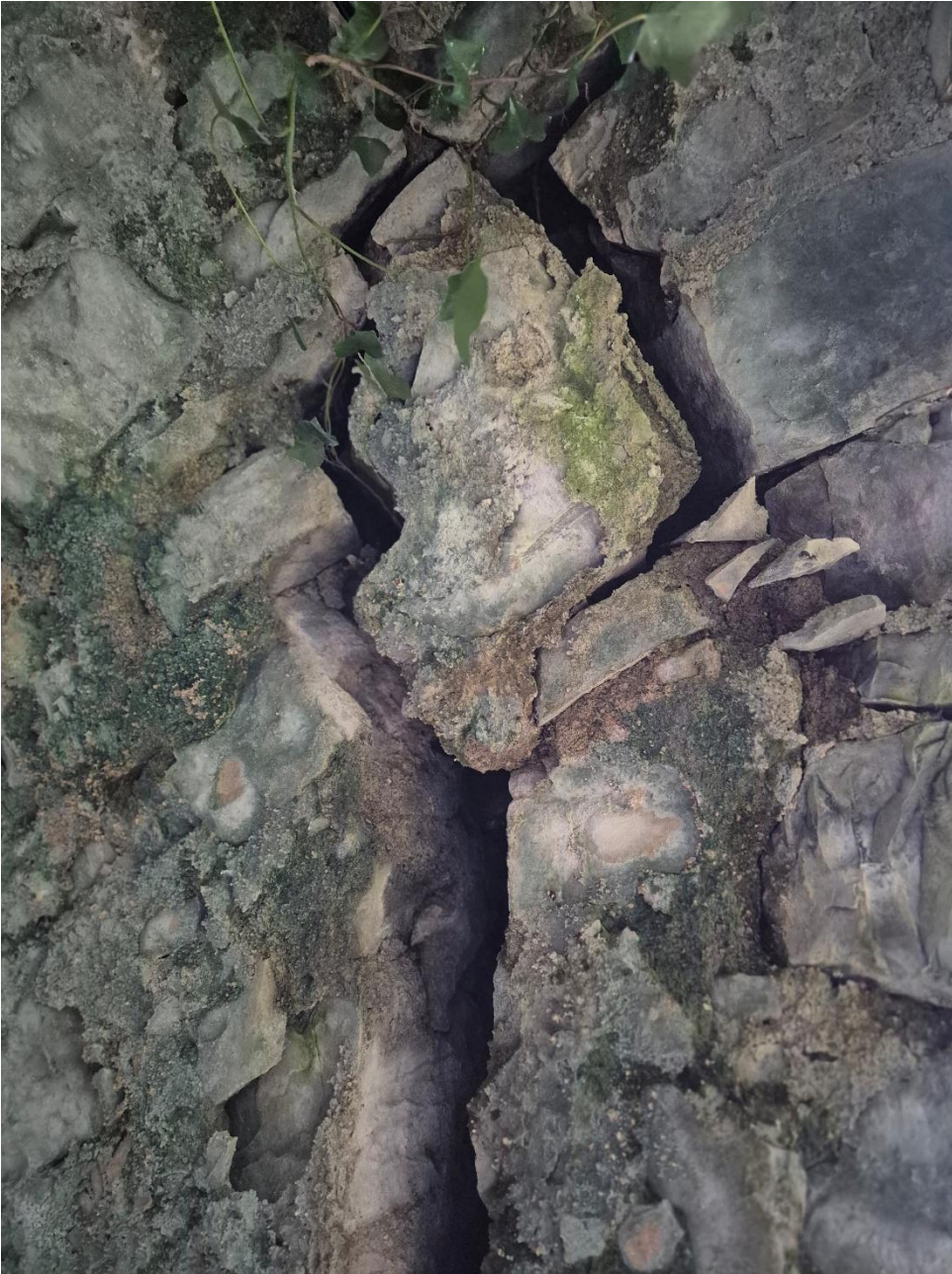
Plate 1b: Continued from Plate 1a - large crack in Drumcree Bridge, Co. Westmeath.
