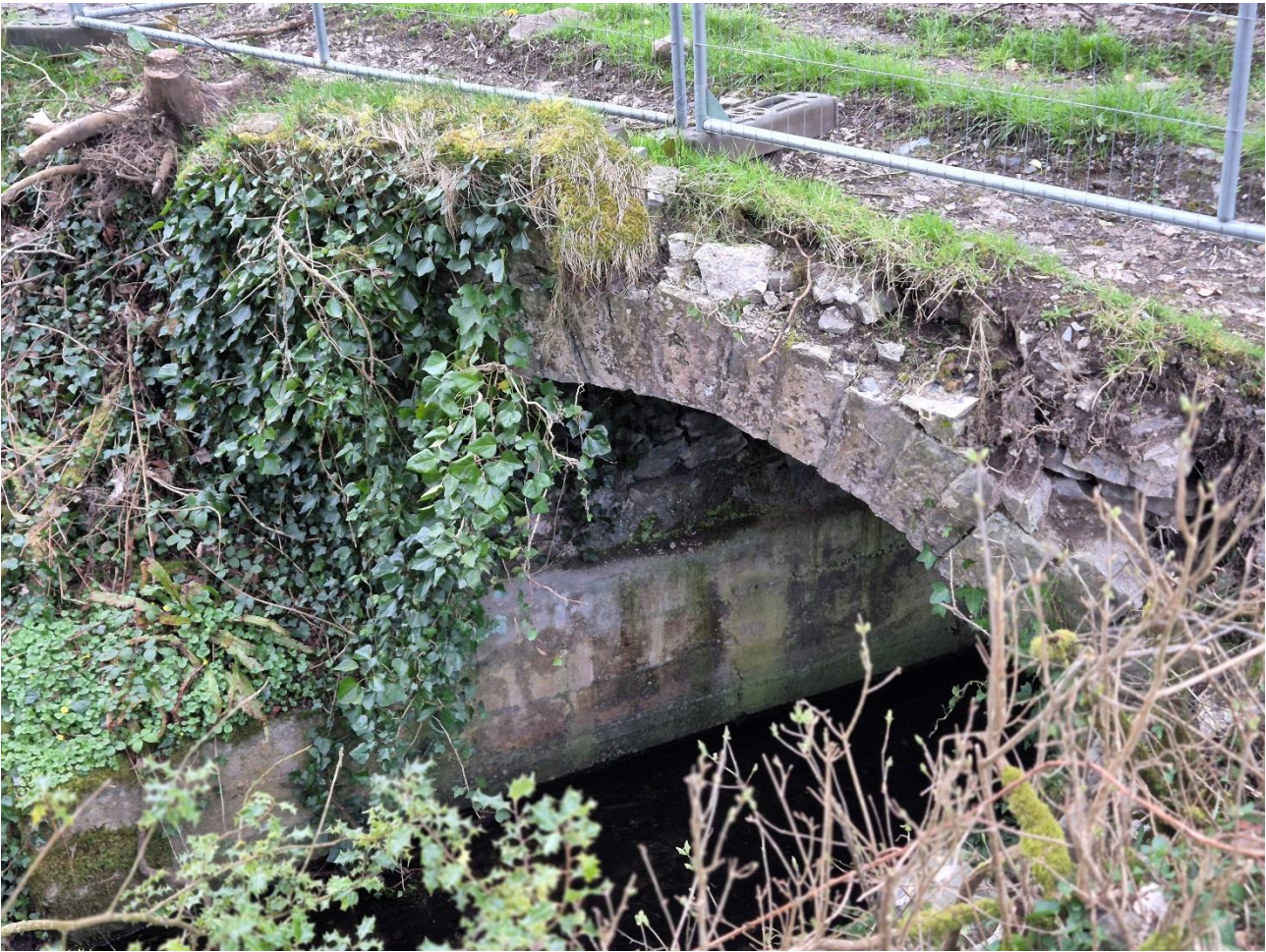
Plate 3: View of in Drumcree Bridge, Co. Westmeath – Section where the large crack is located.
