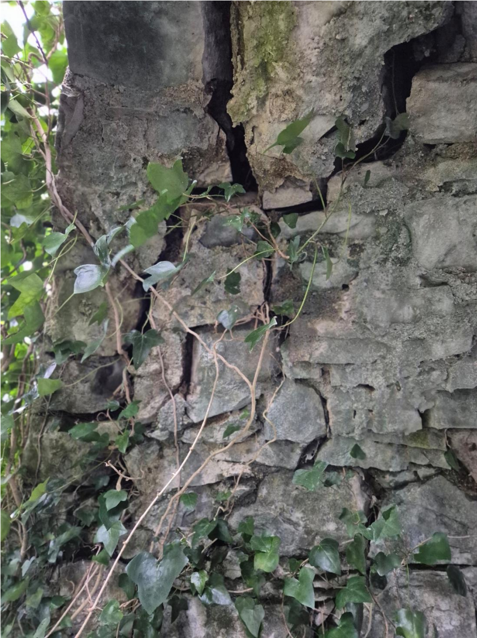
Plate 1c: Continued from Plates 1a & 1b - large crack in Drumcree Bridge, Co. Westmeath.
