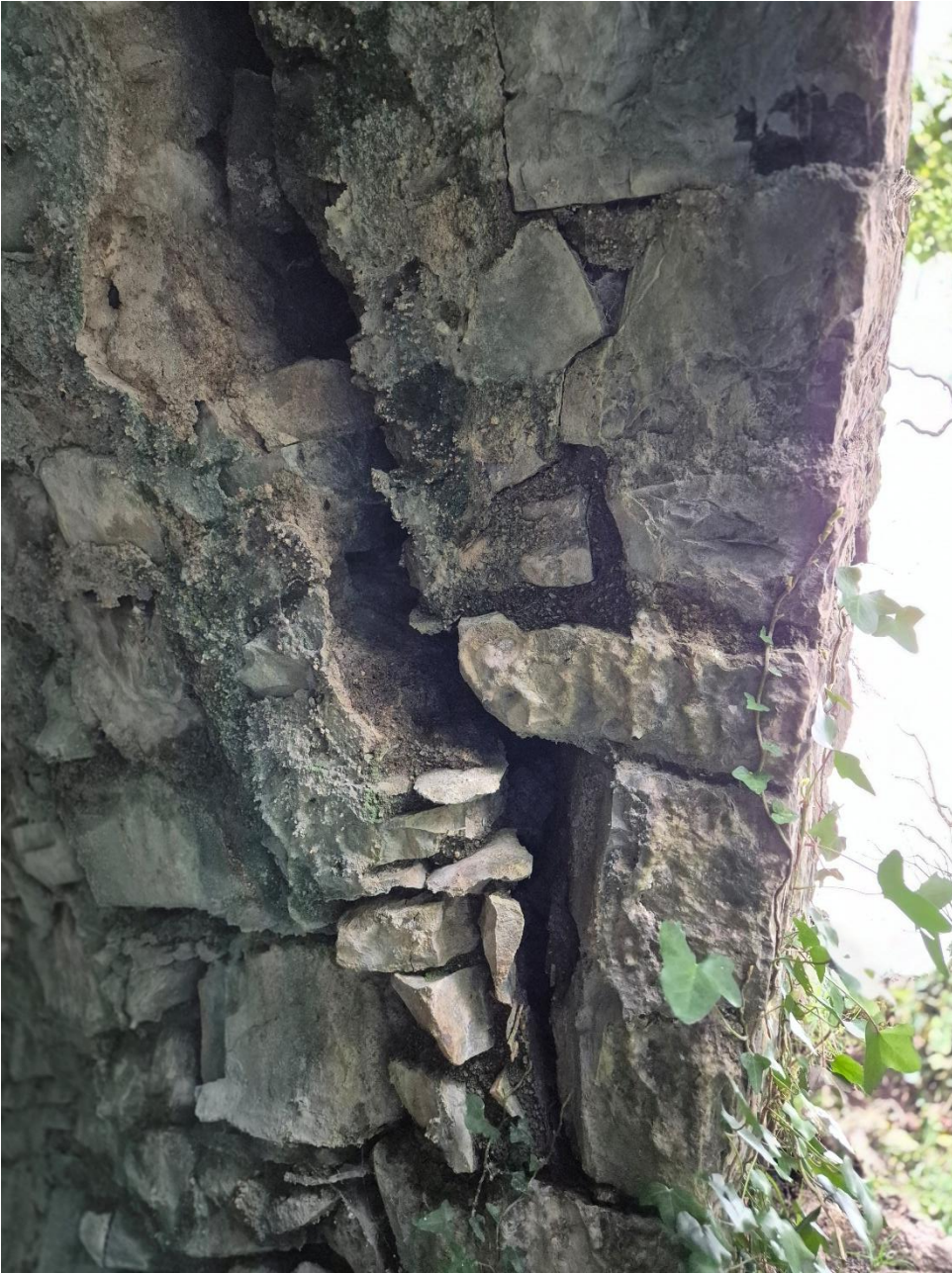
Plate 1a: Section of large crack in Drumcree Bridge, Co. Westmeath.
