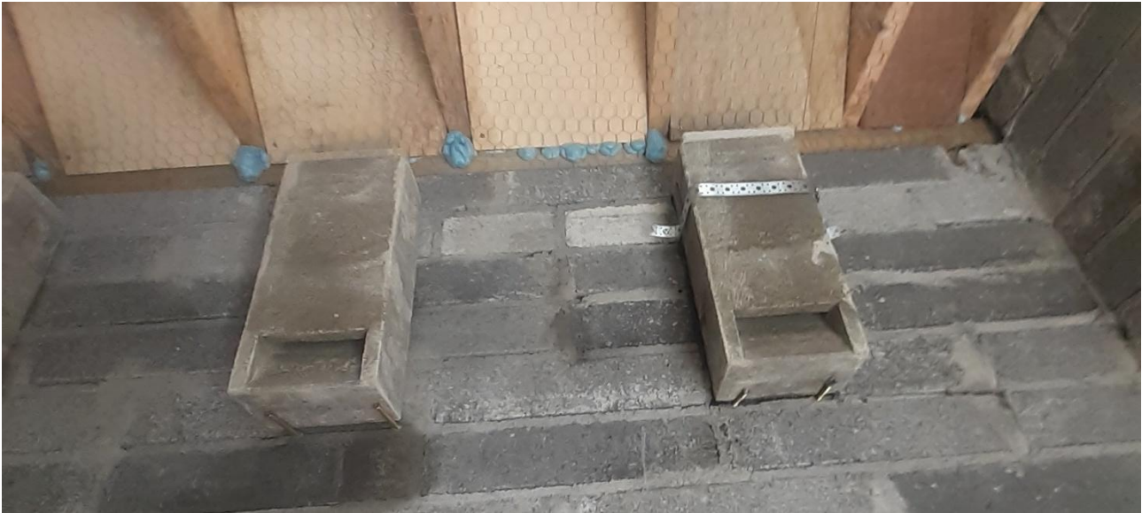
Plate C: Bat Tubes fixed onto internal ground floor wall (Oldstreet Substation bat House, Co. Galway).
