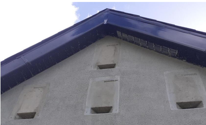
Plate B: Winter Bat Boxes inserted into wall (Oldstreet Substation bat House, Co. Galway).
