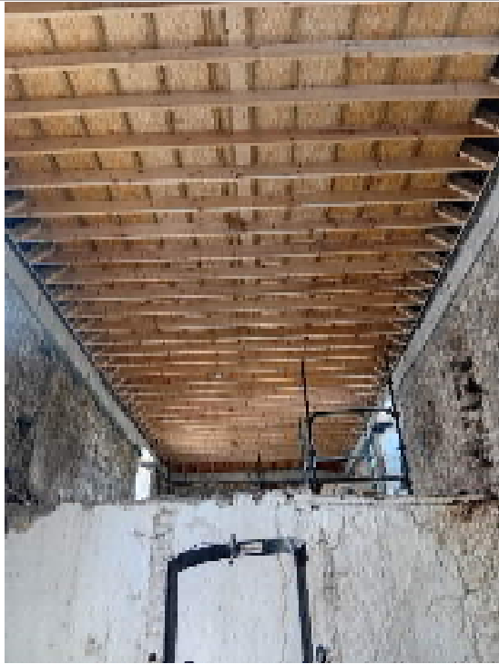
Stable B Interior – looking east. Current access. Access door will be provided from the 9m bat loft space internally and letterbox opening installed on the Western Gable per license.
