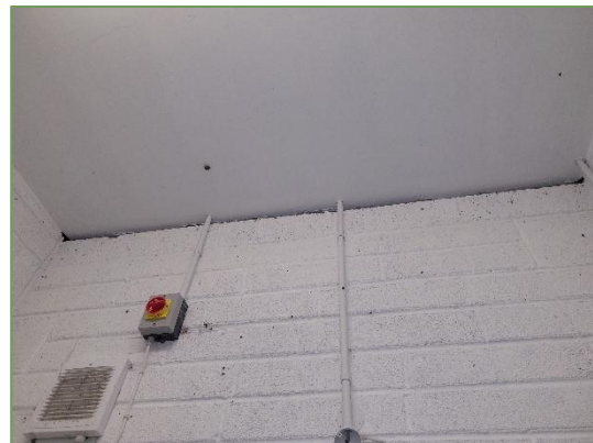
Plate 3.6 Gaps between wall and ceiling appear to provide interior access for bats.
