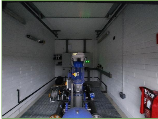
Plate 3.1 Interior of pump room.
