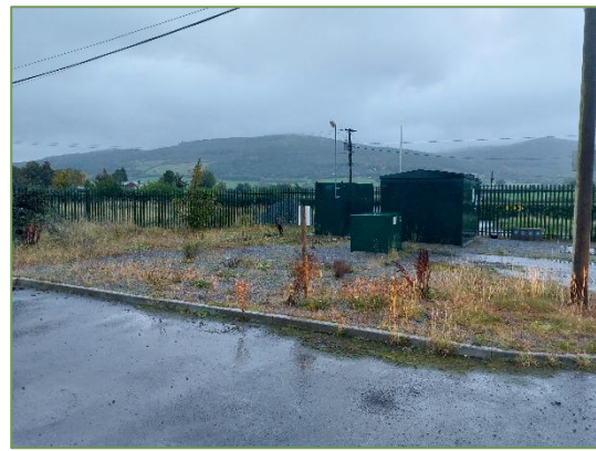
Plate 3.10 Metal structures (control room etc.) within the study area.
