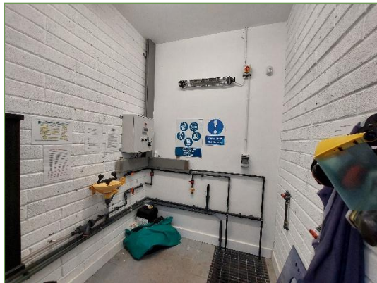
Plate 3.3 Interior of Pump House.
