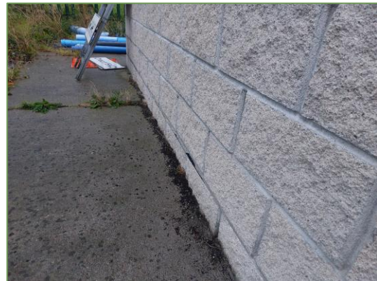
Plate 3.4 Accumulation of droppings on the exterior.
