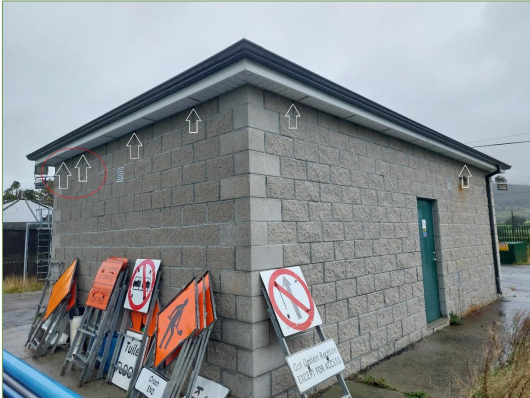
Plate 3.12 View of south eastern side of Pump House building, arrows indicate observed access/egress points. Red circles indicate those observed to most commonly observed to be used.
