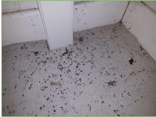
Plate 3.7 Bat droppings within Pump House.
