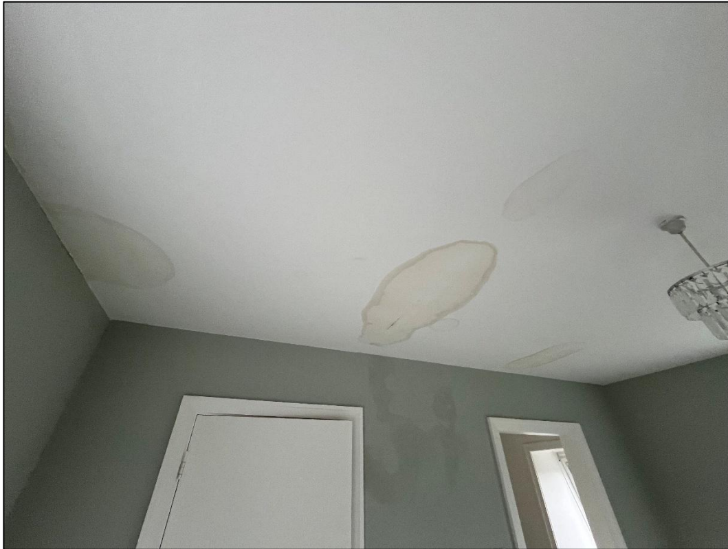
Figure 6. Example of visible water ingress inside existing house.
