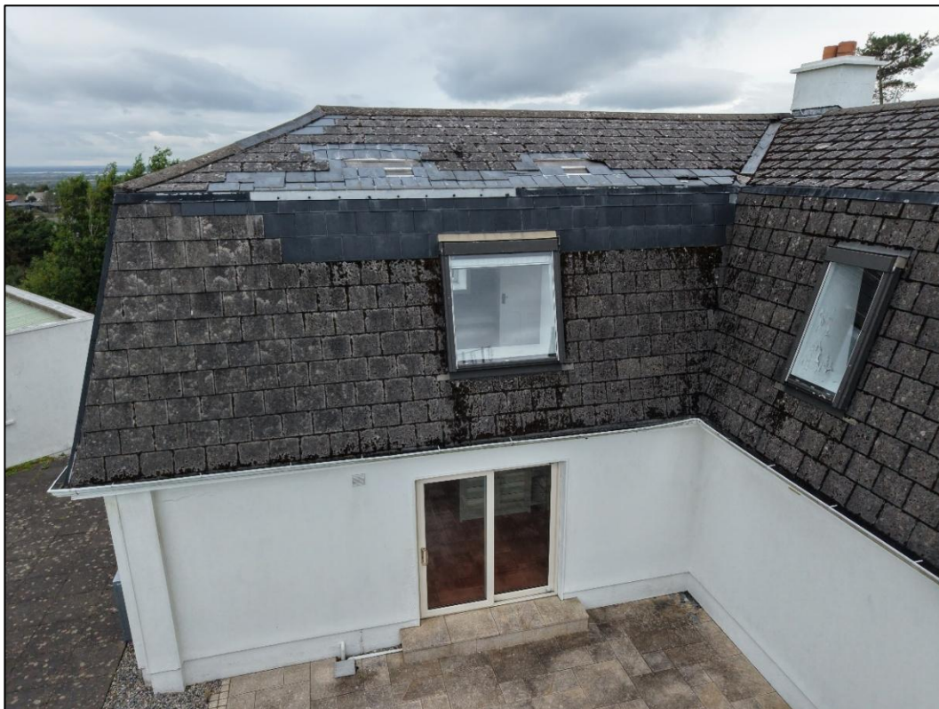
Figure 5. Example of roof damage, missing and loose tiles.
