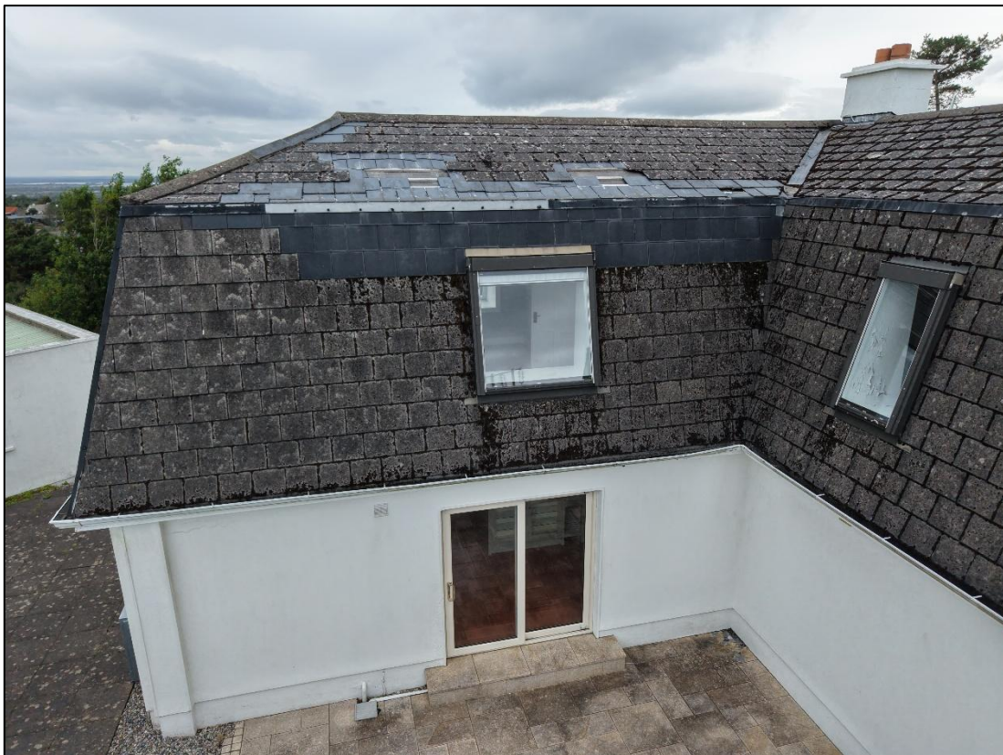
Figure 11. Roof repair, missing and loose tiles.
