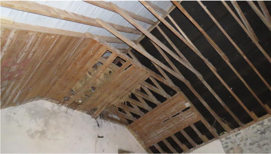
Photo 32 – roof of granary – half bitumen felt lining and half breathable membrane
