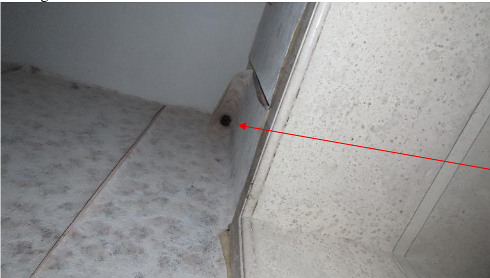
Photo 15 – two brown long-eared bats roosting in peeling wall paper
