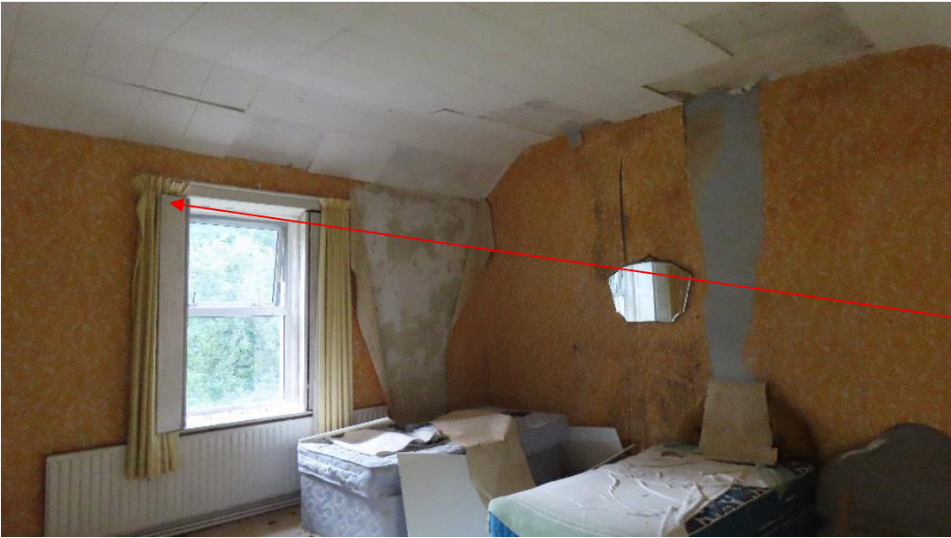
Photo 12 – upstairs bedroom with bat droppings on floor below curtains. Brown long-eared bats were previously roosting in the curtains
