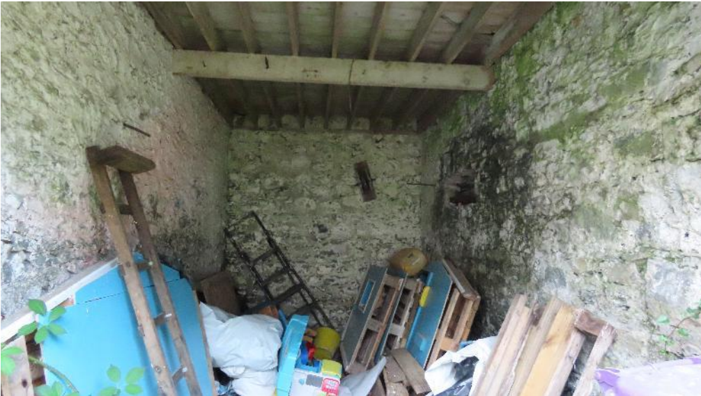
Photo 24 – ground floor of granary building used for storage. Wooden loft floor above
