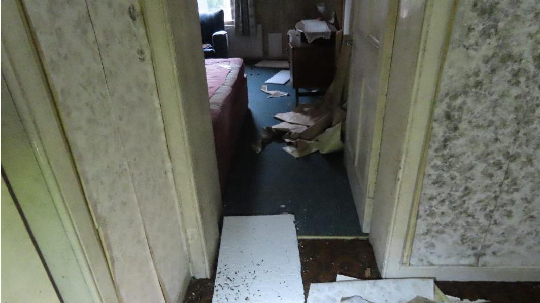
Photo 17 – bat droppings on ground directly below roosting bats
