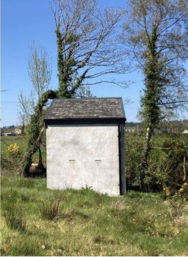
Pump house type roost with natural slate roof lined with bitumen felt
