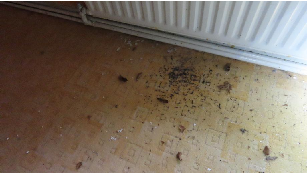
Photo 13 – brown long-eared bat droppings on ground below curtains
