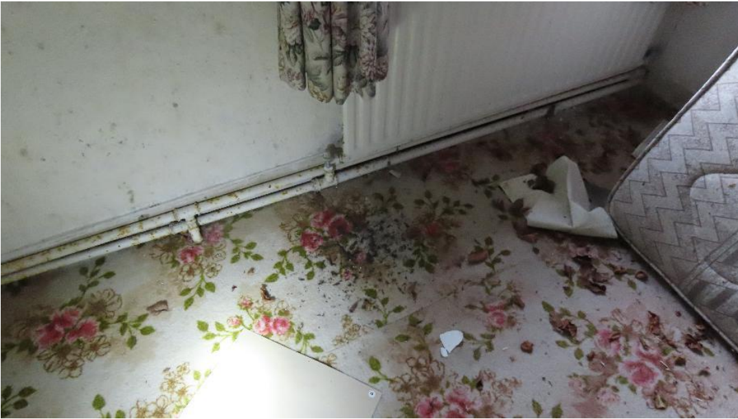
Photo 18 – bat droppings on floor below curtains
