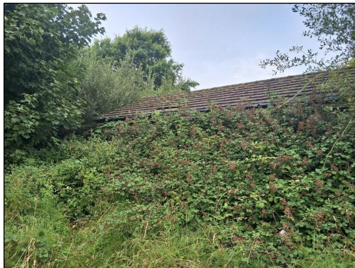
Plate 4-11 Derelict House within the walled garden to the southwest of the schoolyard.
