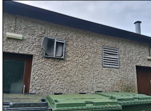
Plate 4-4 Broken air vent to the north of the building
