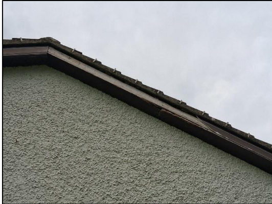
Plate 4-9 Gap between the soffit and barge board of the Art Building
