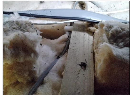
Plate 5-4 Three storey House: Bat dropping found at the attic entrance.
