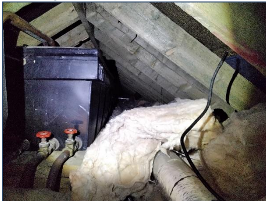
Plate 5-3 Three storey House: Attic space Section B and water tank – not accessed.
