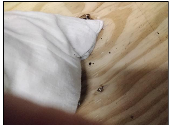
Plate 5-2 Three storey House: Small number of bat droppings found throughout the attic space.
