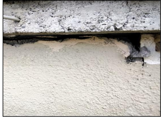
Plate 5-6 Three storey House: Small hole and crevice to the rear external wall.
