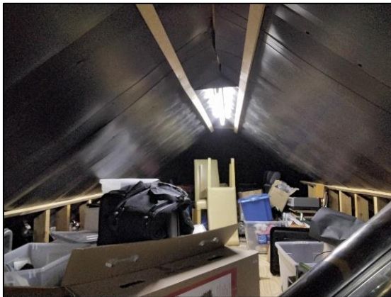
Plate 5-1. Three storey House: Attic storage area with plastic sealed ceiling and felt.
