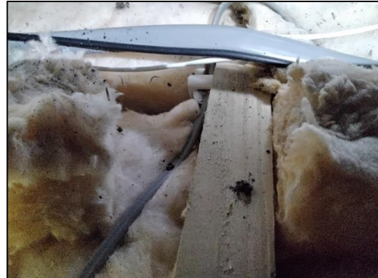
Plate 4 Three storey House: Bat dropping found at the attic entrance.
