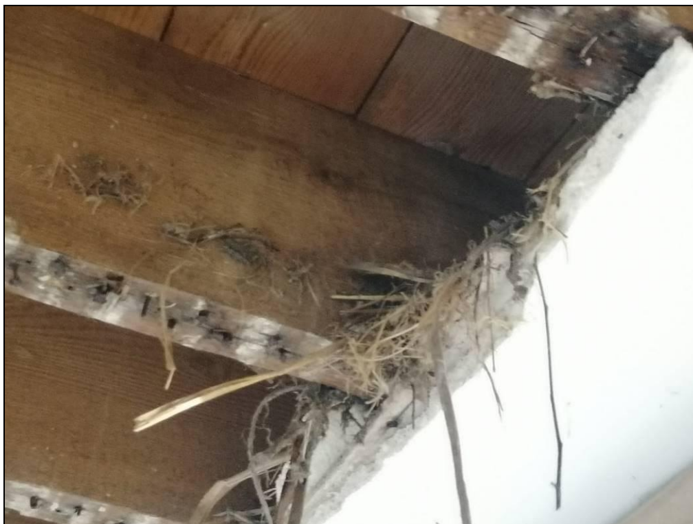
Photo 32. Starling nest in basement.
