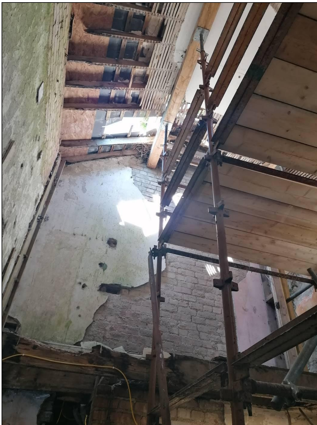
Photo 31. Jackdaw nest above old plaster laths.
