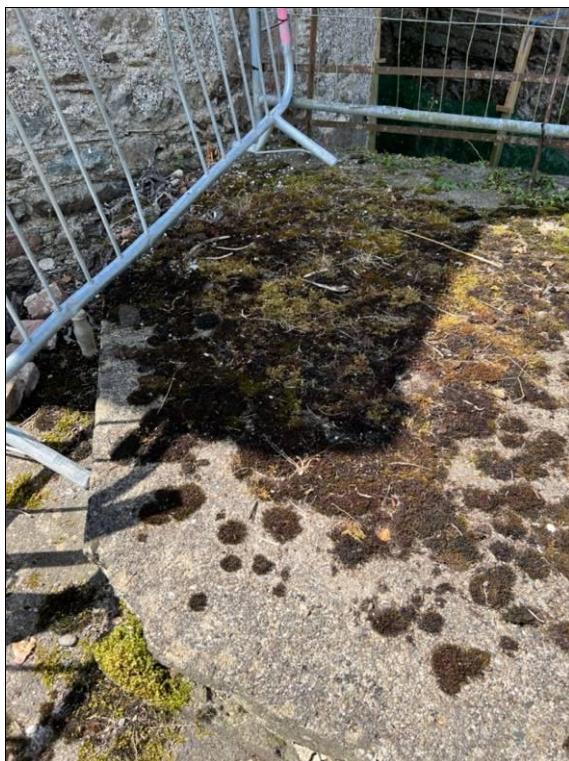
Photo 8. Bryophytes on concrete steps to east of house.
