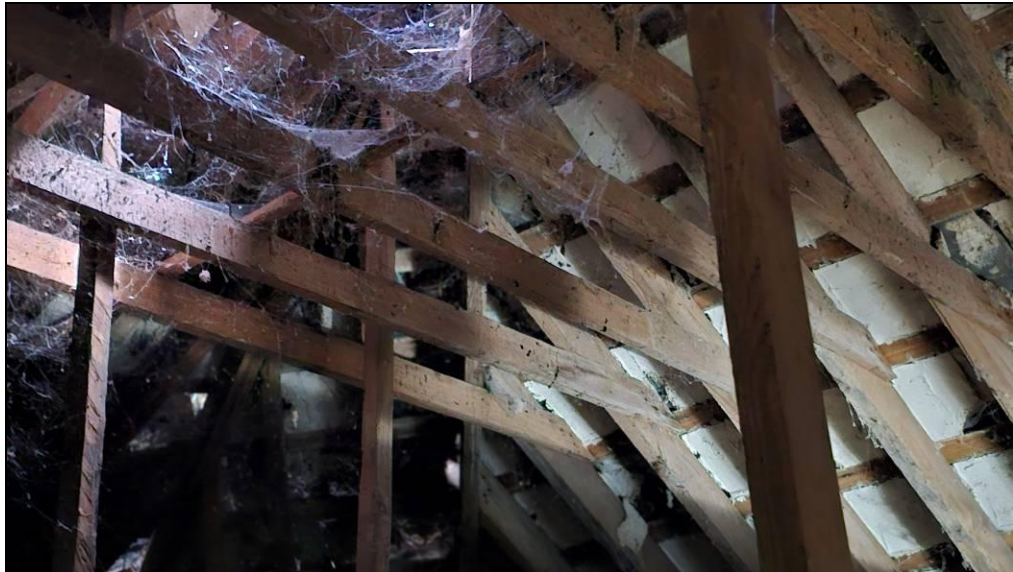
Photo 19. Repairs to the roof of the bullnose have created a darkened attic space.
