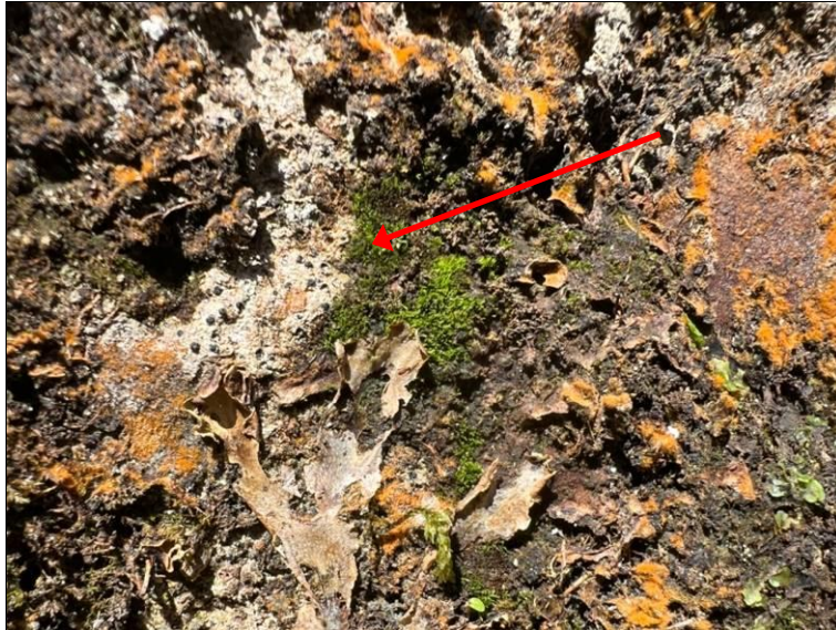
Photo 11. Gyroweissia tenuis on mortar on basement wall.
