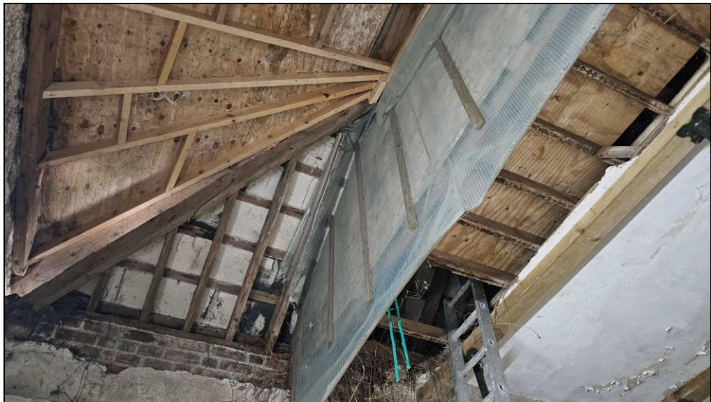
Photo 18. Repairs to the roof of the bullnose have created a darkened attic space.
