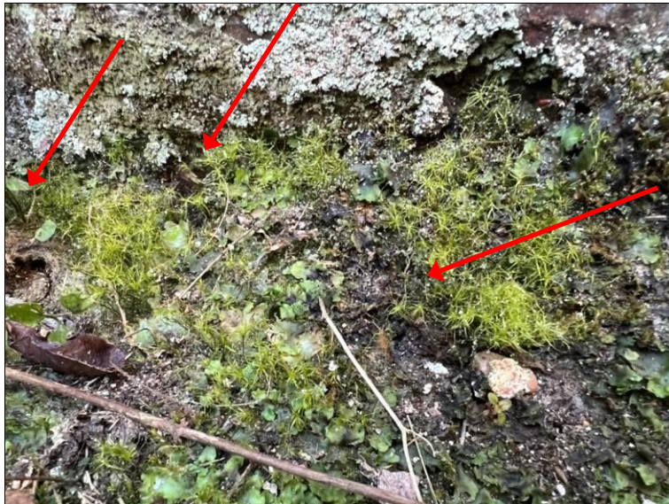
Photo 12. Leptobryum pyriforme at bottom of basement wall.
