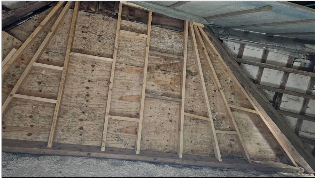
Photo 17. Repairs to the roof of the bullnose have created a darkened attic space.
