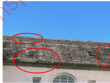
Figure ix: Gaps between slate roof tile at the front of B1's roof.
