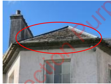
Figure viii: Gaps between slate roof tile at the front of B1's roof.
