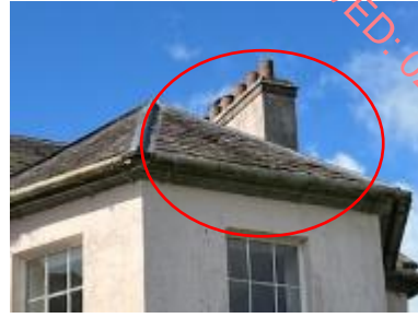
Figure vii: Gaps between slate roof tile at the front of B1's roof.
