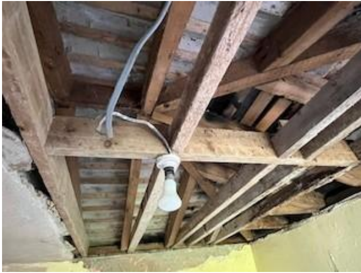
Exposed underside of B14s roof through gaps from missing ceiling material.
