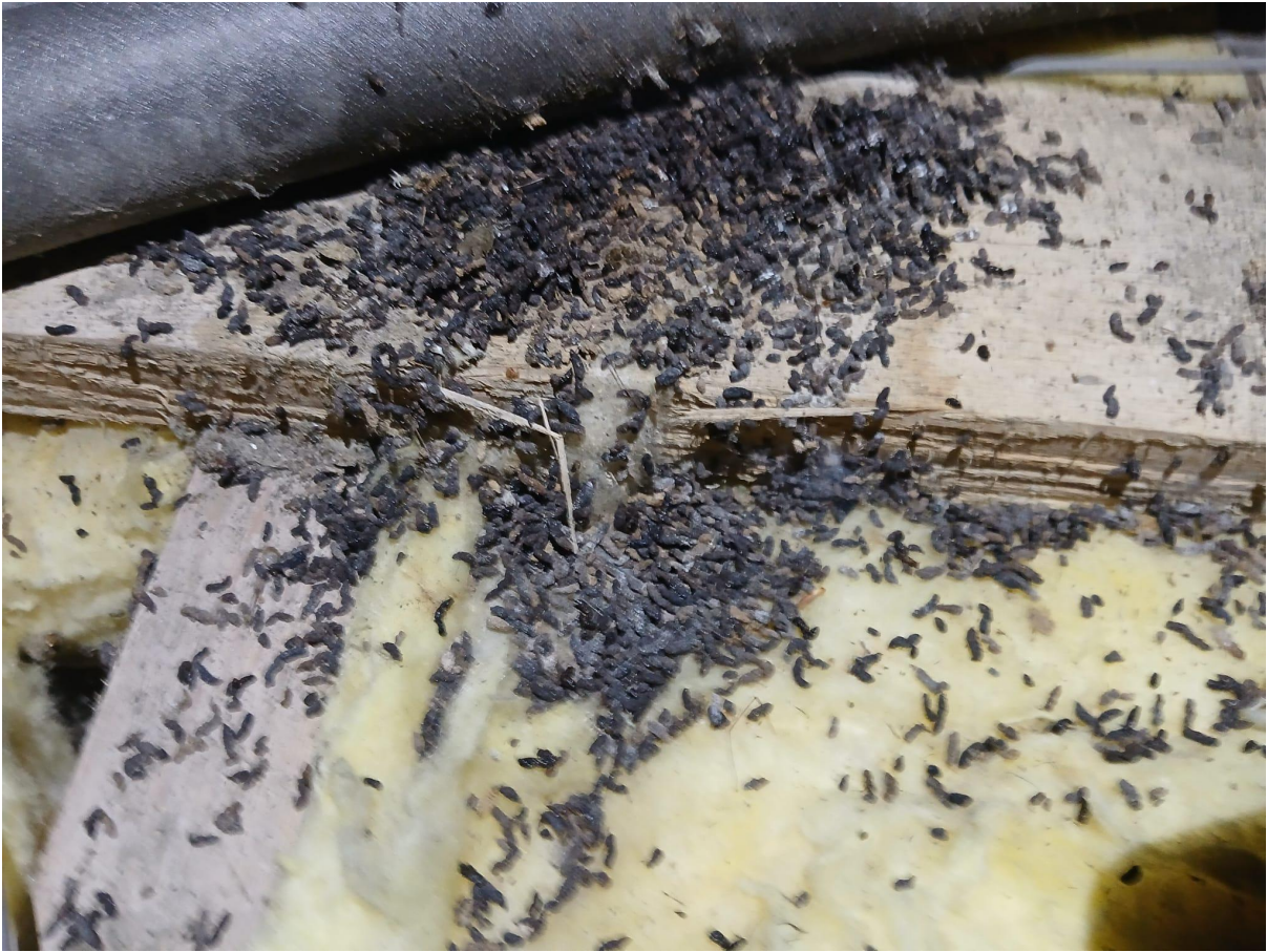
Figure 5. Significant piles of bat droppings.
