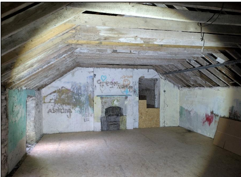
Plate 3-3. Loft level in southern-most section of subject building. Bat droppings recorded stuck to walls including above fireplace.
