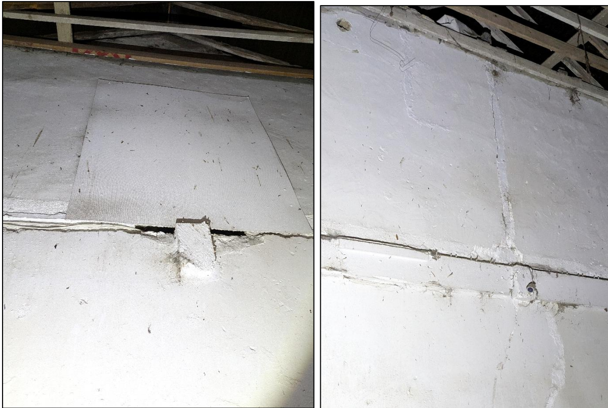
Plate 3-4. Example of bat droppings recorded on end walls in central open section of subject building.
