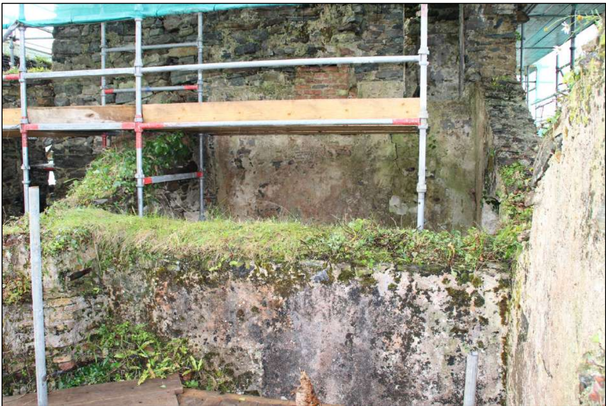
Pl. 28 Another view of the plastered walls of the attic spaces of the two kilns.
