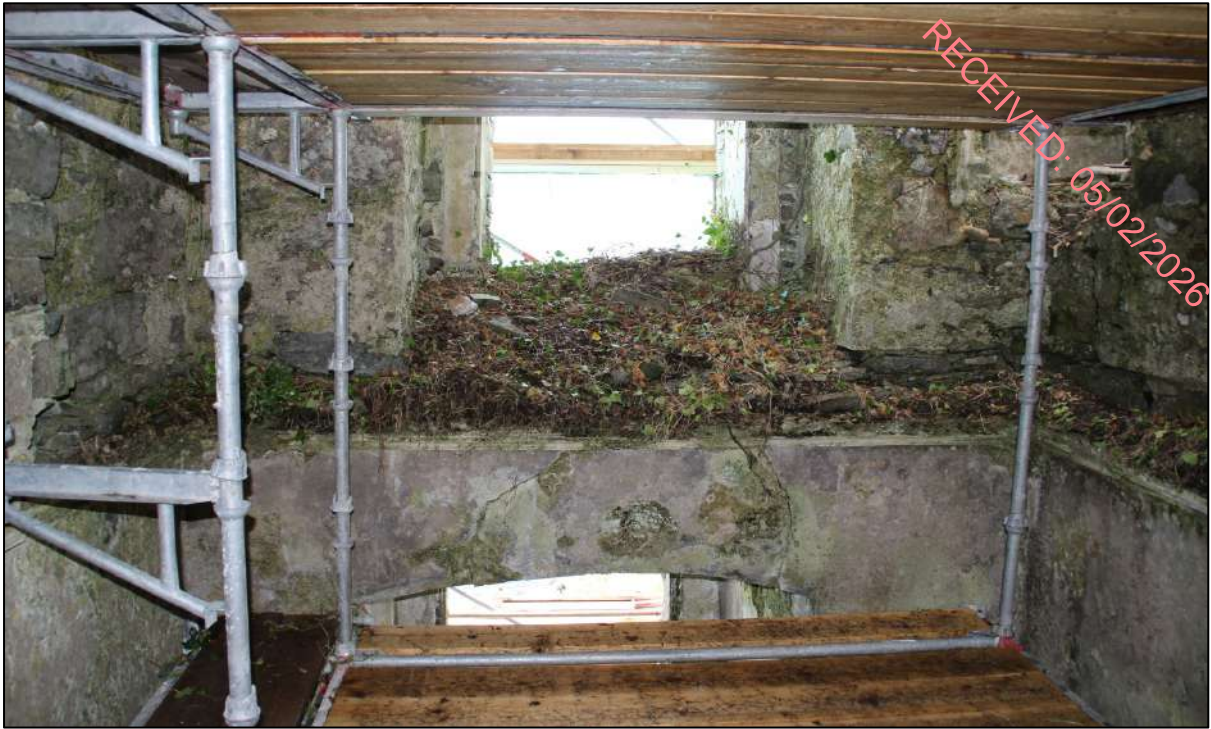
Pl. 8 The western side of the ground floor chamber. The coving on either side of the window survives in reasonable condition.
