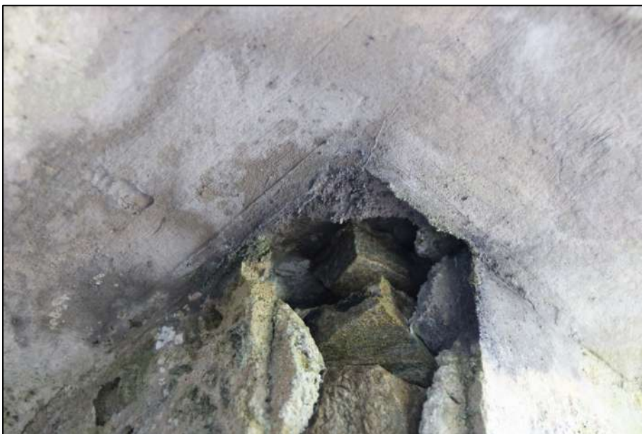
Pl. 24 Detail of corner beading, south side of western window embrasure, ground floor.
