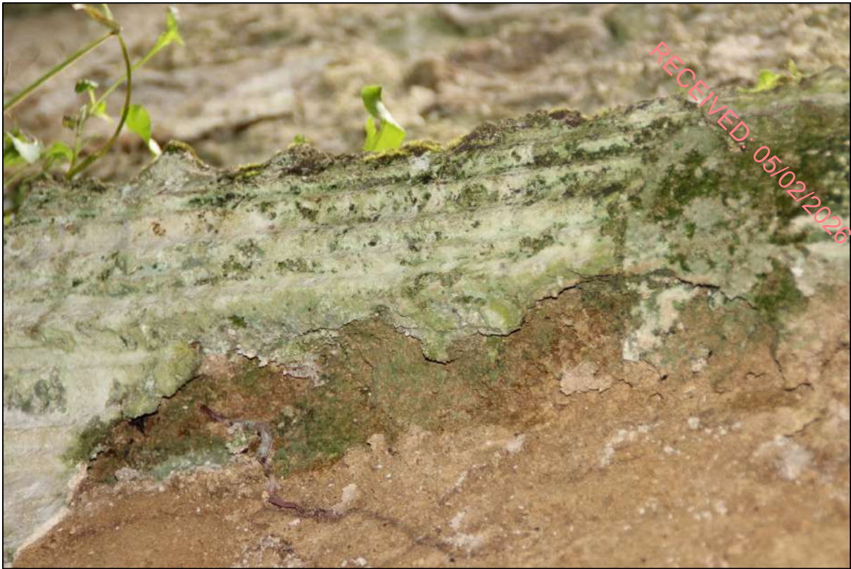
Pl. 4 Detail of coving on interior of eastern wall, entrance lobby. Note deterioration on right.
