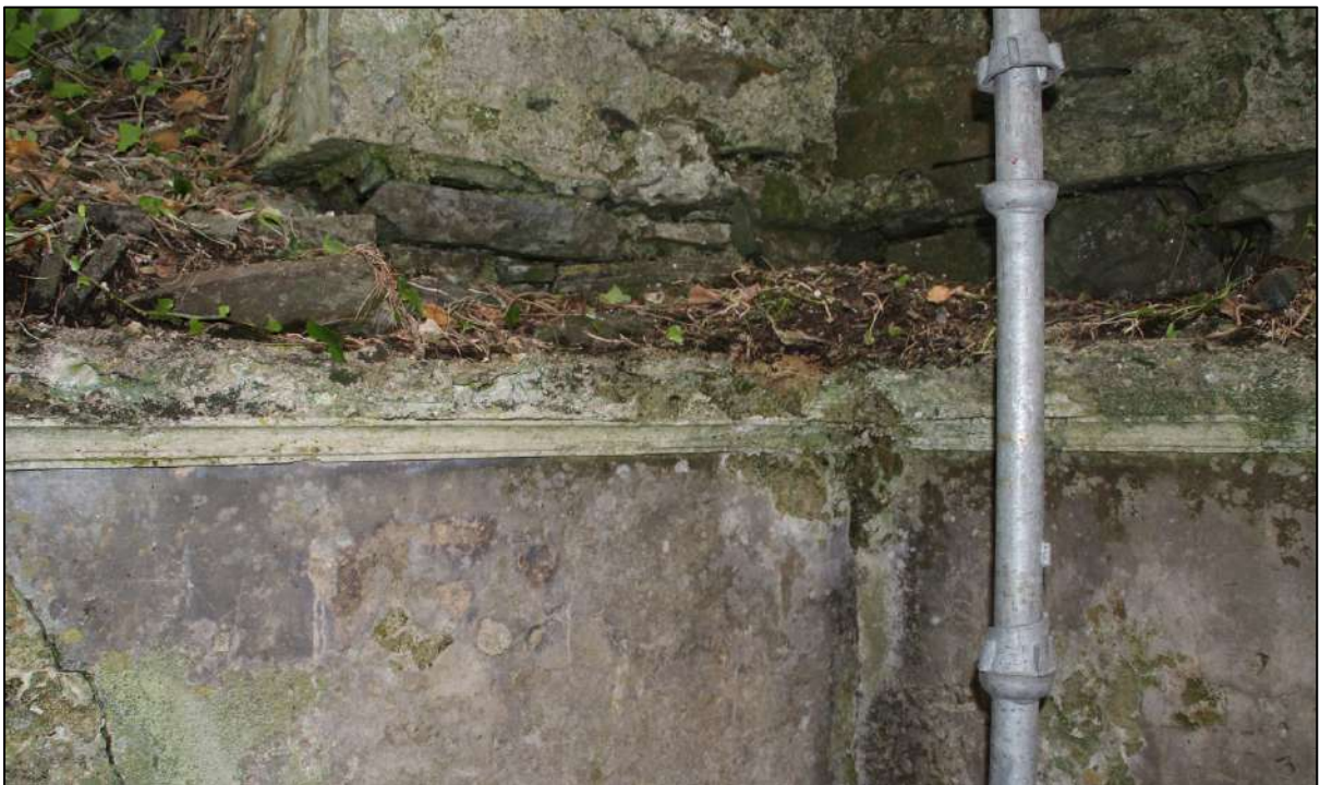
Pl. 15 Moulding detail in the north-west corner of the ground floor chamber. Note how the upper part of the moulding has fallen away.
