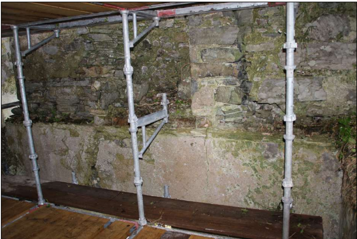
Pl. 7 The interior of the southern wall. The vertical masonry is infilling of the western side of the fireplace. The coving survives on the extreme right with the scratch coat evident elsewhere.
