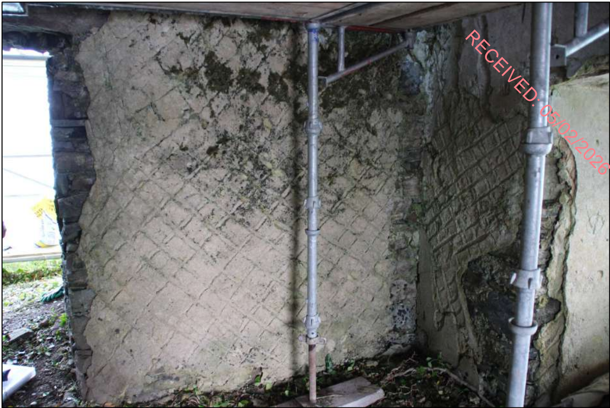
Pl. 16 The scratch coat that lay under the plaster top coat exposed, this finish can be seen on the southern window embrasure on the far right. East face of internal wall of tower house.
