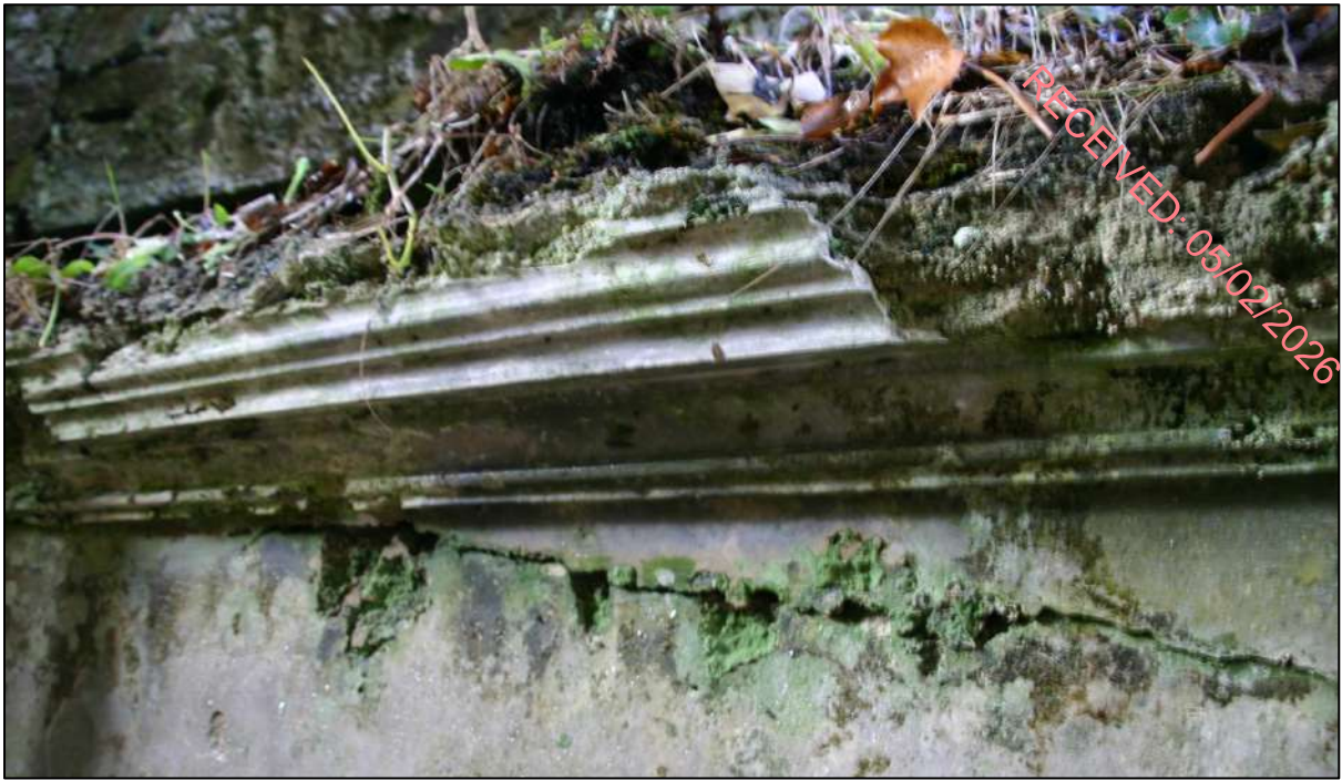
Pl. 10 Detail of the moulding on the northern wall, north-west side. Vegetation accumulates on the lip where the floor joists sat, this eventually leads to a deterioration of the plasterwork.
