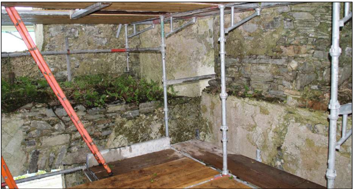
Pl. 9 Detail of south-east corner of the ground floor. The plaster line at right marks the level of the ceiling.
