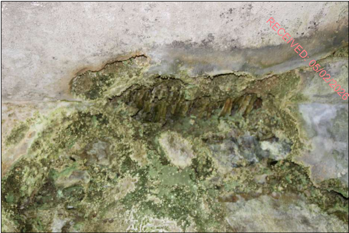
Pl. 25 Impression of wickerwork centring for head of embrasure, northern side of western window. This is the best example of this technique visible in the tower house. All examples occur in embrasures.
