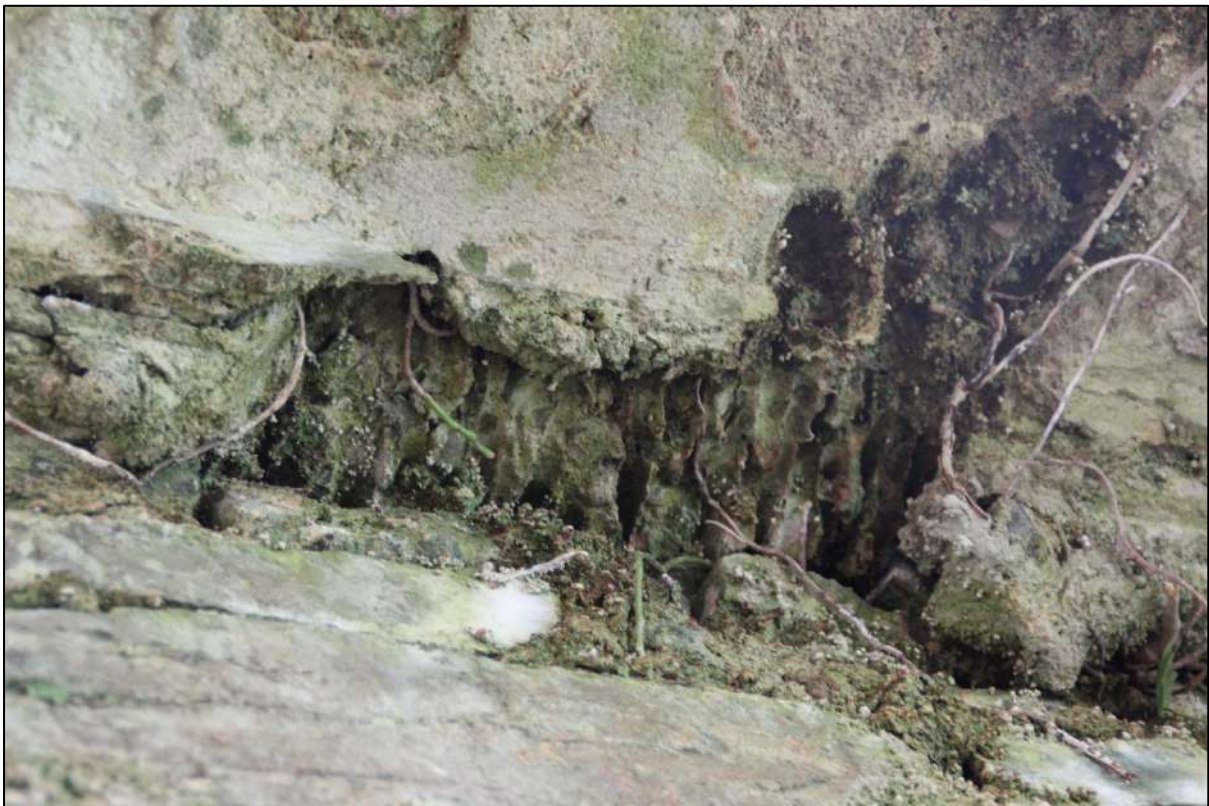
Pl. 26 Another example of the preservation of the impression of wickerwork centring for the window embrasure, in this case the southern side of the western window, first floor.
