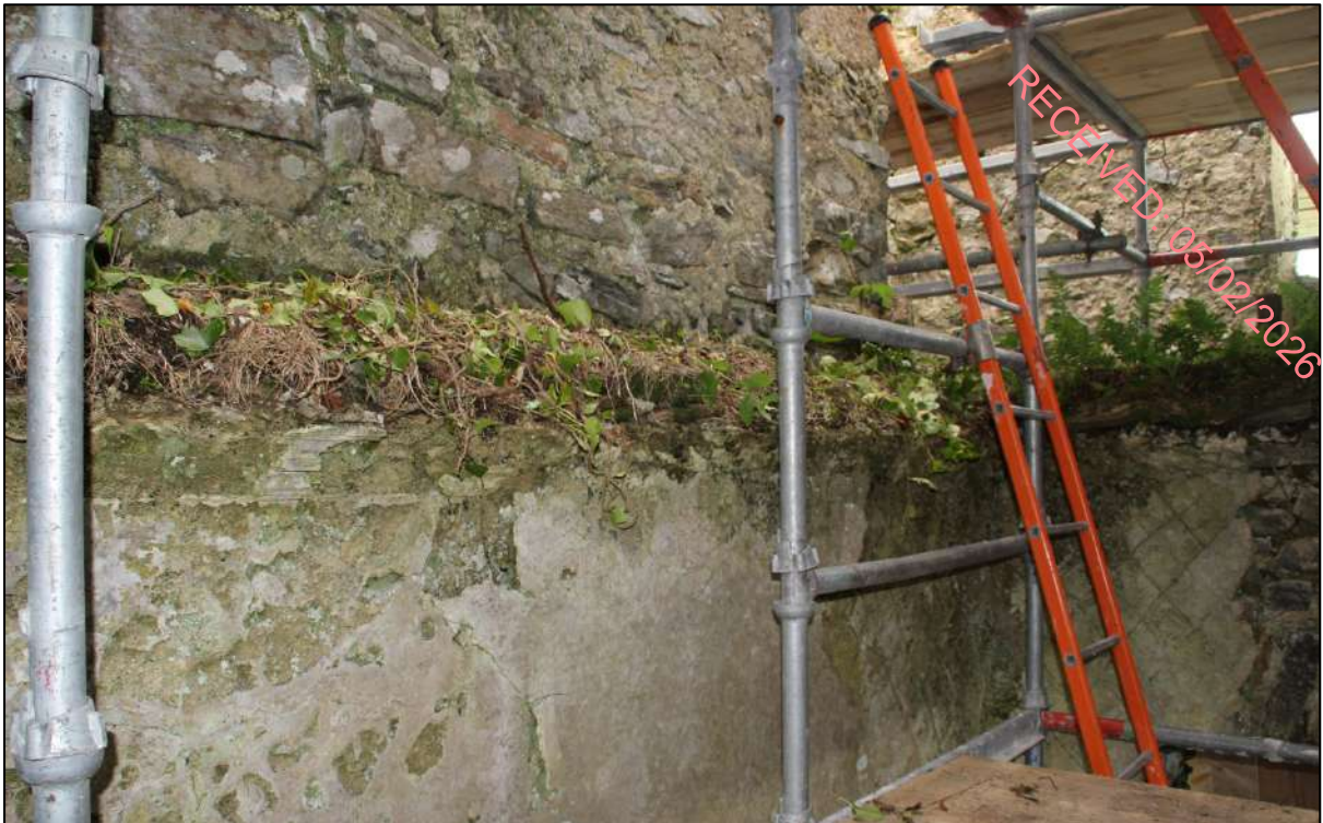
Pl. 14 The moulding on the northern wall of the ground floor chamber. Most of this is in poor condition.
