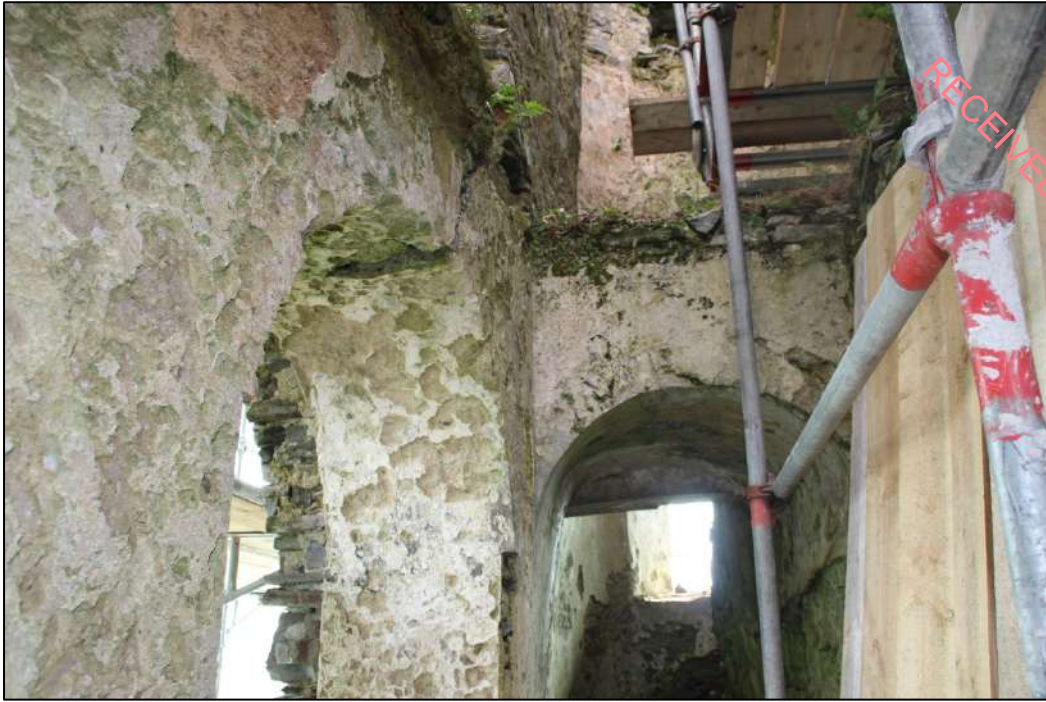
Pl. 2 Entrance lobby looking south. Coving has disappeared from wall over stairwell.
