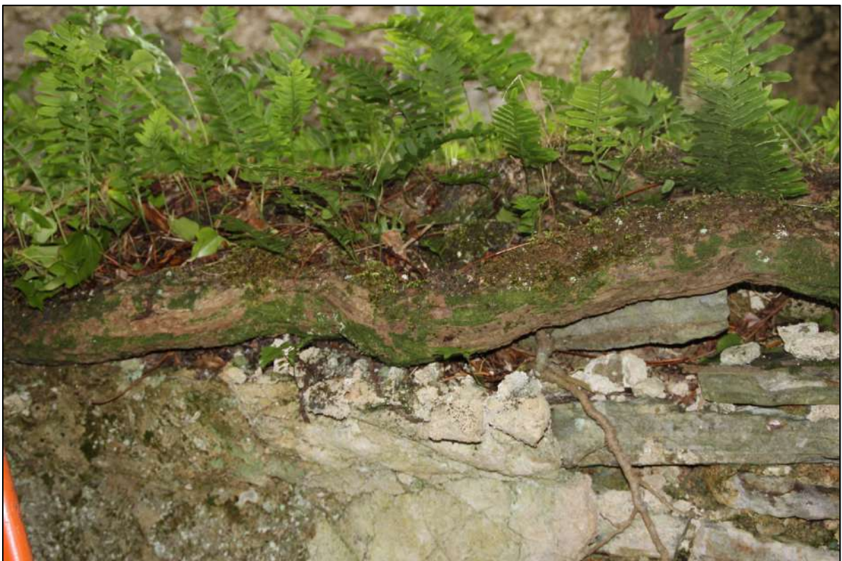
Pl. 11 Part of a tree trunk on top of the internal wall which separates the entrance lobby from the main chamber on the ground floor. The scratch coat base for the coving can be seen directly below the tree in the centre of the picture.
