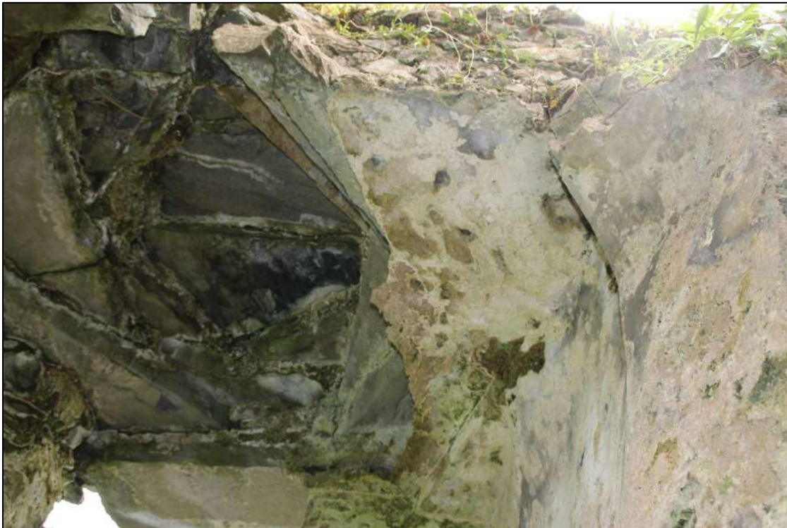
Pl. 19 The roof of the room containing the oriel window. This was entered through a doorway with an arched head, the remains of which are visible on right. There was a flat
