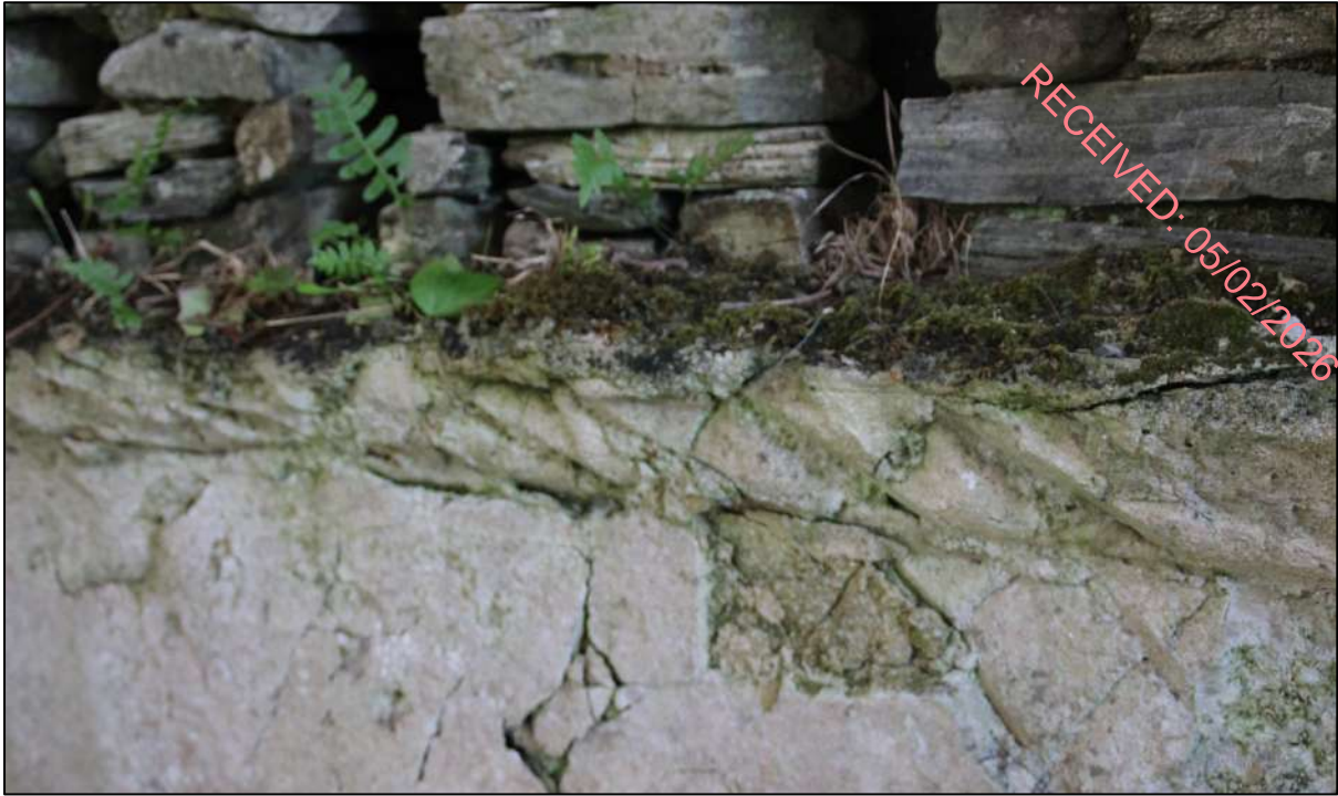
Pl. 12 Detail of the scratch coat band applied to give support to the decorative moulding. This is deeply scored to allow the plaster to grip. Southern wall, ground floor.
