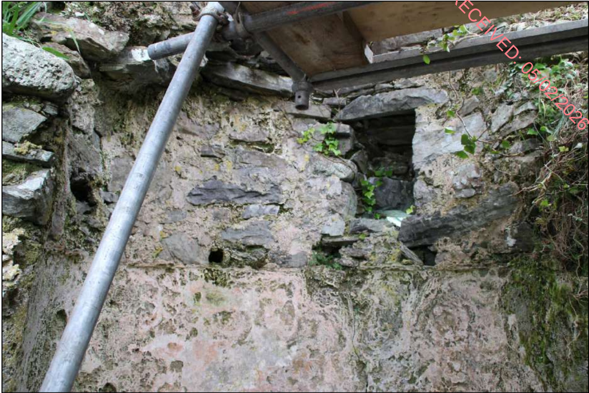
Pl. 18 The upper part of the stairwell. Note the plaster coat on the lower part of the photograph. The small holes held the timbers that supported the ceiling. The small opening is likely to be associated with the late-medieval occupation of the tower house.
