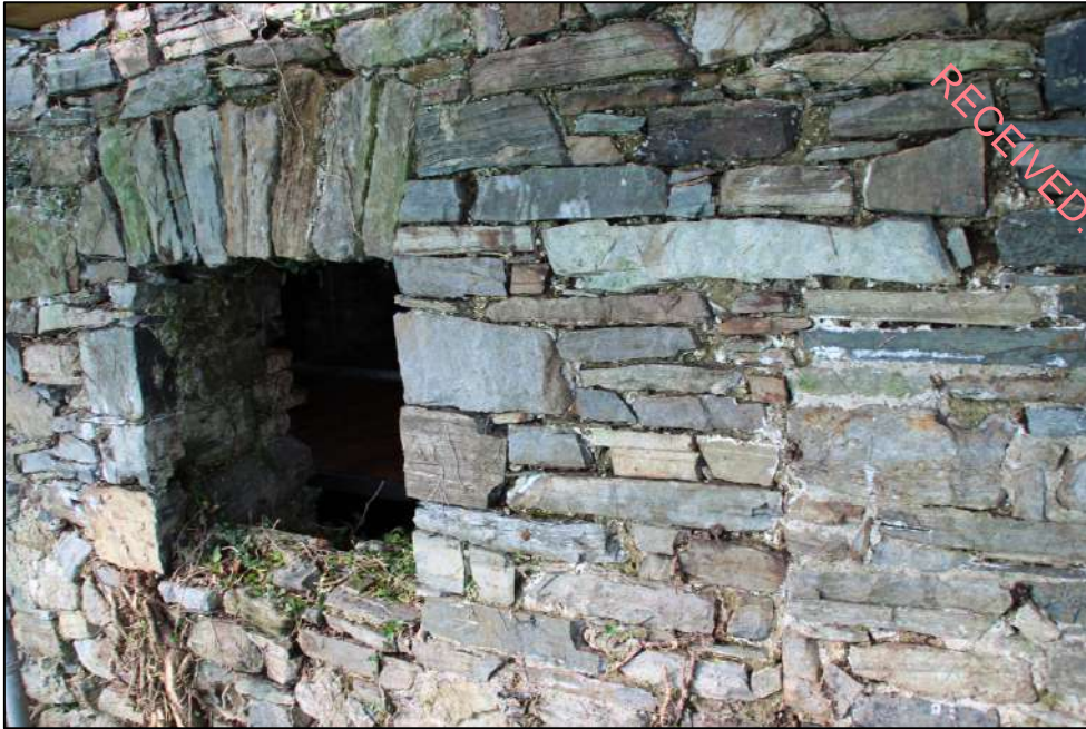
PI. 105 Window on the ground floor of the eastern side of the industrial building. The vertical break in the masonry on the right of the window, indicates that a slit opening was going to be placed here with the linear pale stone forming its lintel.
