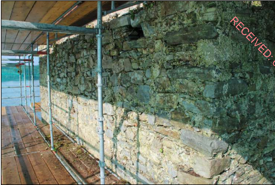
Pl. 39 The upper part of the southern elevation. Note the remnants of the external mortar finish
