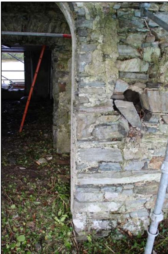
Pl. 5 Northern side of doorway. Note void.
