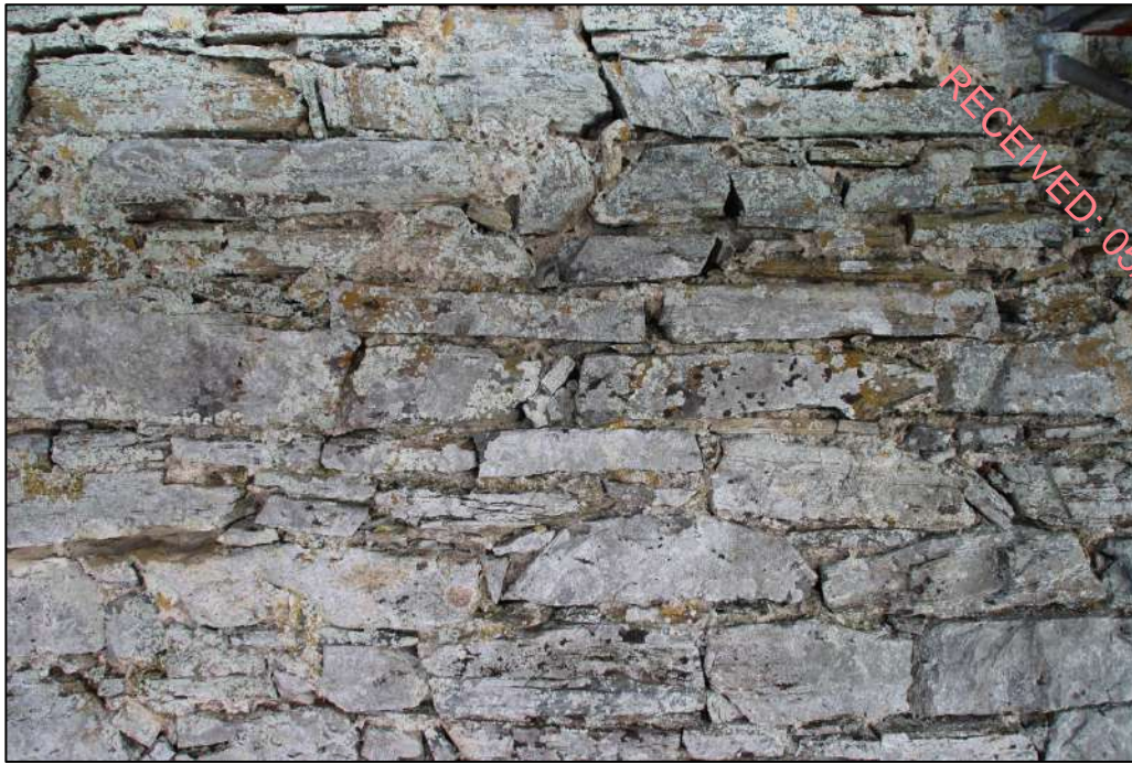
PI. 29 A thin render coating is present on parts of the tower house.
