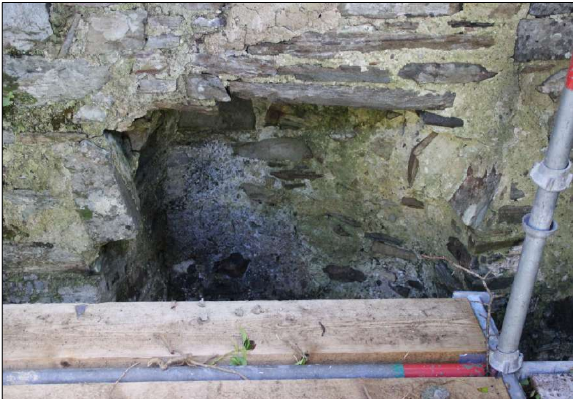
Pl. 125 The fireplace on the exterior of the northern wall of the tower house. This is in the large room of the industrial building. A single rough stone voussoir can be seen on either side of the top of the feature. Note how the right hand side of the fireplace is shallower in depth than the other side, giving an uneven appearance.
