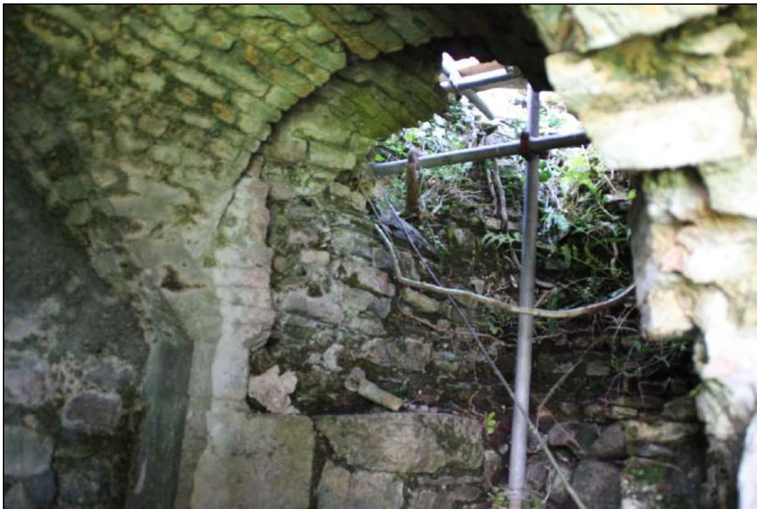
Pl. 140 The upper part of the drawing hole arch has collapsed. This was built of brick with ashlar masonry used for the lower part.
