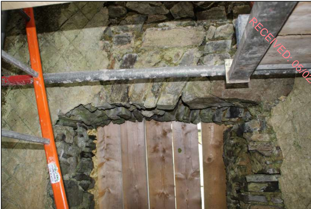
Pl. 50 The doorway leading to the entrance lobby from the main chamber of the ground floor.
