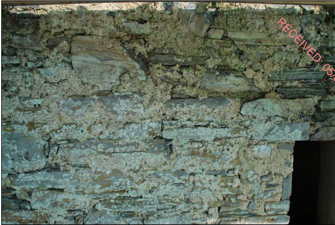
Pl. 41 Remnants of the mortar finish by the stairs window, southern elevation.
