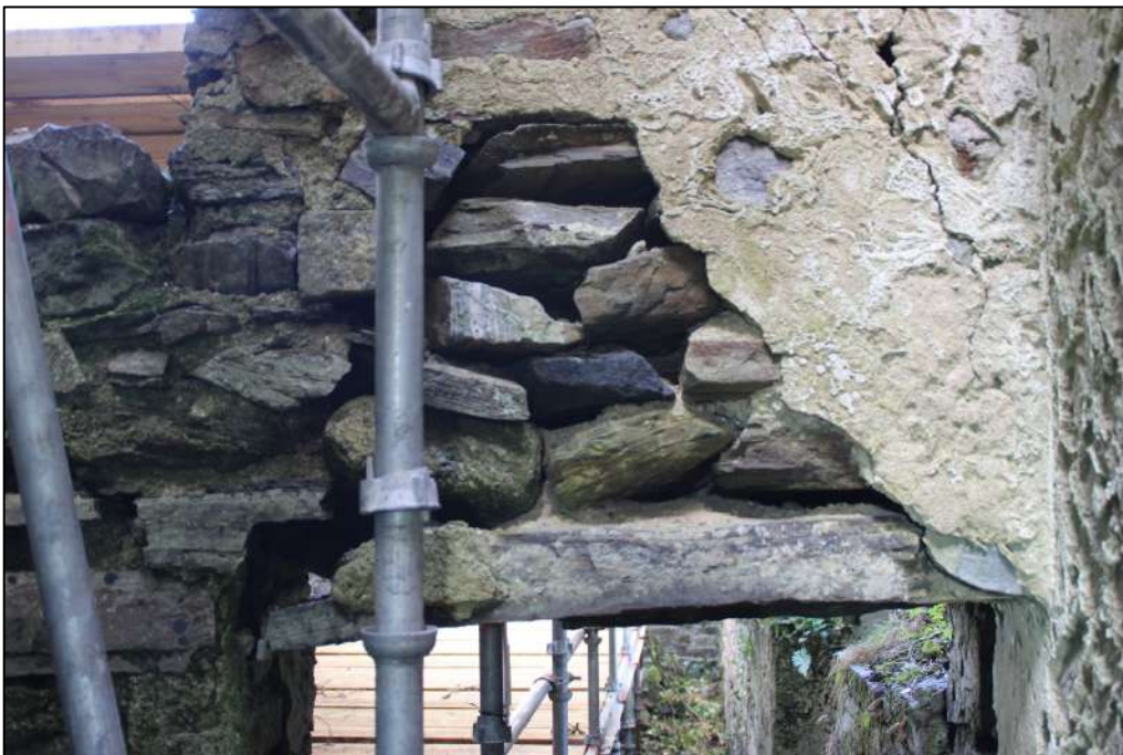
Pl. 47 This is the structurally weak lintel over the door leading from the entrance lobby of the tower house into the industrial building. The wall overhead was rebuilt when the north-east corner was altered.
