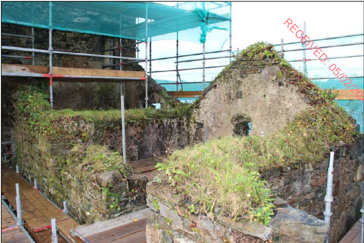
Pl. 146 The gabled form of the roof over kiln 2 can be seen here.
