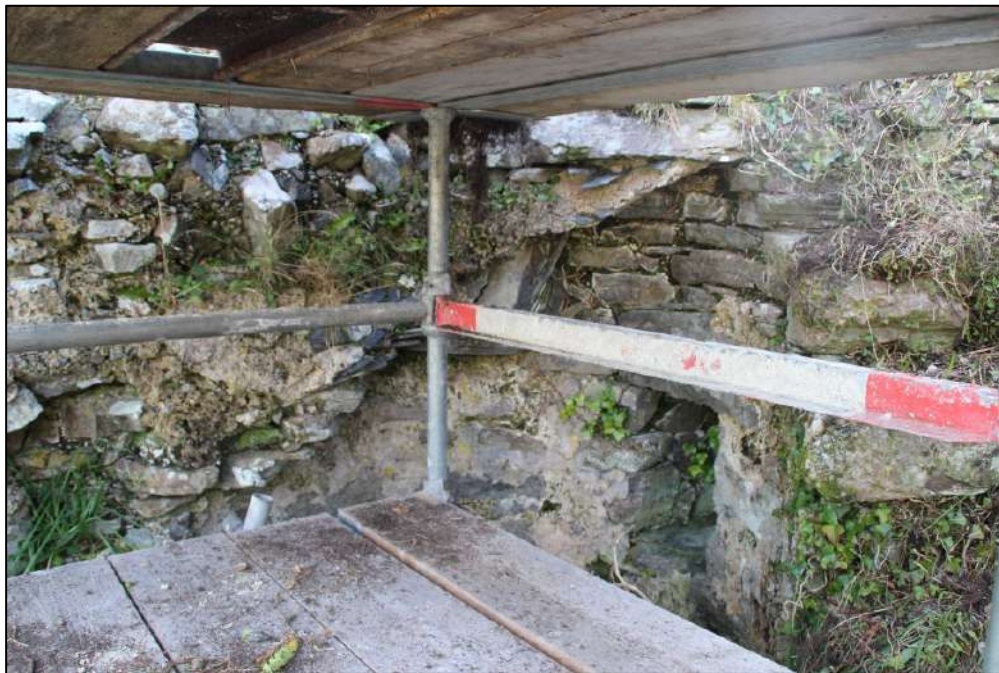
Pl. 103 The northern side of the stairwell roof cap. The sloping line of stones marks the break between the stairwell with the smooth faced masonry and the window opening forming the uppermost part of the stairwell.
