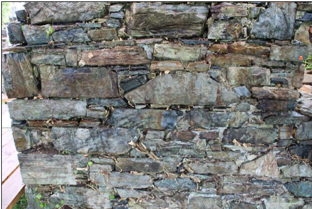
PI. 115 Masonry of the first floor of kiln 2. This is a later addition to the industrial structures on the island.
