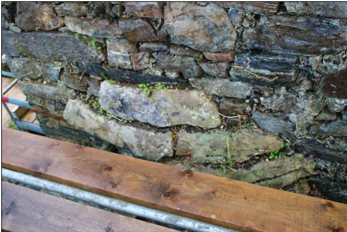
PI. 24 The hood over the window on the north-western corner is the most intact.
