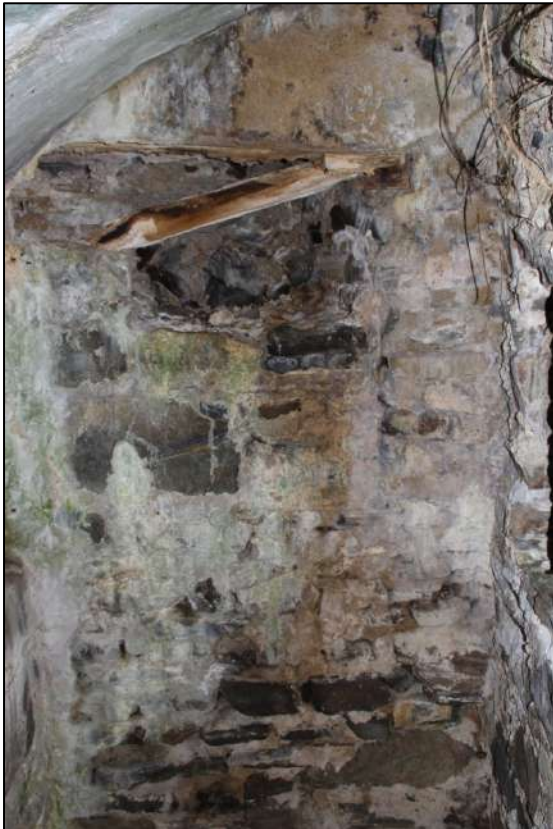
Pl. 131 The front of kiln 1 showing the access opening to the rear of the kiln. This appears to have been the only means of getting into this space.
