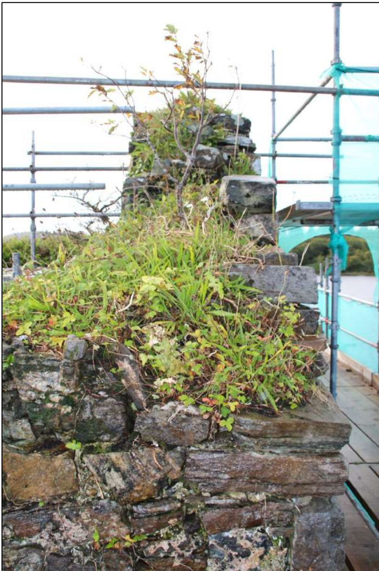
Pl. 20 The northern side of the western gable prior to final trimming of vegetation.
