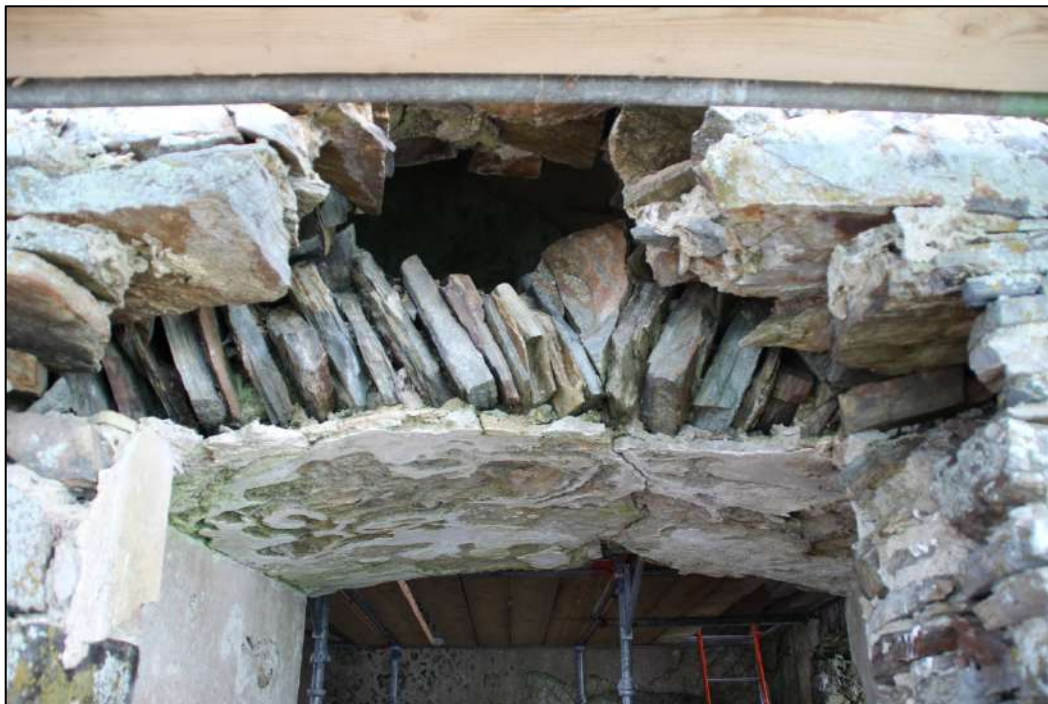
Pl. 34 The hole over the window head. Very little mortar is present.
