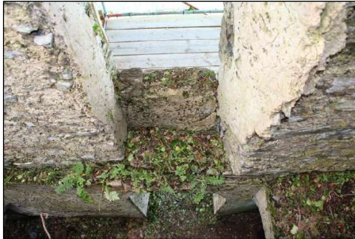
Pl. 77 Note the difference in thickness between the later wall on the left and the medieval fabric on the right.
