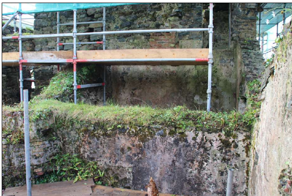
Pl. 145 The gabled single pitch form of the roof over kiln 1 can be seen here. The manner in which the roof crosses the lower part of the northern 'oriel' window on upper right is unusual as no trace of any blocking material is present.
