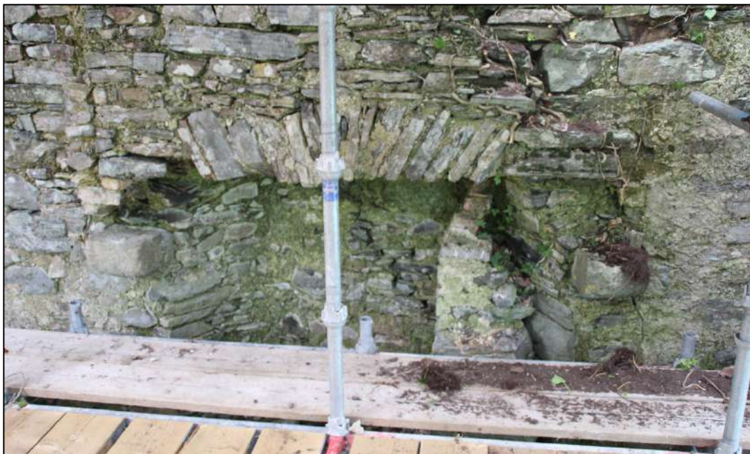
Pl. 81 The upper part of the fireplace. The corbels on either side would have supported a timber lintel. The masonry to the right of centre was inserted to reduce the width of the feature at a later date.
