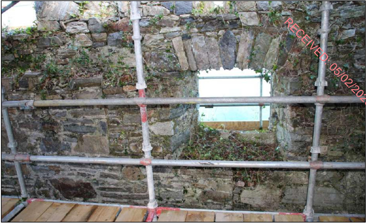
Pl. 124 Inner side of the eastern elevation of the industrial building, ground floor. The infilled masonry area on the left is where a slit window was constructed but changed in favour of the larger window opening.
