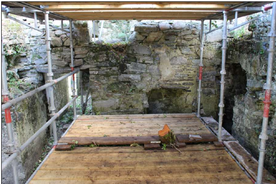
Pl. 118 View of the southern end of the large (eastern) room of the industrial building. The doorway on the left leads into the tower house lobby, that on the right leads to kiln 1. The fireplace just right of centre appears to be inserted. The doorway in the top of the photograph is part of the later rebuilding of the north-eastern corner of the tower house.
