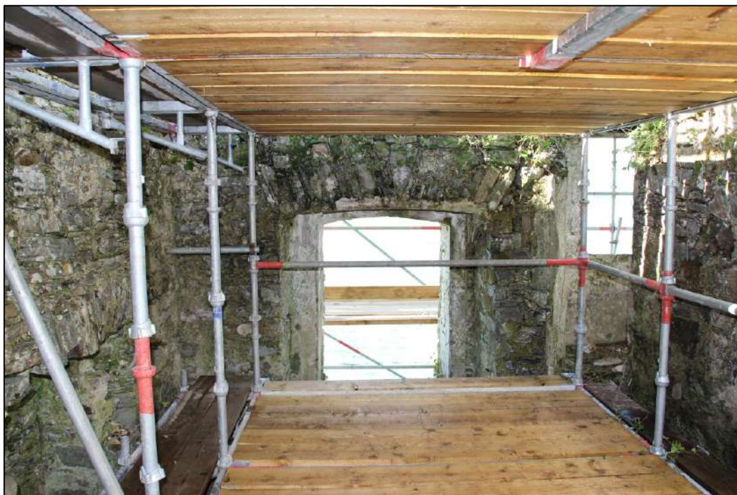
PI. 79 The first floor chamber looking west. Note the 'oriel' chamber on right.
