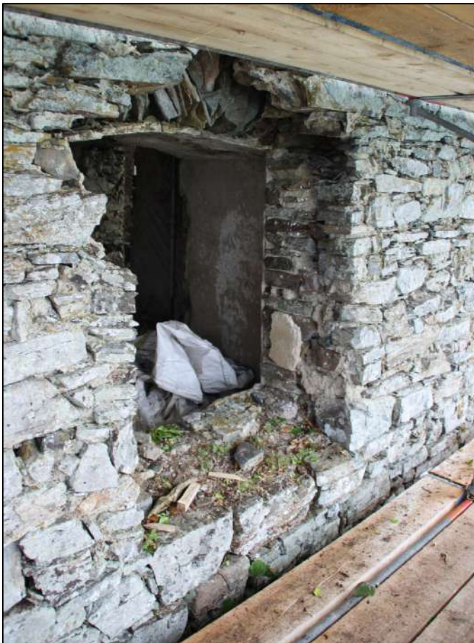
Pl. 32 This is the ground floor window on the southern side of the tower house. The collapse of the masonry head has resulted in a small hole appearing in the floor of the garderobe passageway.
