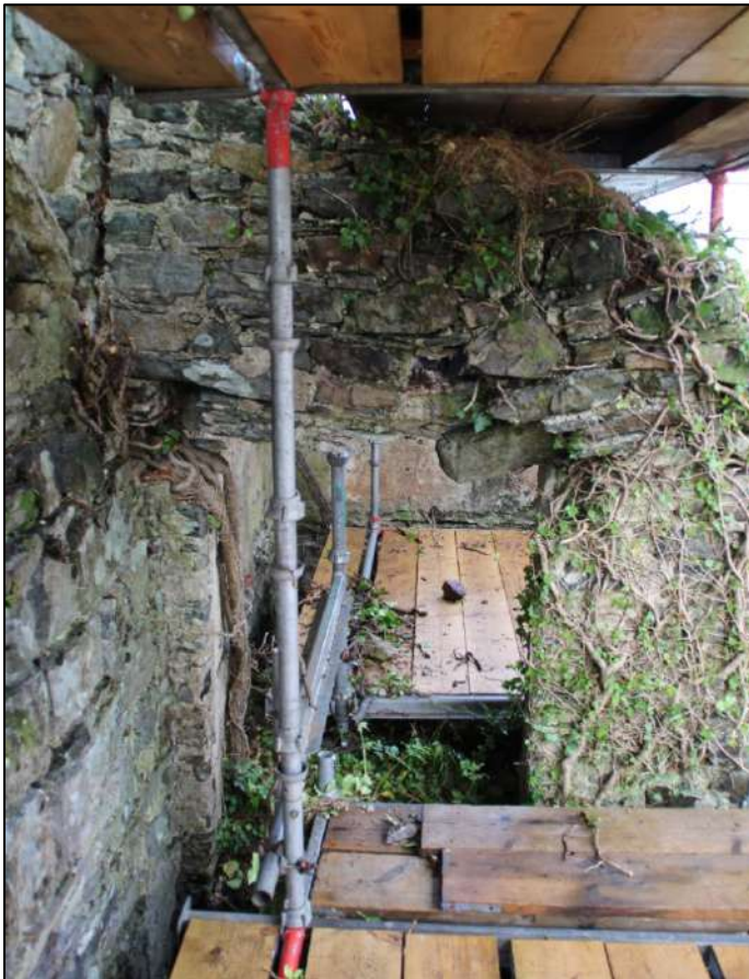
PI. 135 The space at the rear of kiln 1. The lower part of this has not been plastered while the floor above has been plastered. The floor line is evident.
