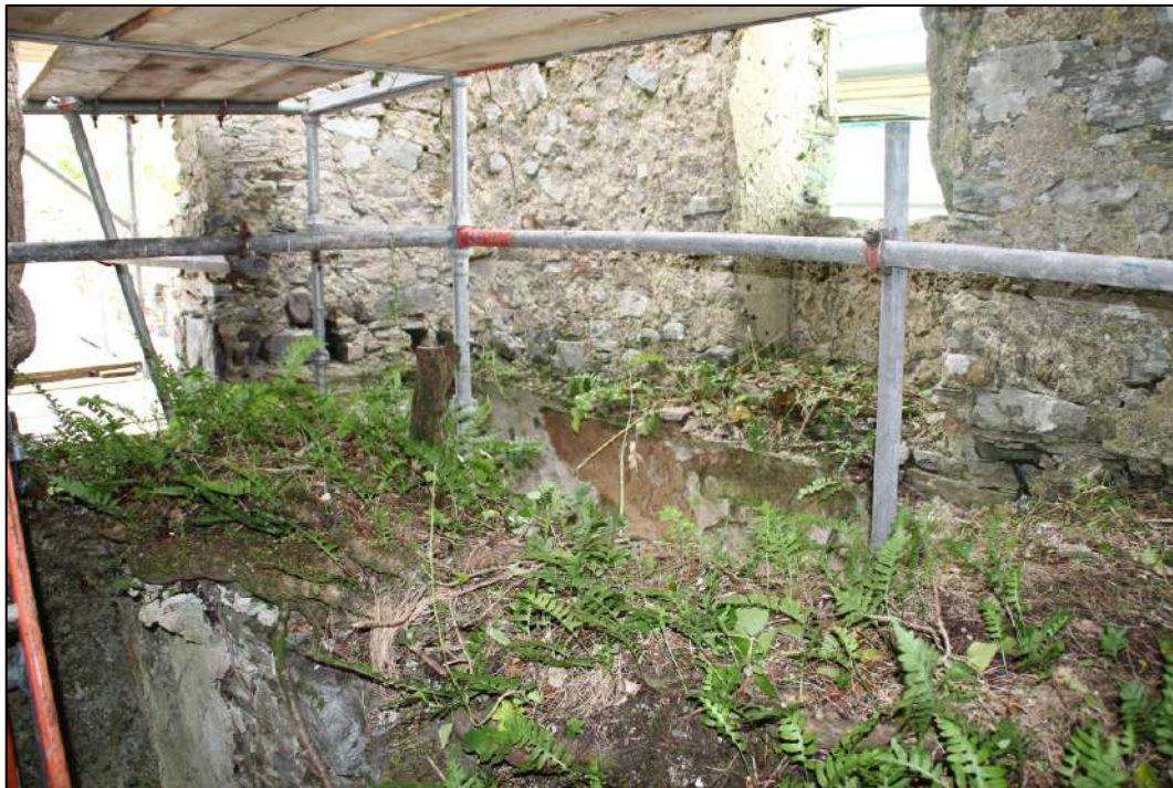
Pl. 73 The location of the first floor lobby. It is presumed that there was some form of partition separating this from the main room at this level.
