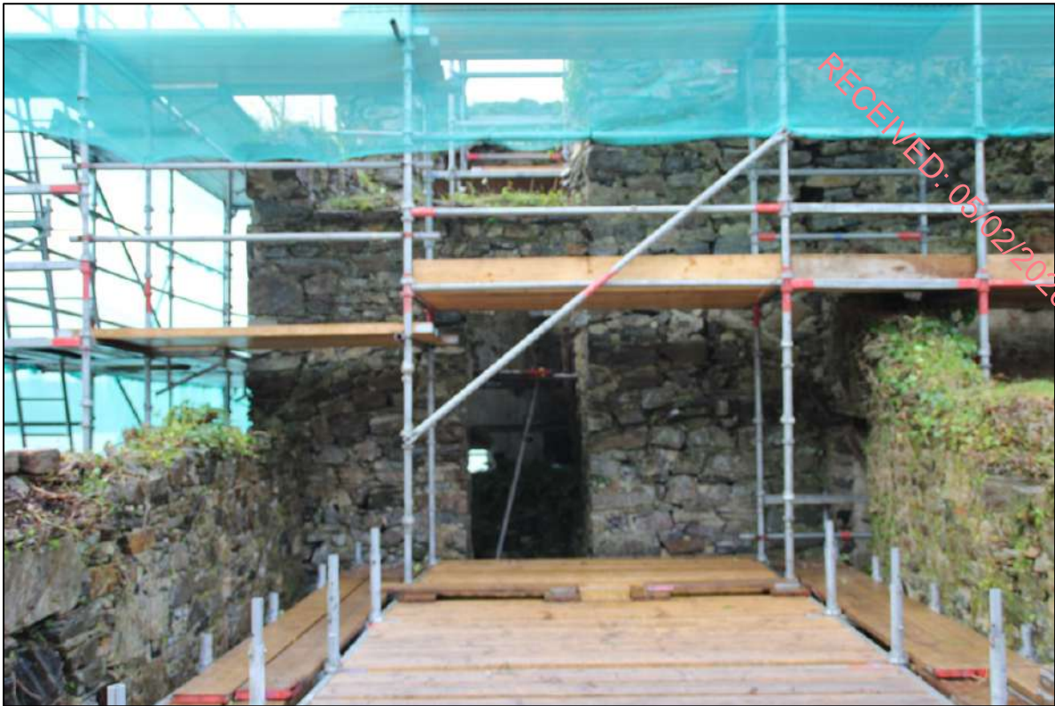
Pl. 129 The southern end of the first floor. The doorway leads to the first floor lobby of the tower house. All of the north-eastern (left hand side of the doorway) corner has been rebuilt. Note the mortar scar running from the tops of the walls of left and right to just over the doorway.
