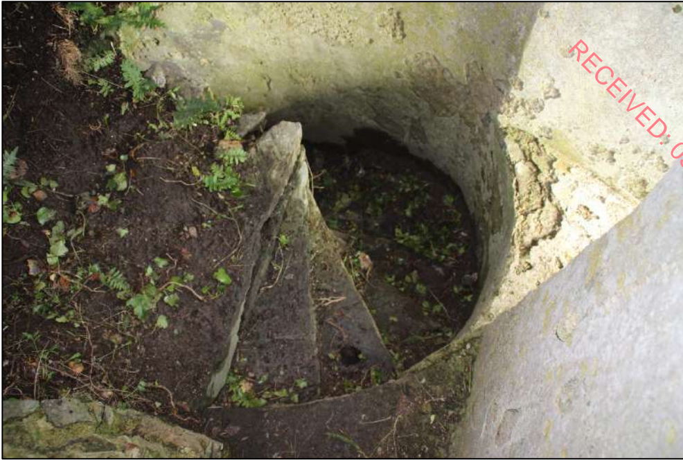
Pl. 62 The spiral stairs. It enters the first floor lobby on the far left.
