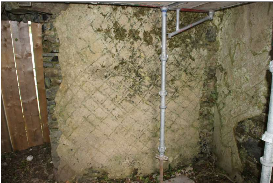
Pl. 51 Much of the plaster coat has fallen off the eastern and southern walls of the main room of the ground floor revealing a prominent scratch coat.
