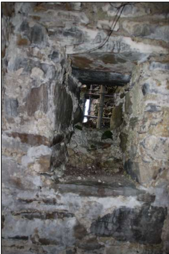
Pl. 134 Small window or opening looking out into the large room of the industrial building from kiln 1.
