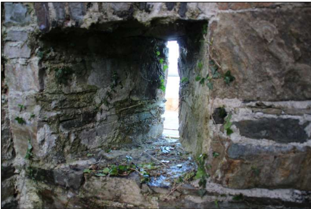
Pl. 123 Interior of the northernmost slit window of the eastern elevation, ground floor of the industrial building. Note the wide splay to allow the maximum amount of light.
