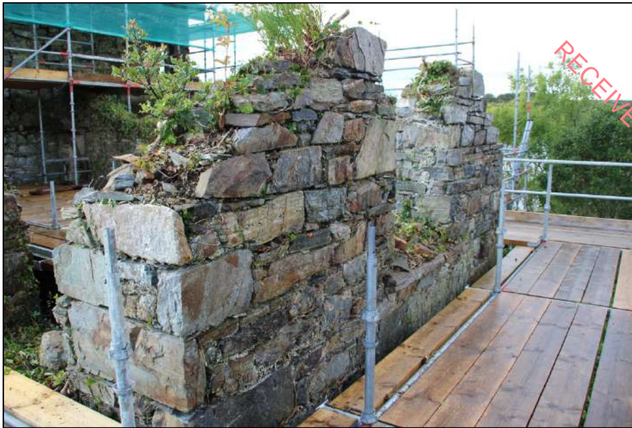
Pl. 112 Northern end of the eastern side of the industrial building. This had a gabled end with a large central window.
