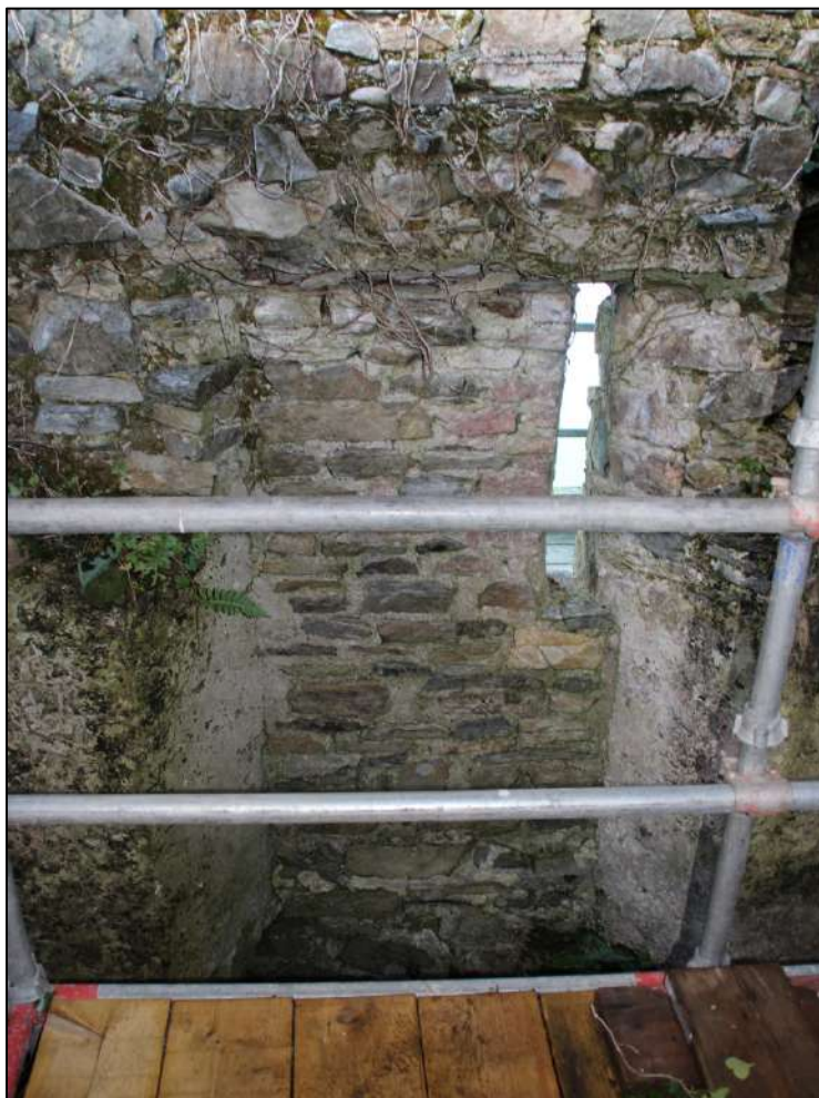
Pl. 120 The interior of the blocked doorway on the eastern wall of the southern end of the large room of the industrial building. This was adapted as a slit window.
