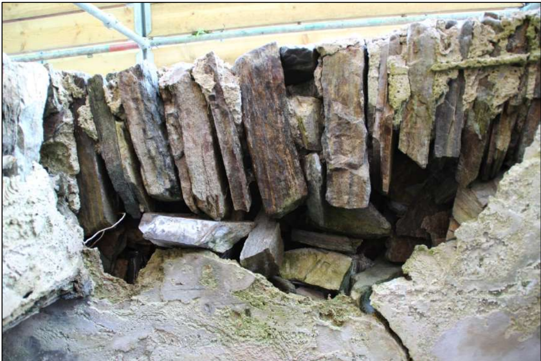
Pl. 49 The underside of the window head, western window, ground floor. This has lost much of its mortar bonding.
