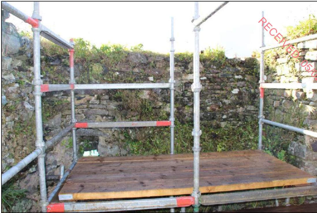
Pl. 102 View of the second floor looking east. The irregular masonry on the centre right of the photograph marks the location of the roof cap of the stairwell.
