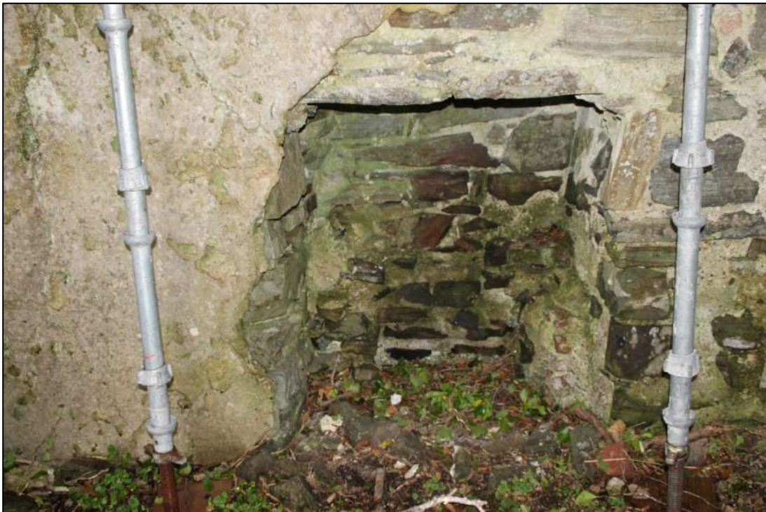
Pl. 57 Close up of the fireplace. Note the two voussoirs of the arch that spanned the feature.
