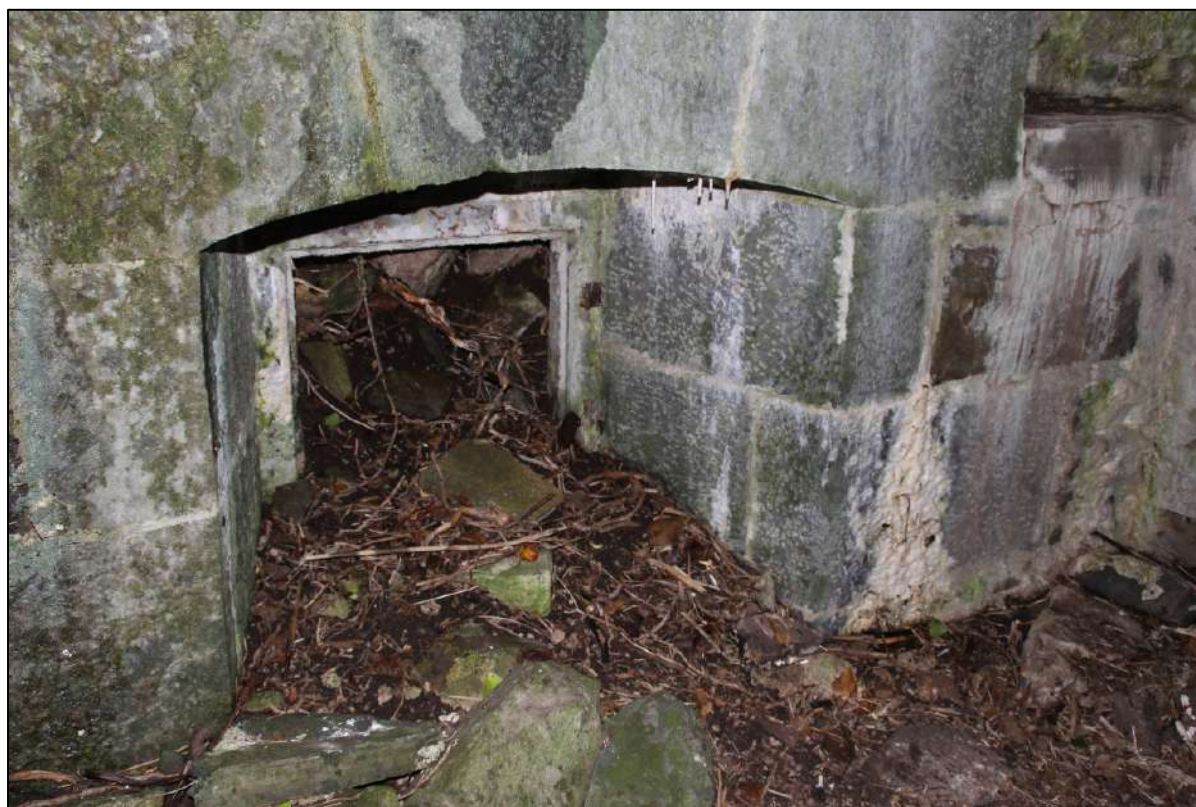
Pl. 130 Kiln 1 looking at the drawing hole. Two iron hinges are present on the right hand side of the inner doorway. The poking hole in inner part of the kiln is full of debris. The quality of the masonry here is excellent. At the top right can be seen the access opening to the back of the kiln.
