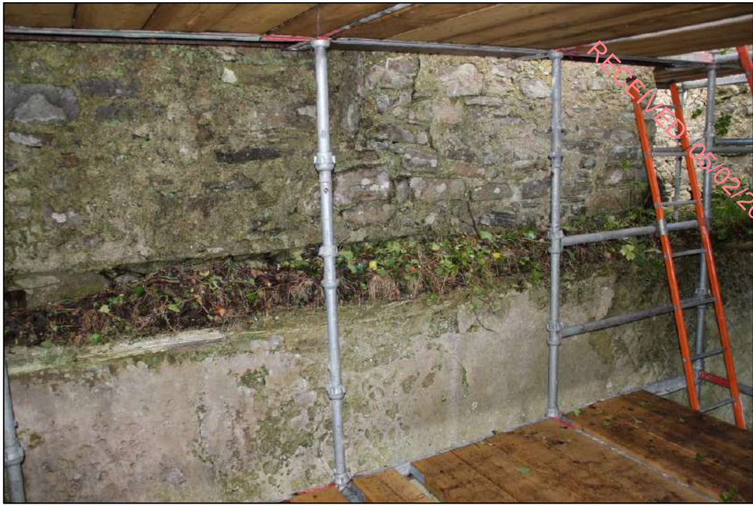
Pl. 58 The ceiling level is marked by the lower edge of the band crossing the centre of the photograph. This is where a shallow lip held the joists of the floor. A small part of the decorative moulding can be seen on the left. It has collapsed in the middle and right of the picture.
