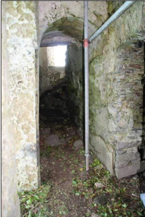
PI. 44 The stairs on the southern side of the entrance lobby. Many of the examples of graffiti on the site are on the left hand wall.
