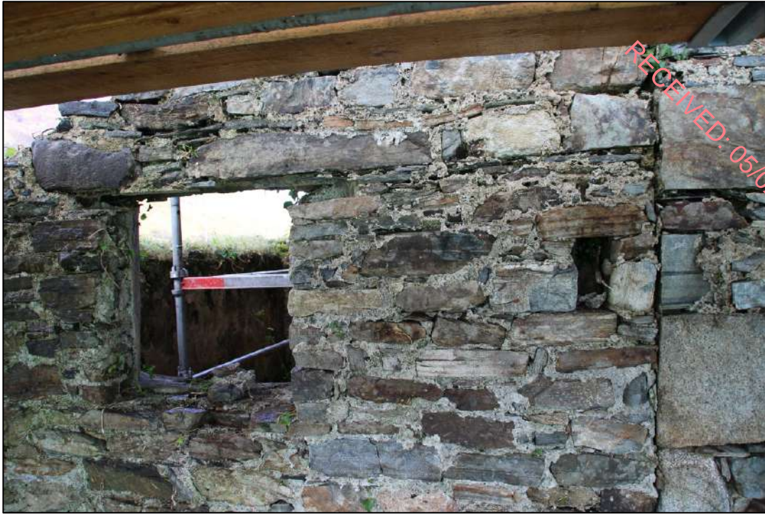
Pl. 116 The window of the first floor room over kiln 1, the first kiln on the site. The wall on the far right of the photograph is that of the tower house. The rectangular slot may be a putlog hole with another possibly present on the left hand side of the window, out of picture.
