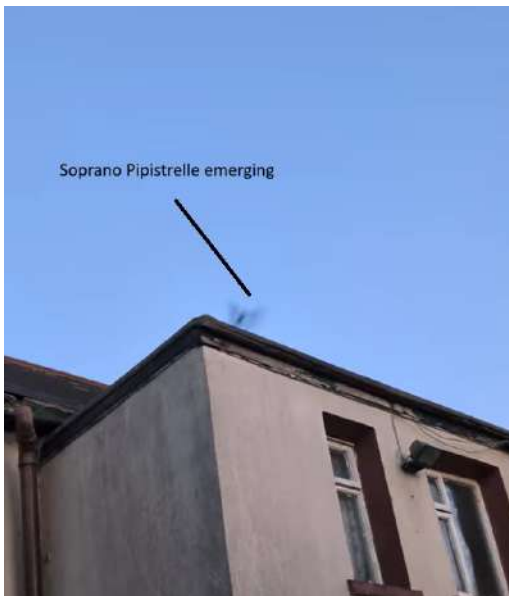
Figure 4. Bat emerging from fascia on flat roof extension at rear of dwelling
