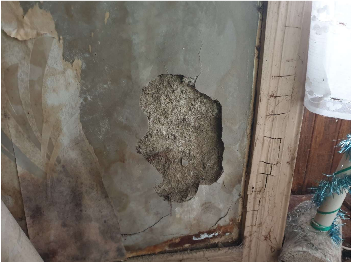
Plate 40: Detail of cubic rot and gypsum delaminating plaster to external wall.
