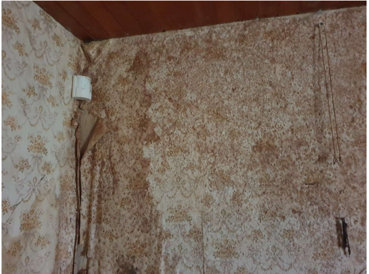
Plate35: Detail of damp to walls
