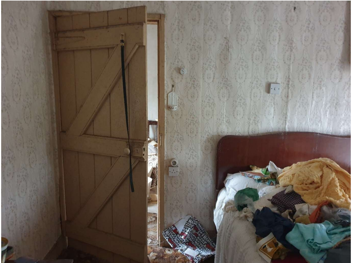
Plate 43: Detail of typical door to first floor bedrooms. Note timber sheeting to walls over papered.
