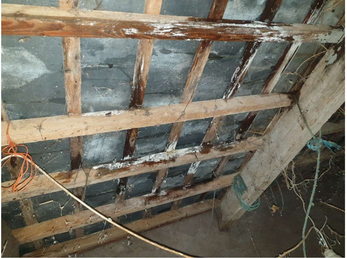
Plate 56: View of rotting and water damaged roof structure to Building C
