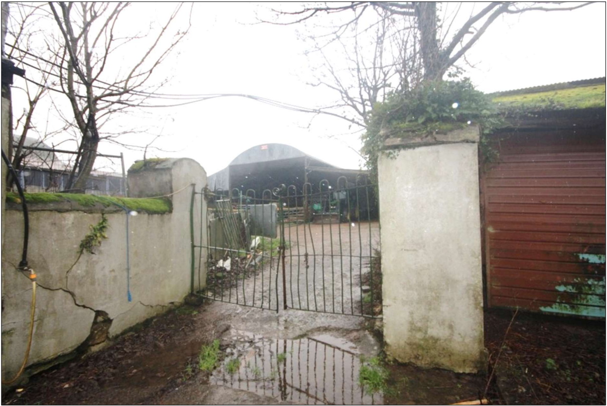
Plate 10: Piers and gateway to rear farmyard to be repaired and made useable.
