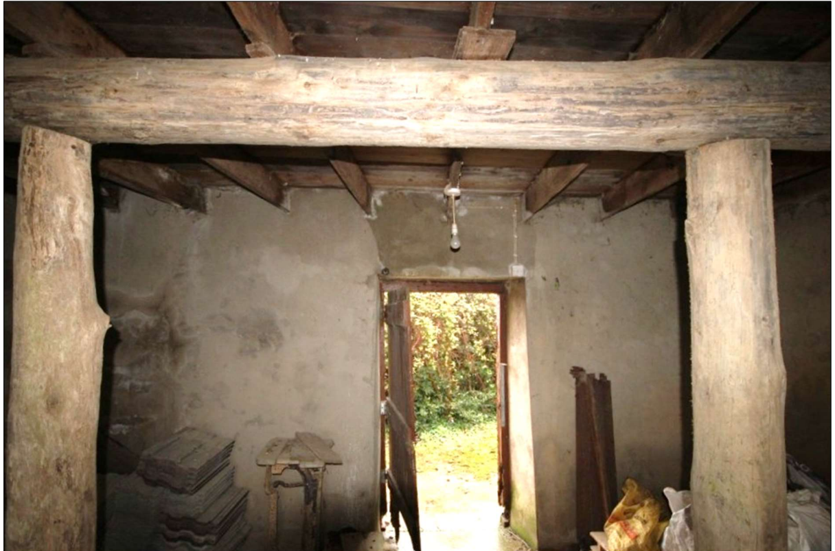
Plate 47: Interior of eastern bay of Building B. Note round post column and support beam to reinforce the floors above .Joists built into walls each end.
