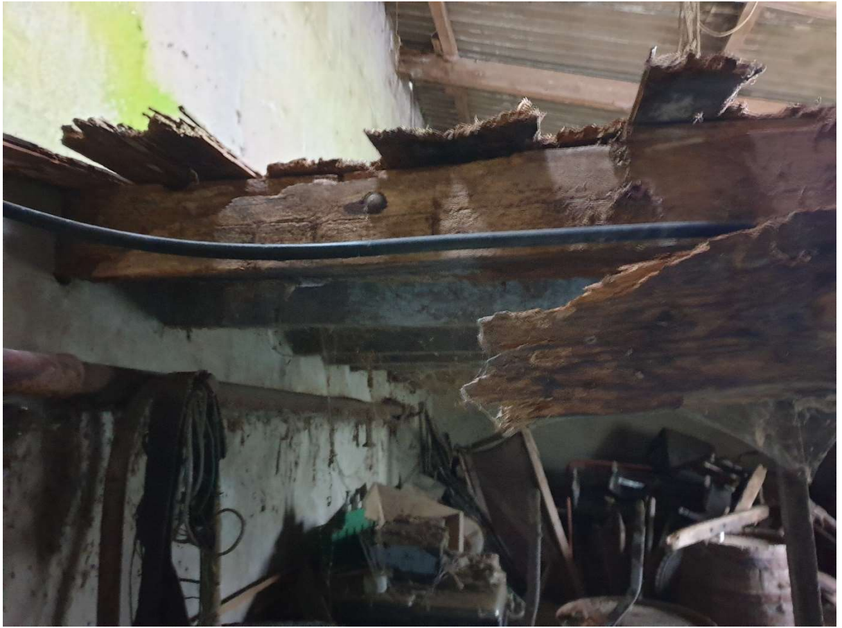
Plate 50: Detail of collapsing floor to Building B -Barn attached to main house.
