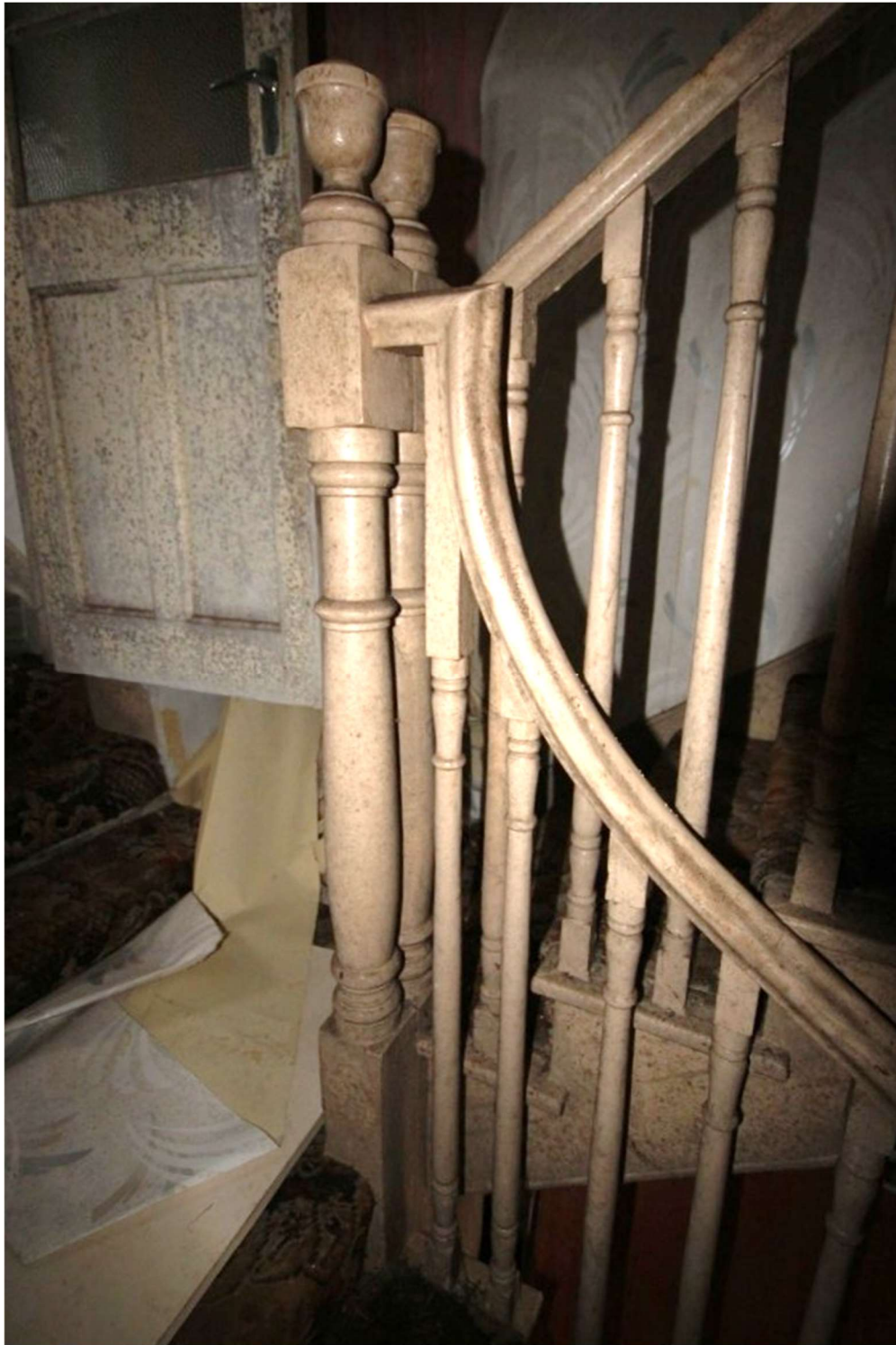
Plate 22: Ramped handrail and double newel to staircase on half landing. Stairs in good condition except mid landing collapsing most likely due to wood worm on supports. No access was made to inspect underneath.
