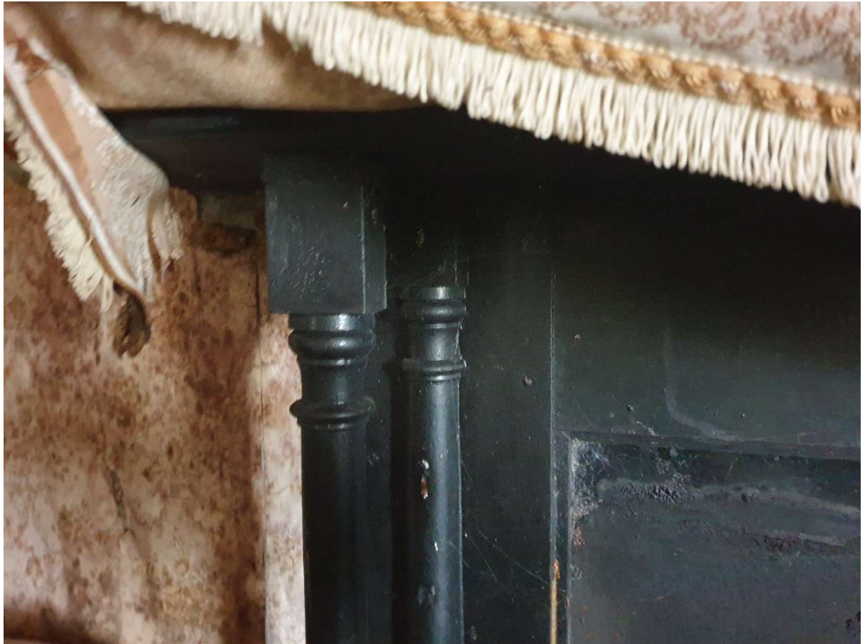
Plate 41: Detail of engaged and free standing timber support columns to fire surround to Living room.
