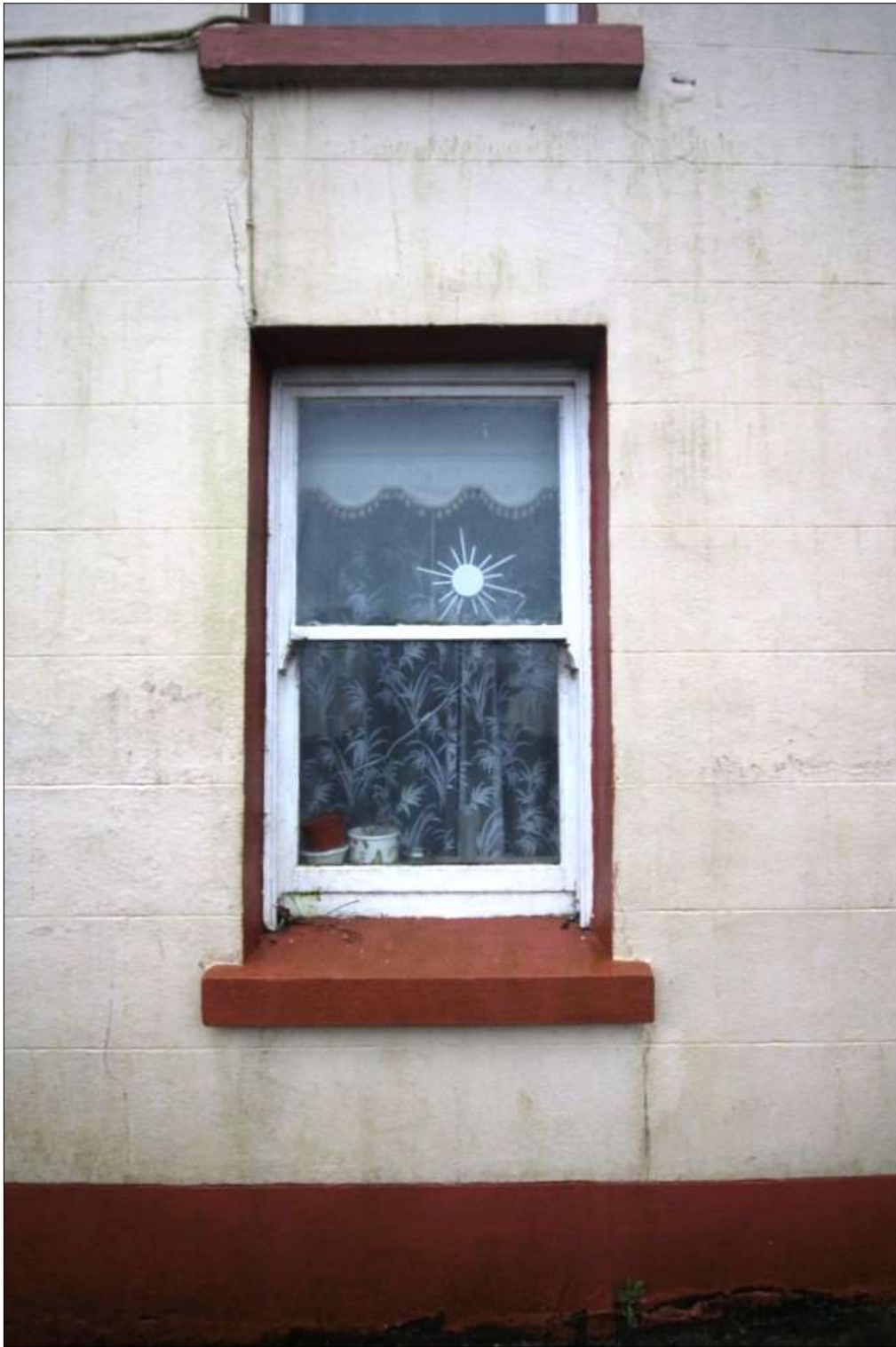
Plate 11: Replacement window detail to front elevation-note sash have been replaced at some time in the last 40 years and are a more square and fresher profile.. Cills are cast concrete
