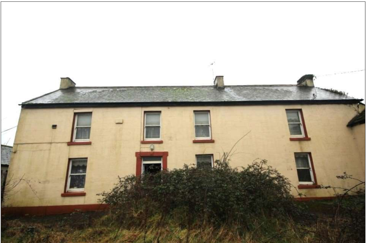
Plate 5: Front (eastern) elevation of Building A-Note window head to lhs first floor window cracked and dislovcated.
