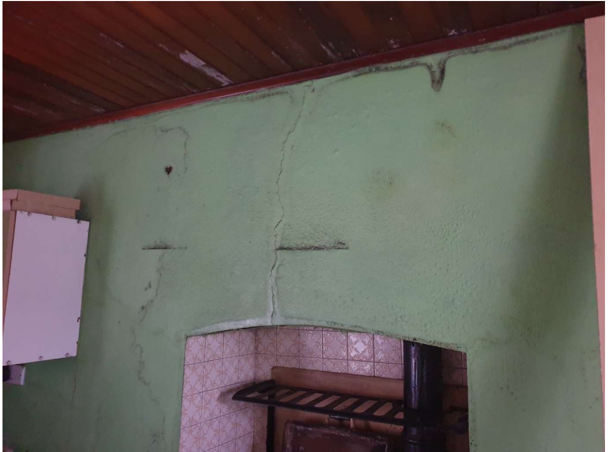
Plate 36: Detail of crack to gable to kitchen.
