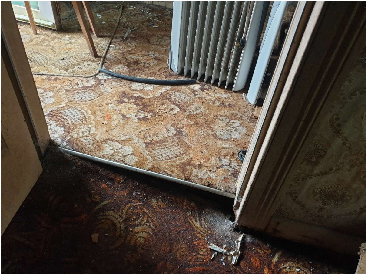
Plate 39: Detail showing collapsed floor to Tv room
