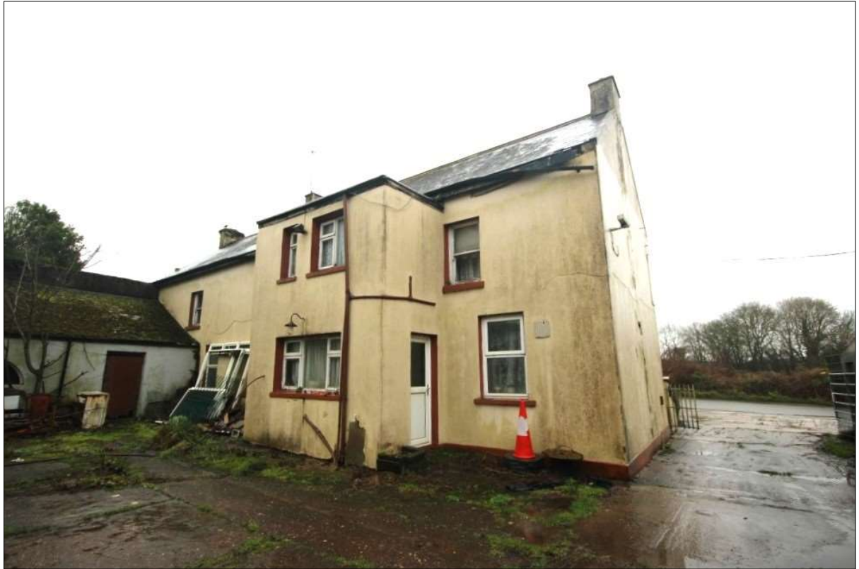
Plate 7: Rear elevation of Building A with later flat-roofed extension-all to be retained in new development -Note gutters and fascias collapsing and modern upvc windows and doors.
