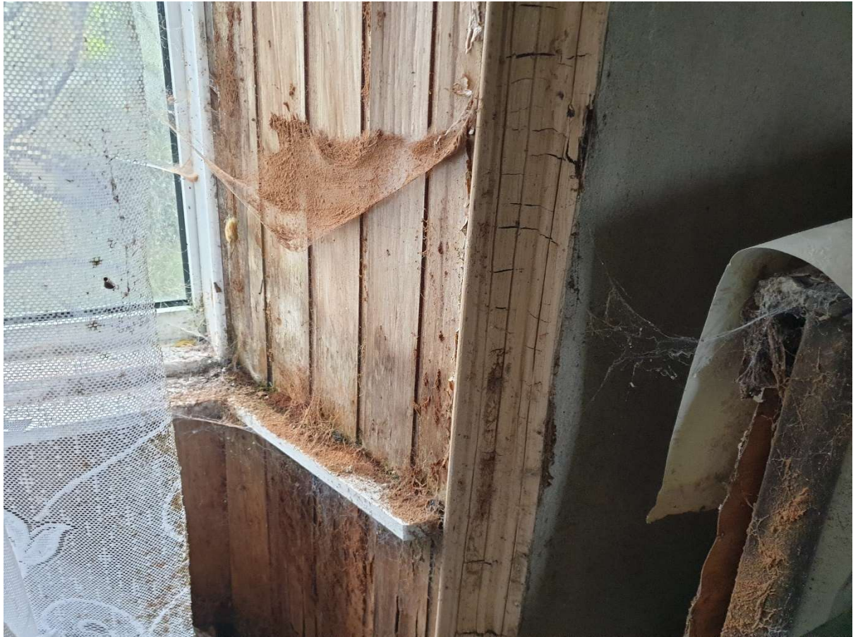
Plate 42: Detail of rotting original timber sheeting to rear window to Living room
