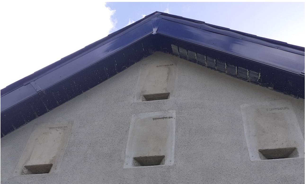
Winter Bat Boxes inserted into wall, post plastering (Oldstreet Substation bat House, Co. Galway).
