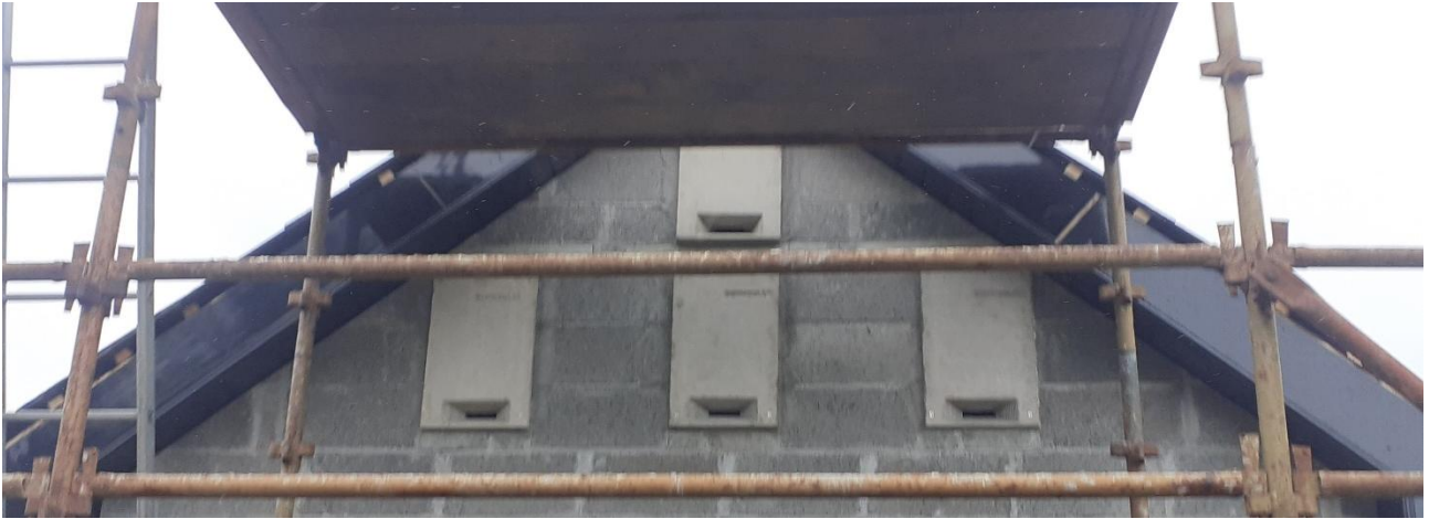
Winter Bat Boxes inserted into wall, prior to plastering (Oldstreet Substation bat House, Co. Galway).
