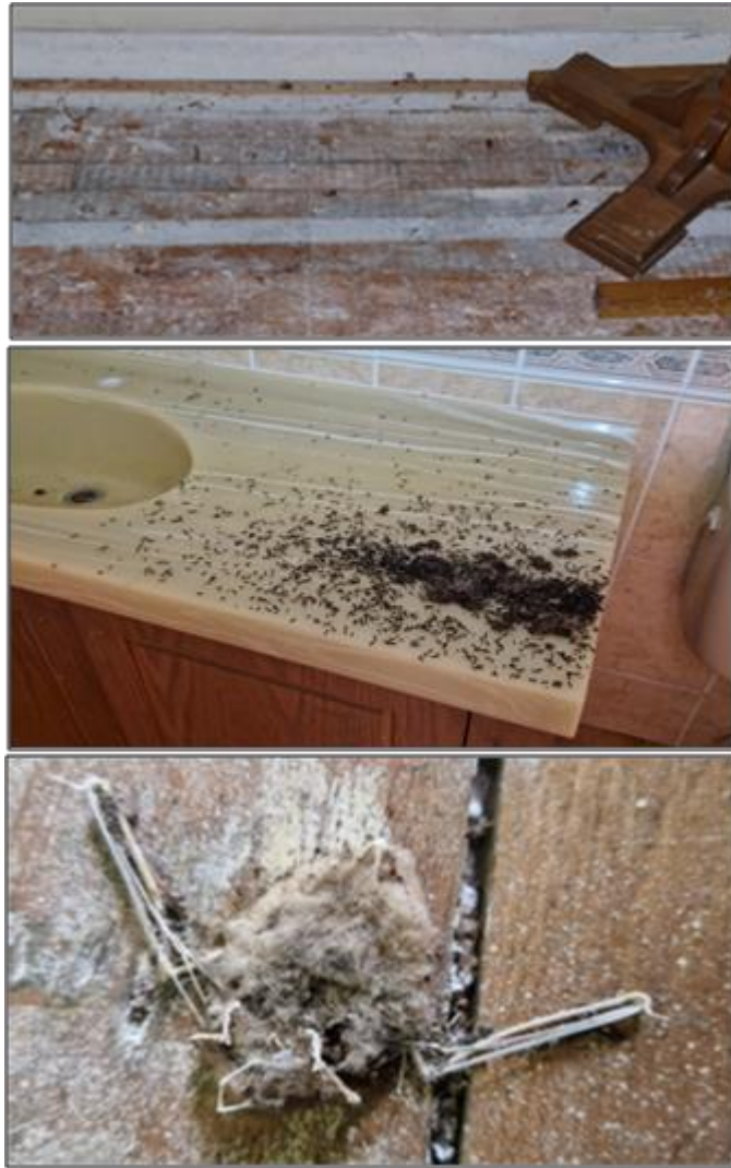
Plate 2 Bat droppings and remains from within two-storey section of hotel.
