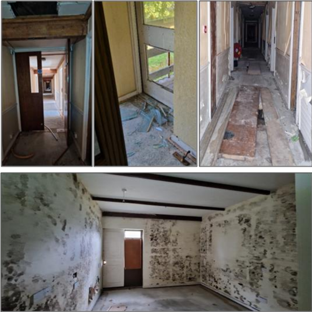
Plate 1 The interior of the two-storey section of the hotel with damage and prevailing damp conditions.
