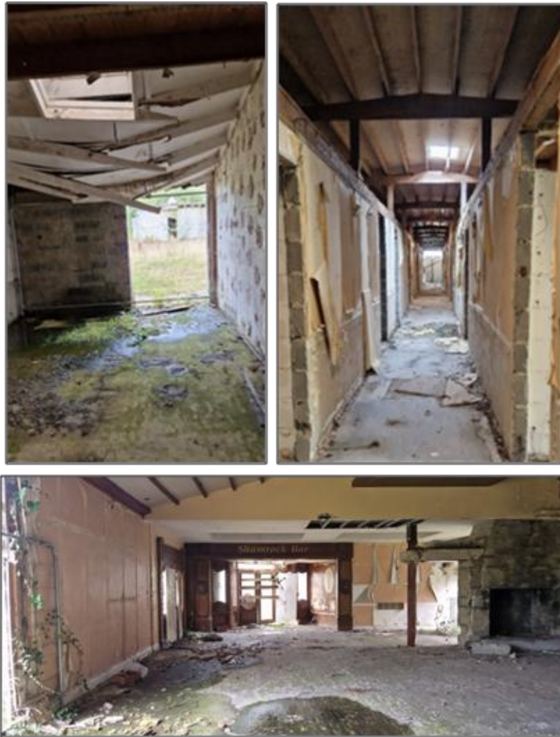
Plate 5 Parts of the single-storey section of the hotel were in very poor condition.
