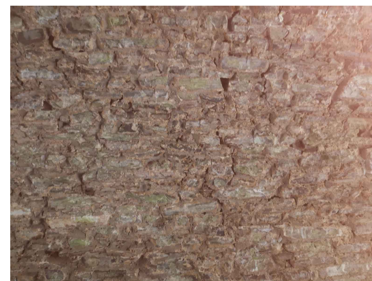
FIGURE 4 ARCH BARREL MINOR CRACKING TO BE REPOINTED
