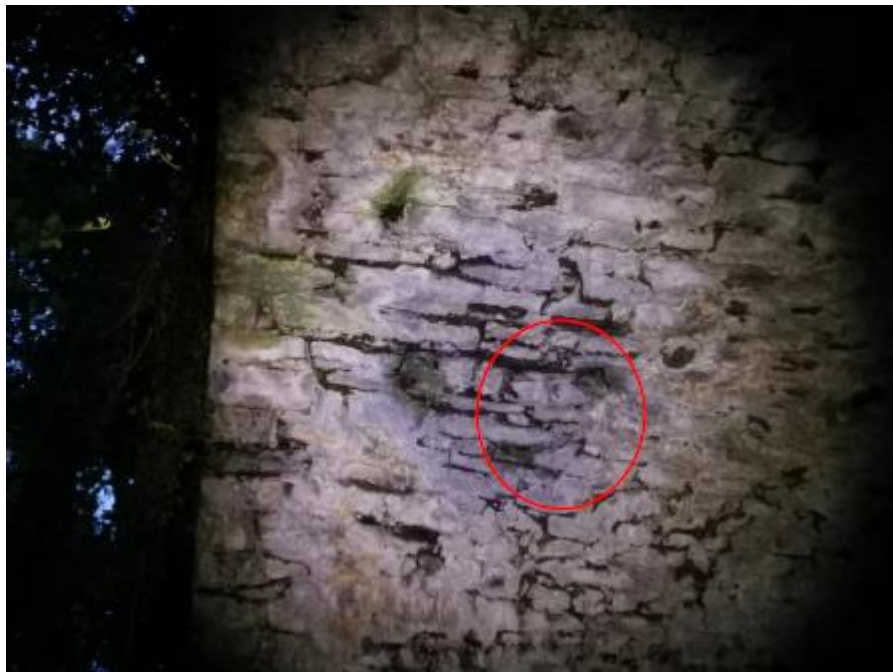
Figure 3.1 Feature on the southern side of the existing Glenmore Bridge where a Daubenton's Bat was observed entering a roost on 13/09/2024.
