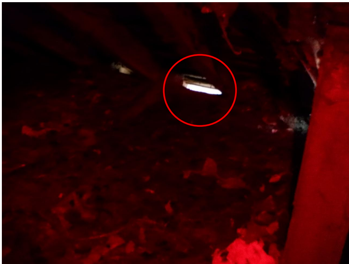
Figure 4-2: Gap under the eaves of the roof providing access to the attic.
