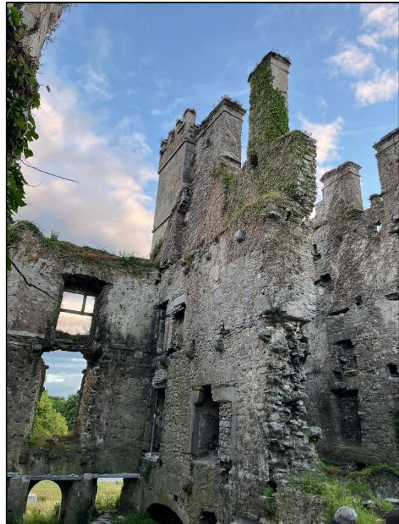
Plate 3 east side of internal wall to be repaired as part of phase 5
