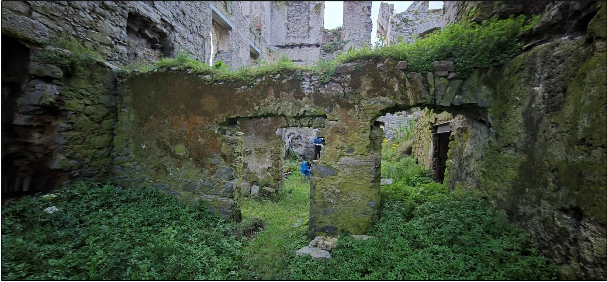
Plate 4: internal walls in the west area of the castle to be repaired as part of phase 6
