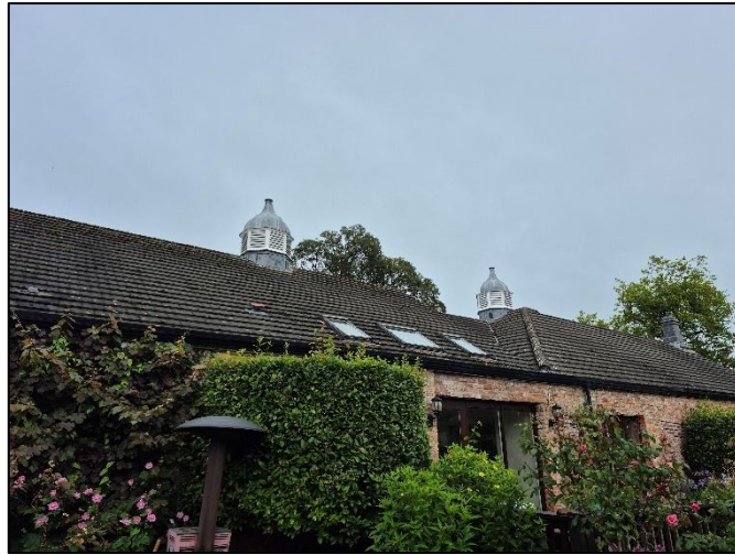
Plate 21: Photo of the roof on the exterior of the Golf Club House.
